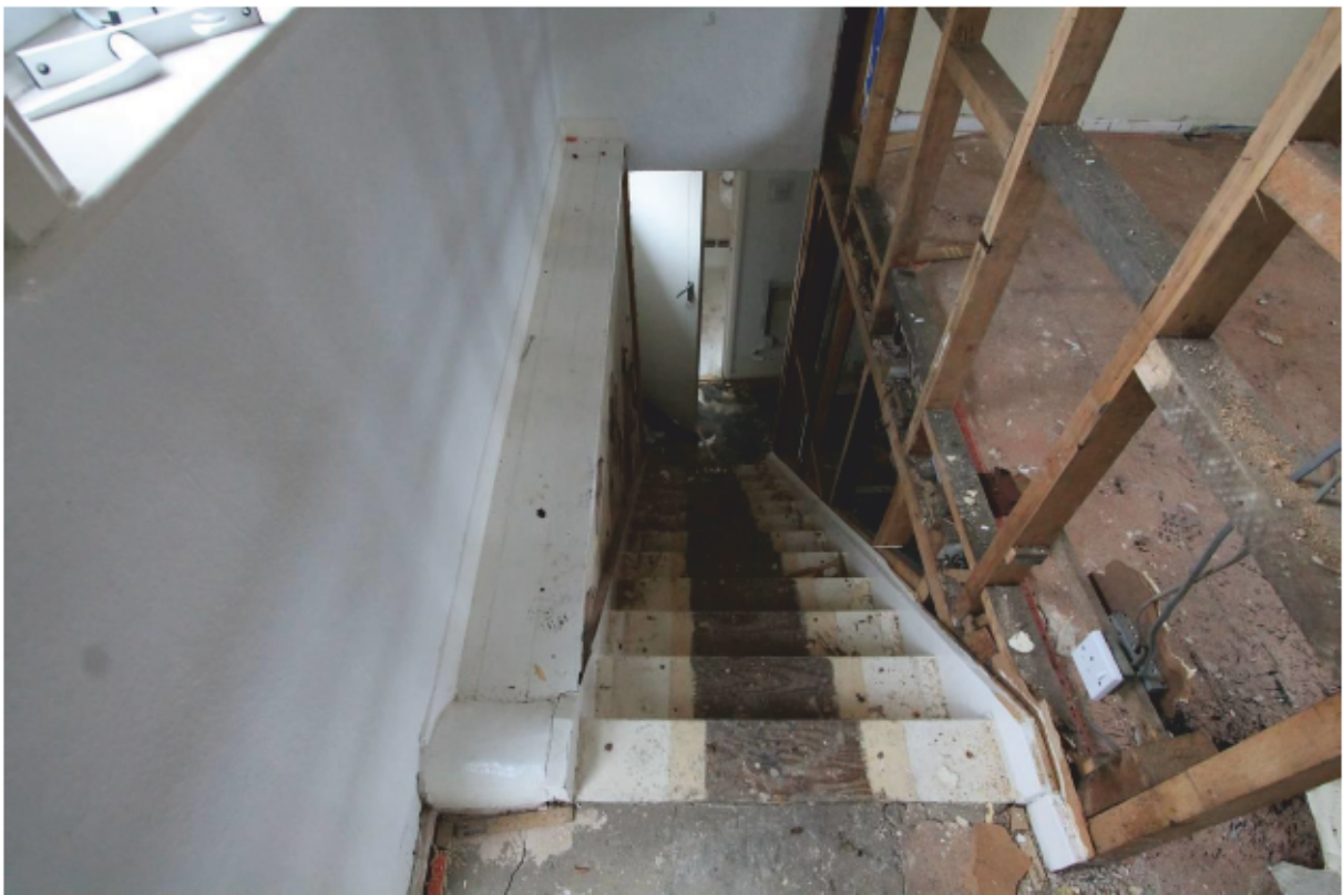
Plate 28 First floor landing showing heavier wall at ground floor level, looking north-west
