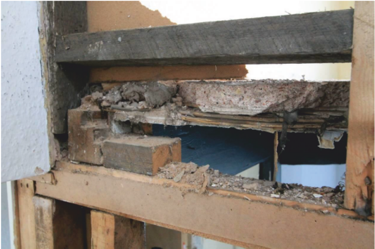
Plate 19 Dovetail lap joint (for trimmer) in end of common joist and lime ash/reed floor, looking north
