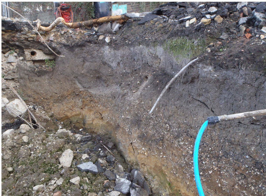
Plate 1. North facing shot of excavations showing recently exposed natural sands and gravels.
