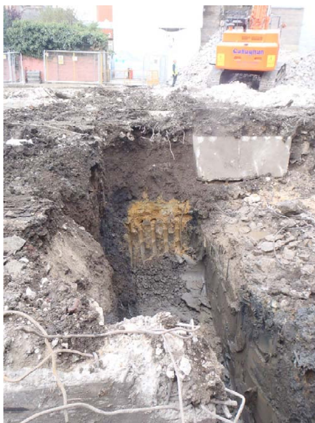
Plate 4. North facing shot in centre of site, shows modern made ground, gravels and London Clay.
