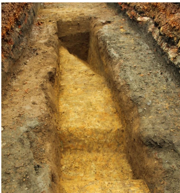
Plate 2: N-S ditch [45] and NW-SE ditch [47] positioned in the background and foreground respectively in Trench 1 and looking NE.
