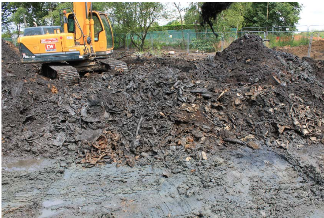
Plate 3: Contaminated made ground in the area of balancing pond, view north
