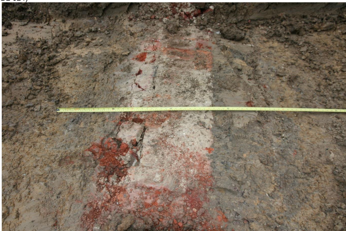
Plate 8: North-south part of wall 19 th century L-shaped brick wall foundation [17] in Trench 6, looking north (BAM16 D2 024)
