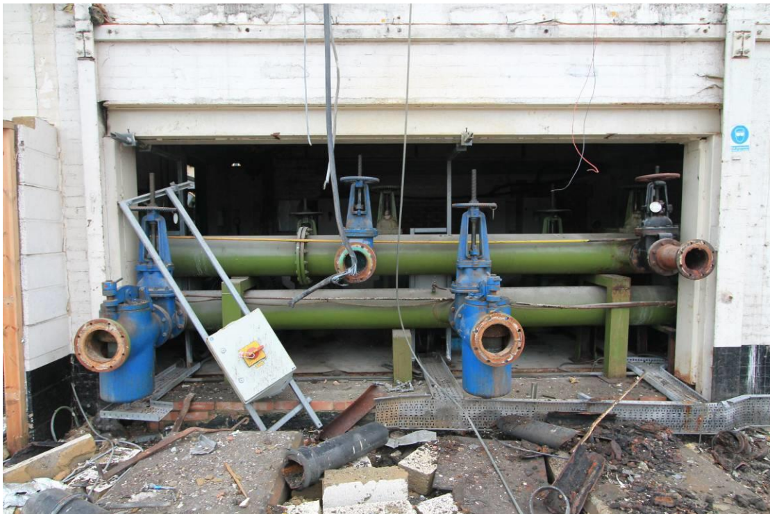
Plate 14 Compression Pipework into adjacent range (north)
