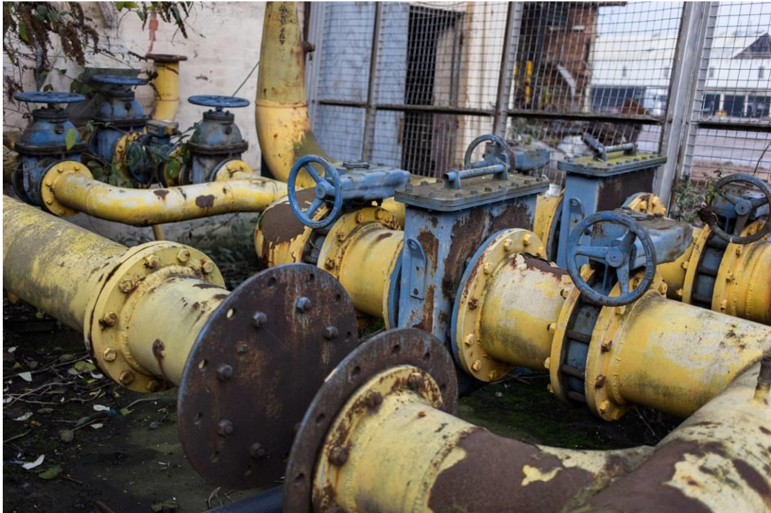
Plate 13 Pipework to east of Power House
