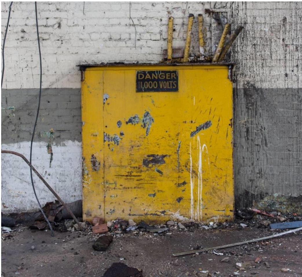
Plate 20 Electrical Outlet/Exchange box
