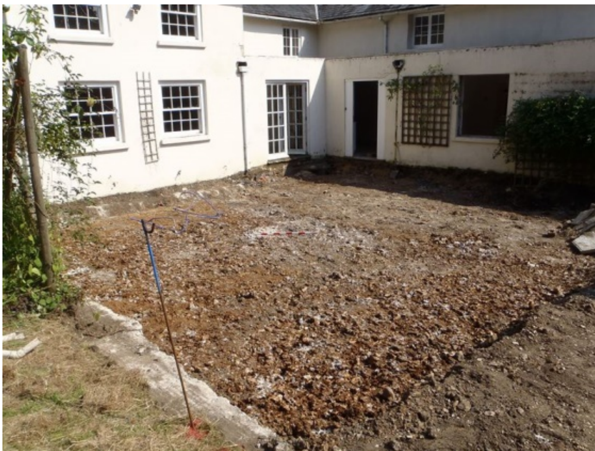
Plate 2: Stripped area for new terrace and extension revealed natural clay-with-flint. View to south-east.
