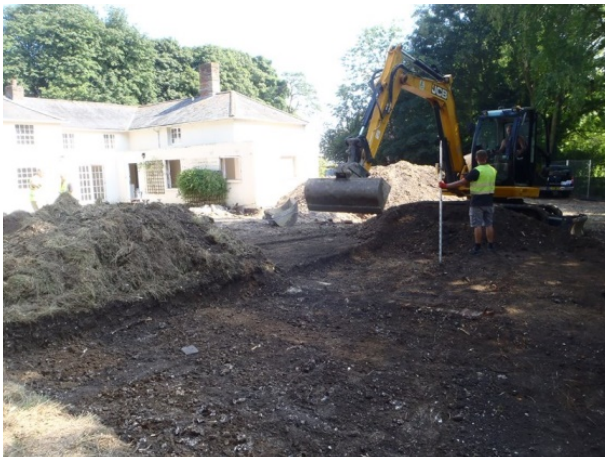
Plate 1: On the western side of the Site, the stripped footprint of the proposed workshop revealed modern made-ground. View to south-east.
