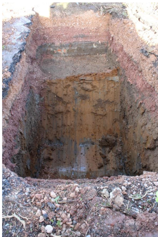
Plate 10: Overview of Trench 12 after excavation of the machine sondage, photograph faces north
