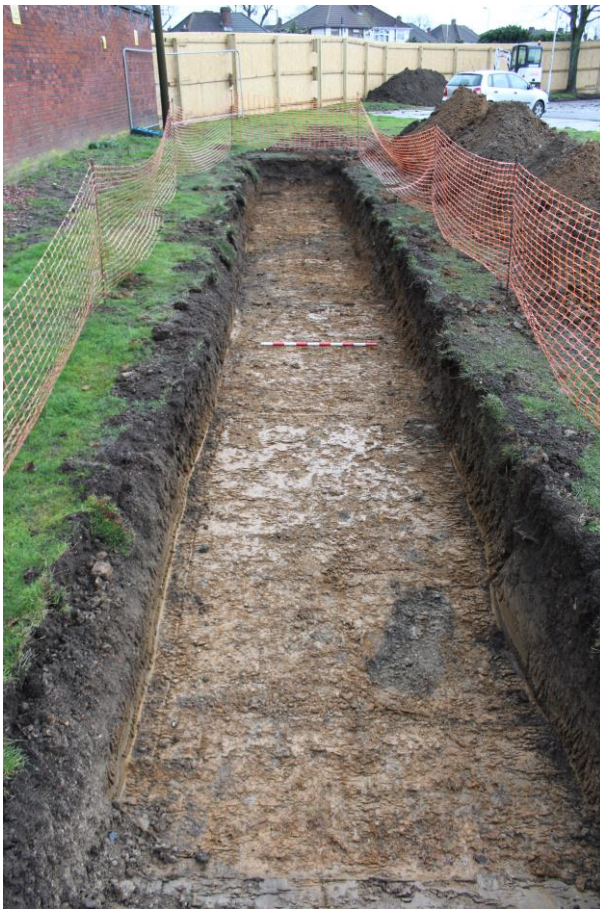
Plate 1: Trench1 facing north. The darker areas represent modern intrusions in all of the plates.
