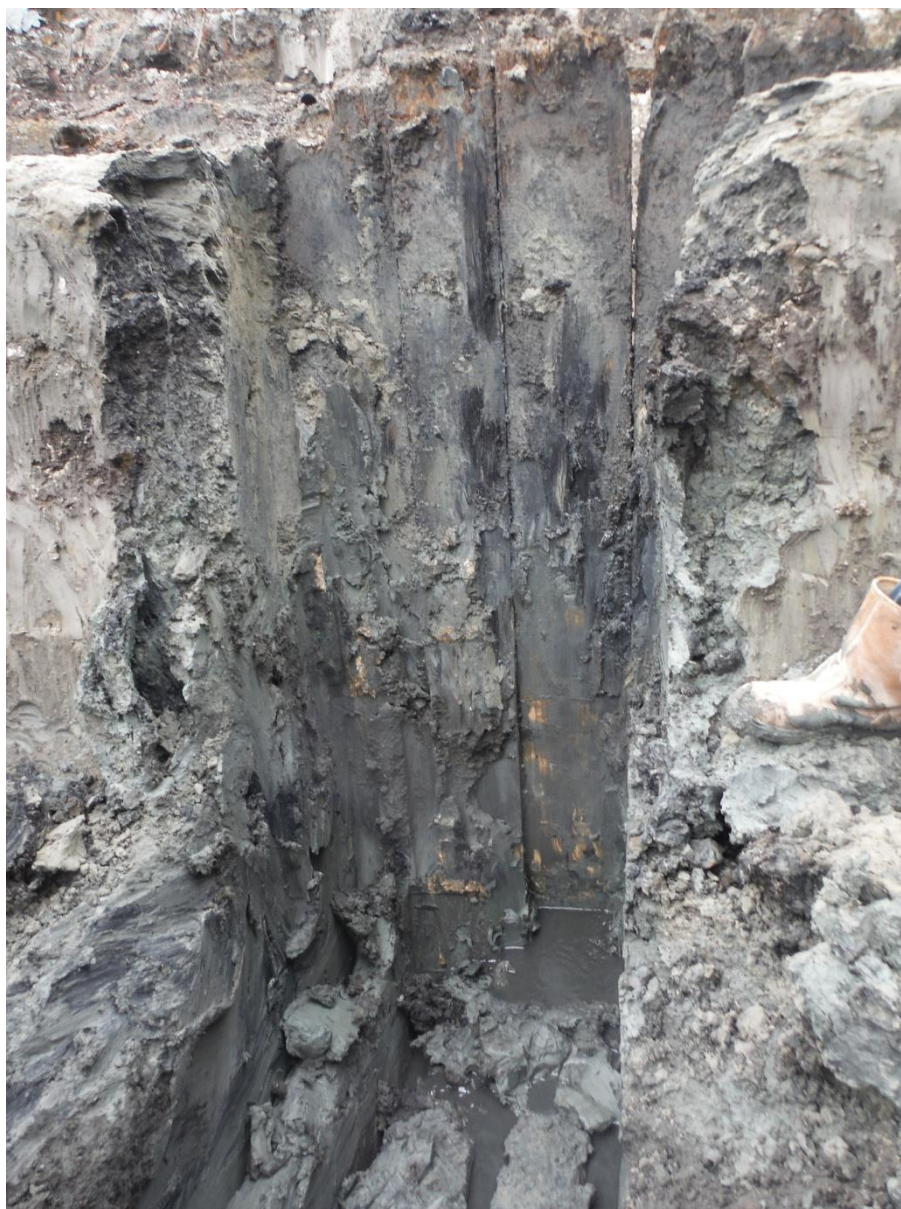
Plate 5: South facing view of sondage on eastern side of canal retaining wall [238] showing extent of timber verticals and water ingress.
