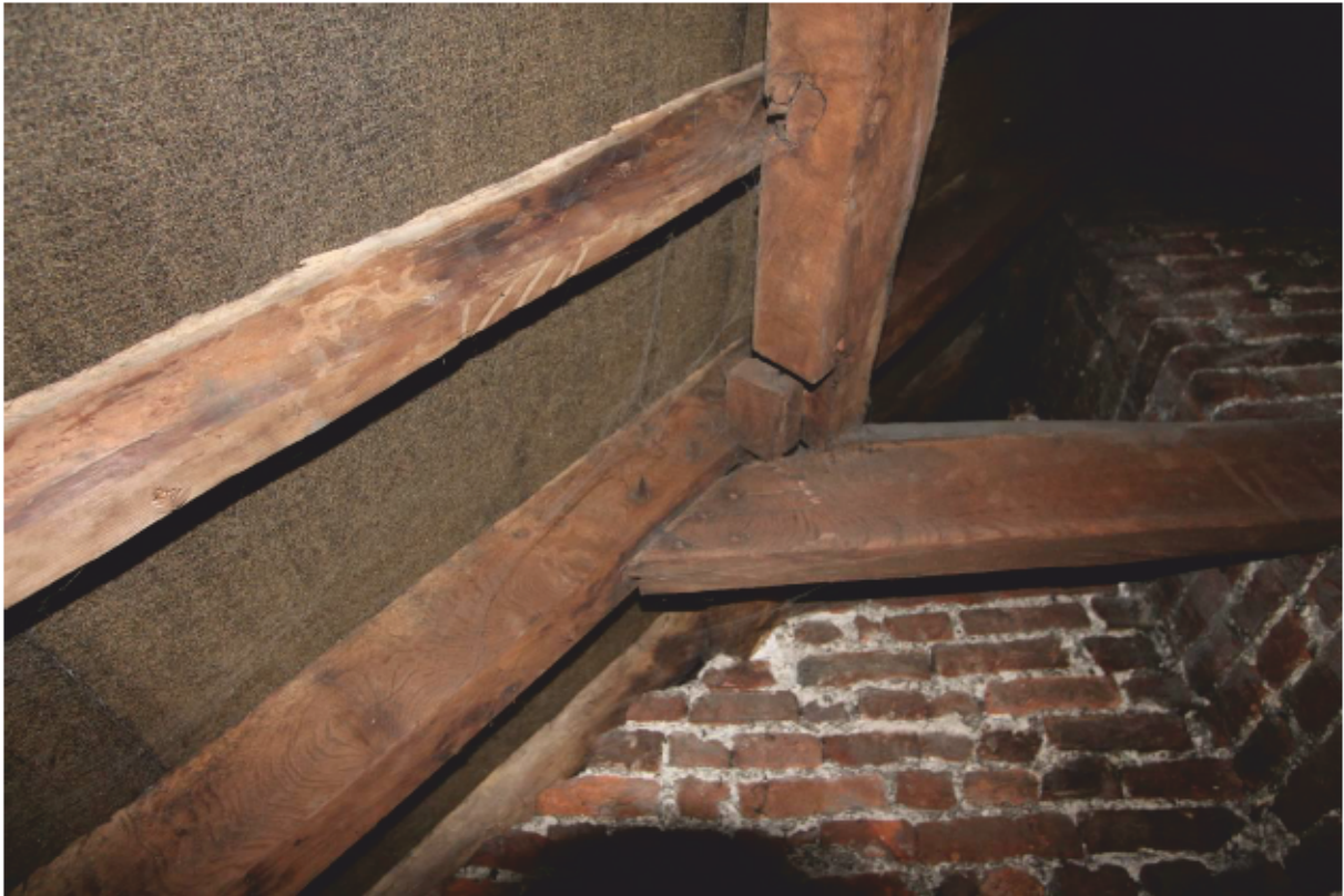
Plate 37 Pegged collar and side purlin
