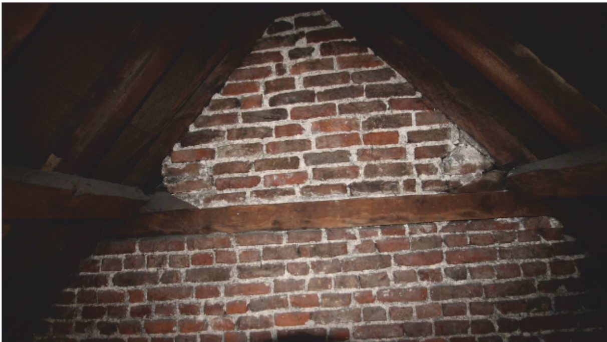
Plate 38 Collar, north cross wall, showing later cleats
