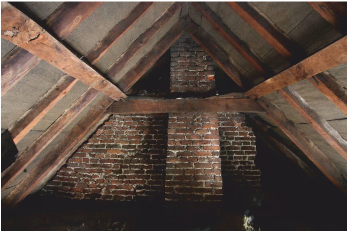
Plate 36 Oak clasped side purlin roof looking south (unit 2) to original stack and cross-wall
