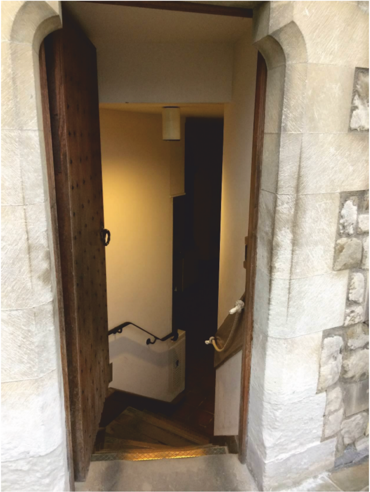
Plate 3 West doorway of the Lanthorn Tower and staircase (before alteration work), looking east (photograph provided by Historic Royal Palaces)
