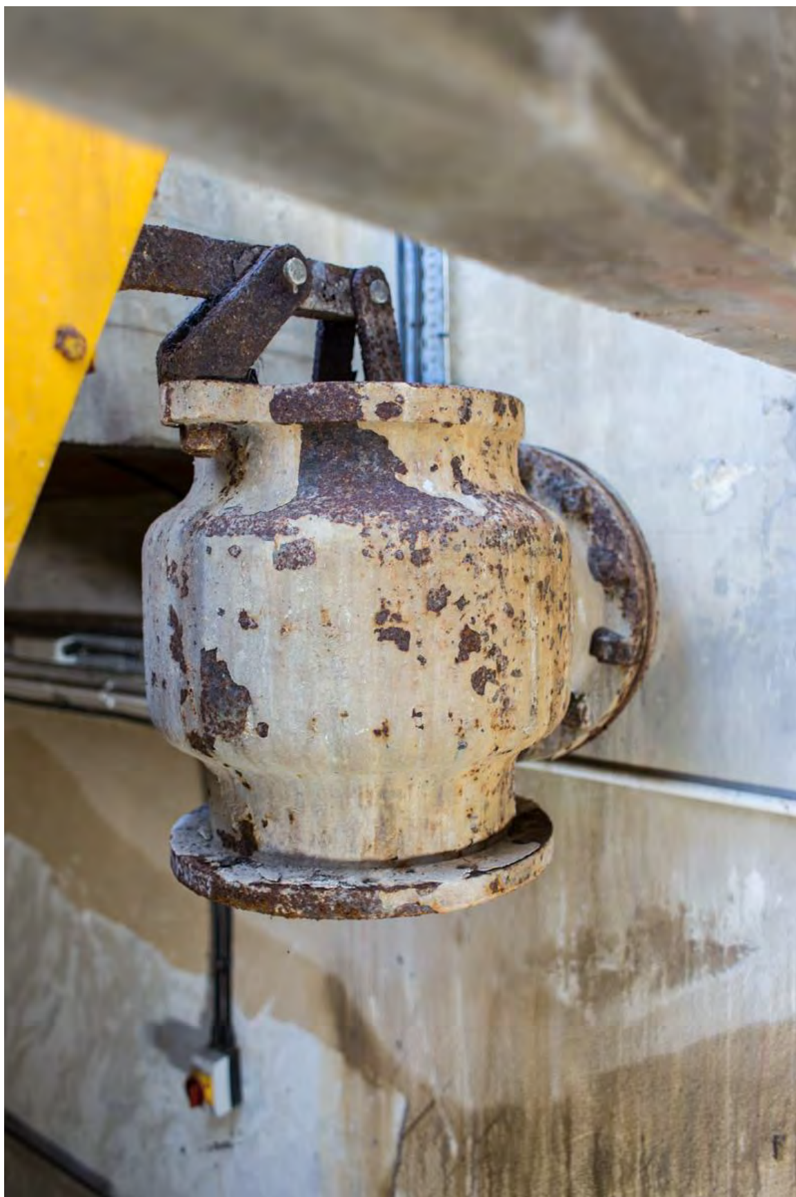
Plate 18 Close up of inlet valve
