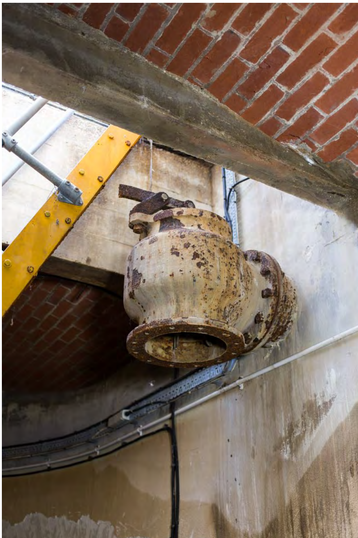
Plate 17 Inlet valve on south-west wall, beneath escape hatch steps
