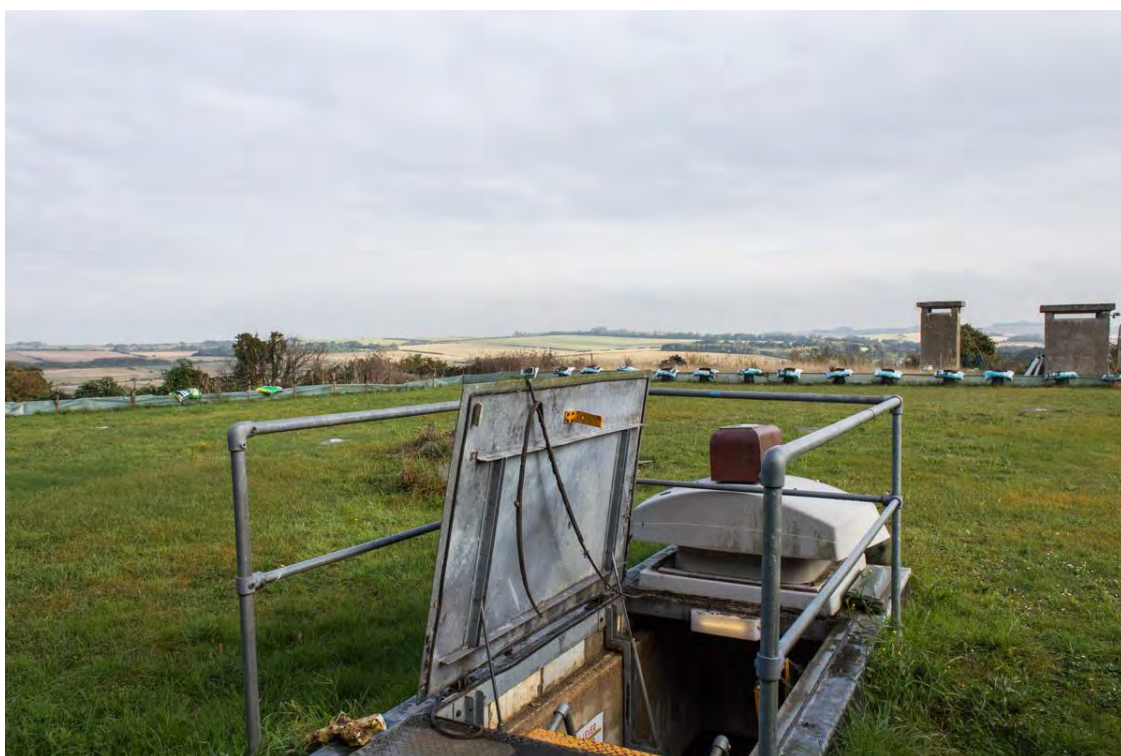
Plate 2 View to the north of roof of reservoir (escape hatch in foreground and bunker ventilation shafts in background)
