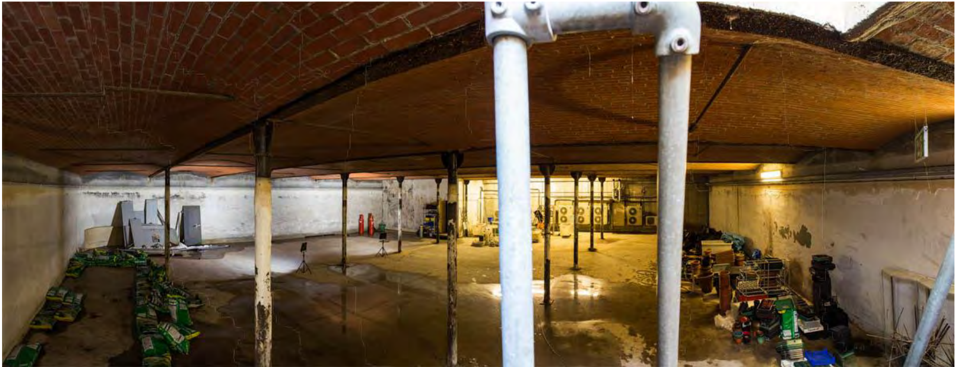
Plate 4 View to the north from reservoir entrance (escape hatch), of internal reservoir space
