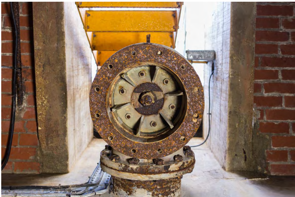
Plate 19 View from beneath of inlet valve
