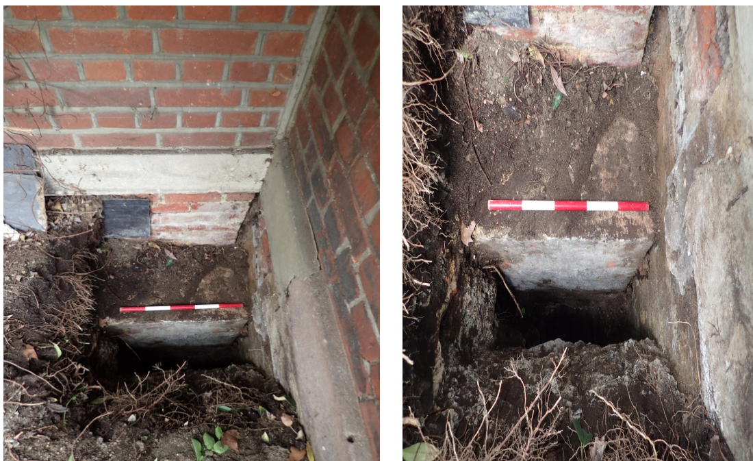
Plate 2a & 2b: Test Pit 2, view to the north (scale 0.5m). Plate 2a clearly shows the expansion gap between the buildings and the modern concrete footing [6]. Plate 2b shows the concrete layer [14] to the bottom of the picture which had to be broken out to create access to the base of the footings [6].
