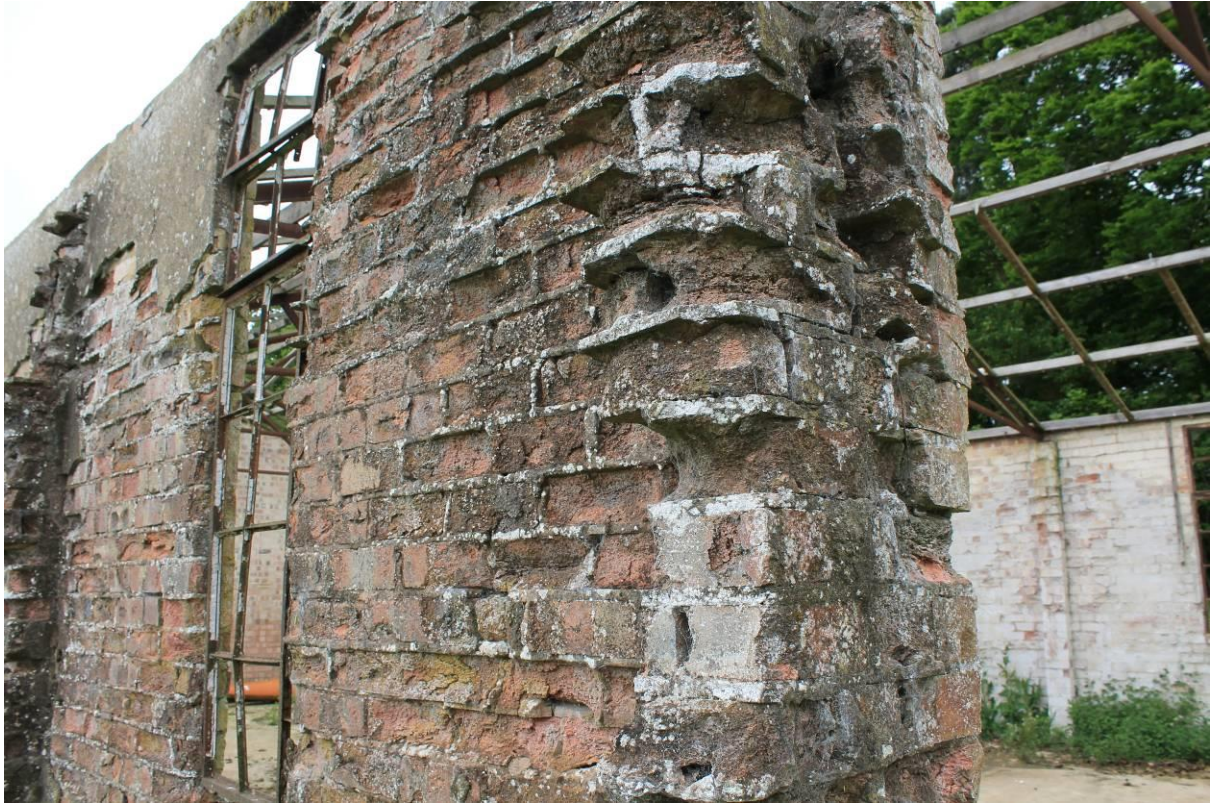
Plate 7 Detail of spalled brickwork
