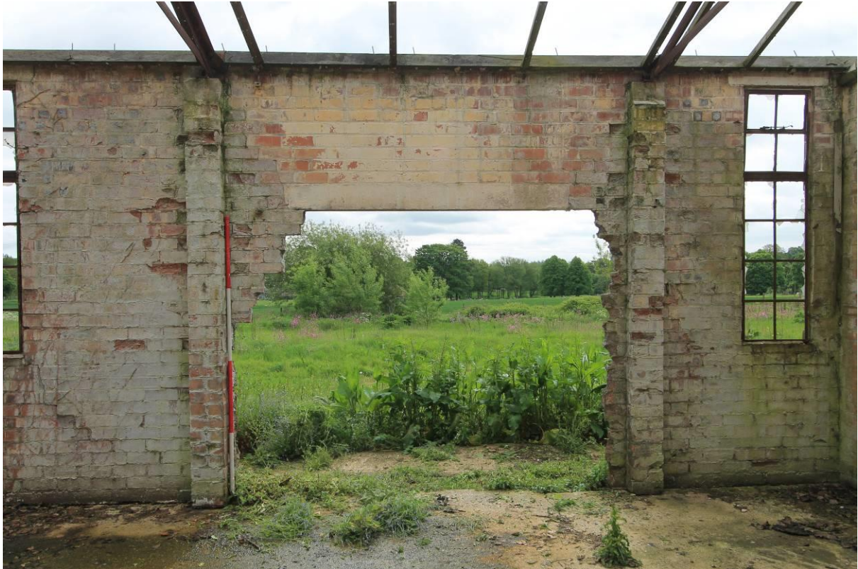
Plate 14 Original opening (part collapsed) to bay 3
