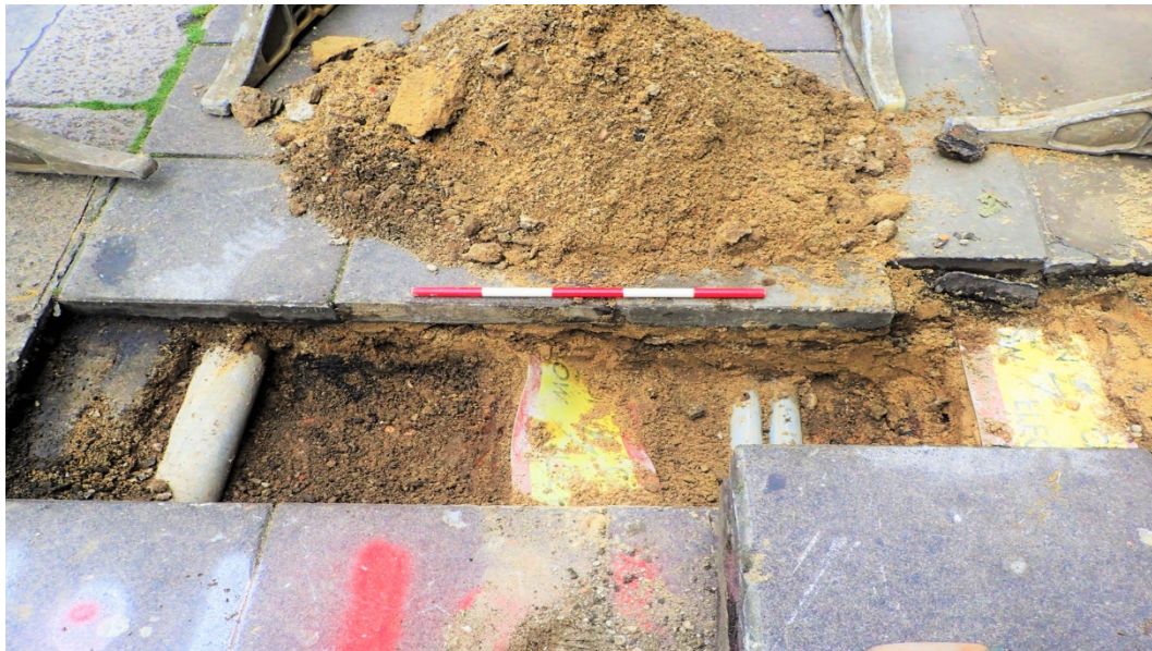
Plate 2: TH1:B1 view to north-west with roadside kerb to the left of the photograph. Multiple services were revealed directly below the paving slabs. Layer [9] was service trench backfill. Scale 0.5m.
