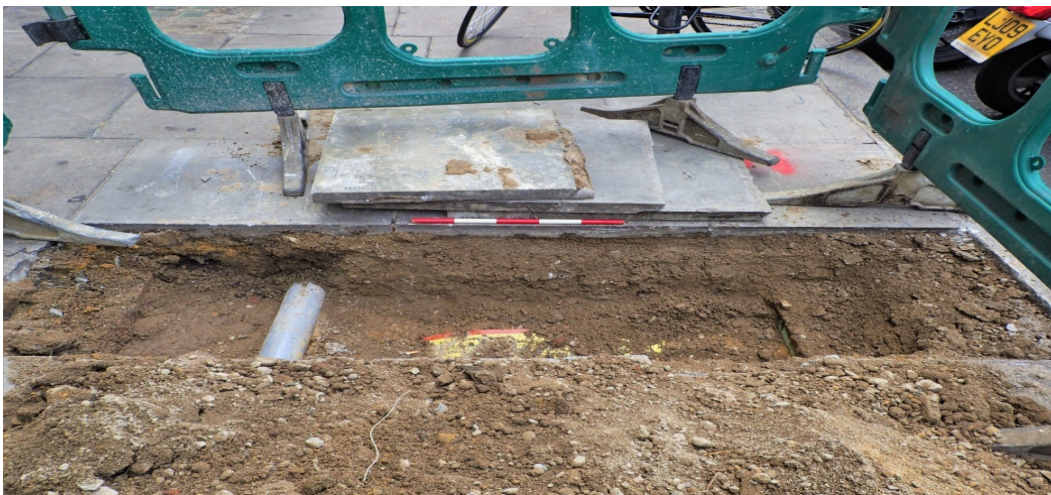
Plate 7: TH4:B4 view to the south-east, roadside kerb on the right of the picture. Services and made ground [4]. Scale 0.5m.
