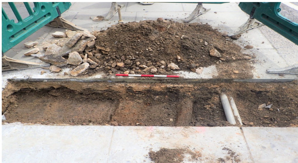
Plate 5: TH2:B2 view to the north-east, roadside kerb on the right of picture. A series of services prevented further excavation. Scale 0.5m
