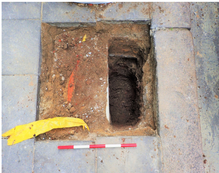
Plate 3: TH02 view to the south-east, roadside kerb on the right of the photograph. Services prevented the hole being excavated to its full size so a sondage was created on the western edge. Scale 0.5m.
