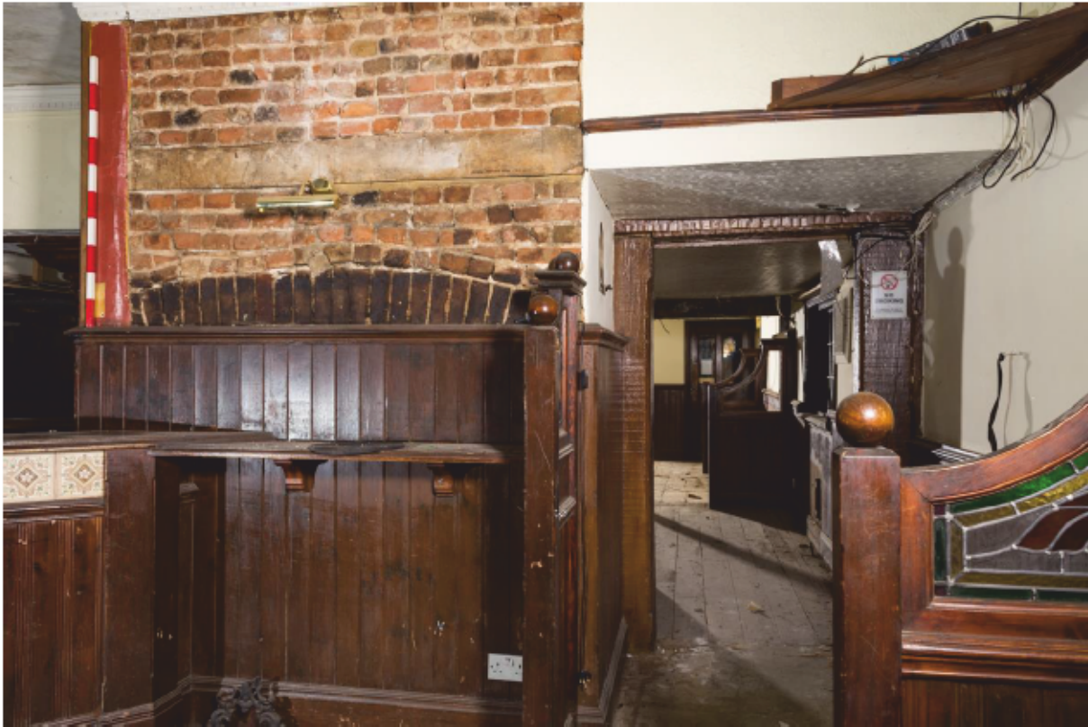
Plate 23 Blocked fireplace in GF6
