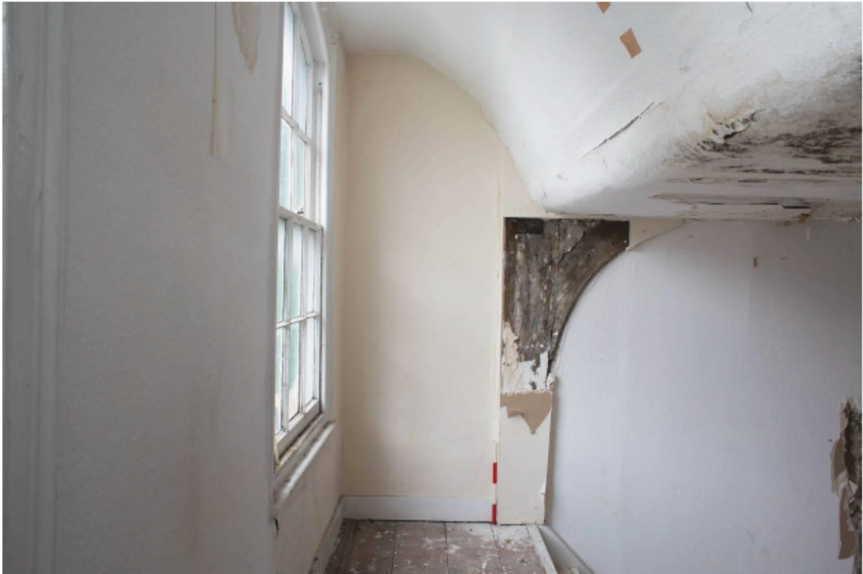
Plate 31 Curved arch brace and storey post, plus later refronting and window heightening (FF2)
