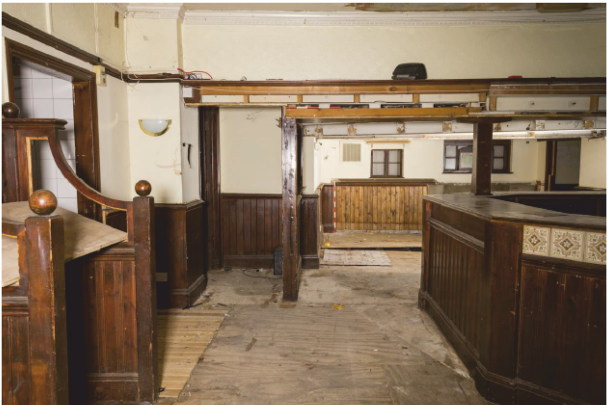
Plate 16 Bar, from GF6 to GF5
