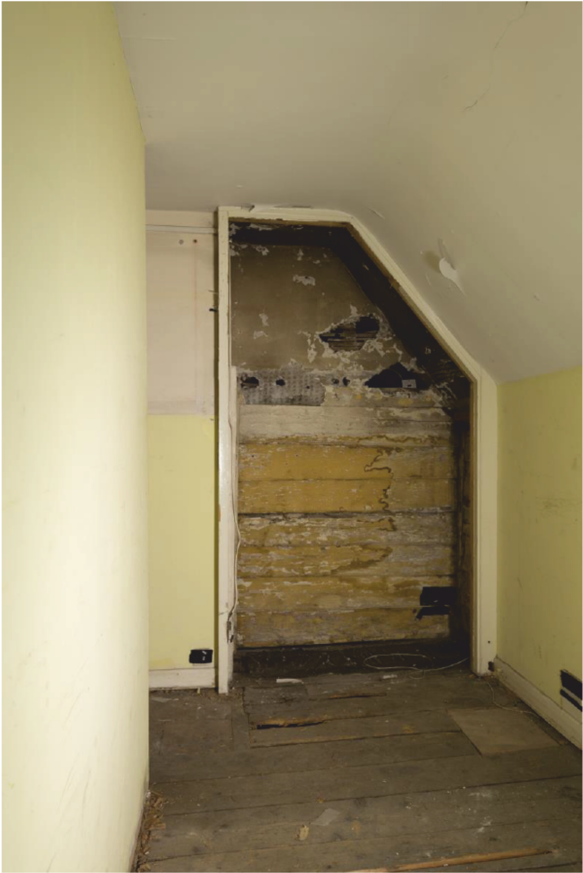
Plate 39 Trapped weatherboard in alcove (FF7)
