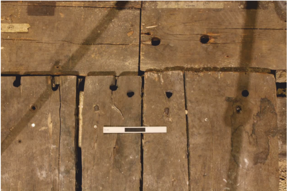
Plate 13 Bay IV Floorboards (49 and 50) west, detail of historic nails and drilled holes (0.15m scale)
