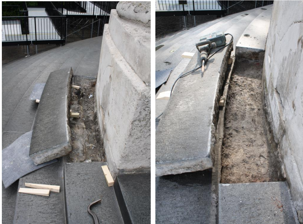
Plates 3 and 4: Test Pit 2, before and after the removal of the bedding, facing east.
