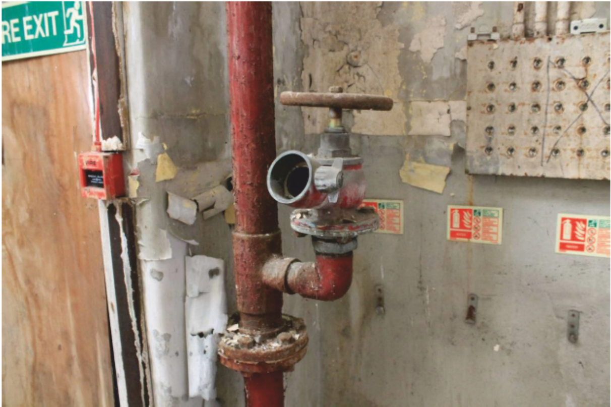
Plate 34 Fire hydrant at ground floor
