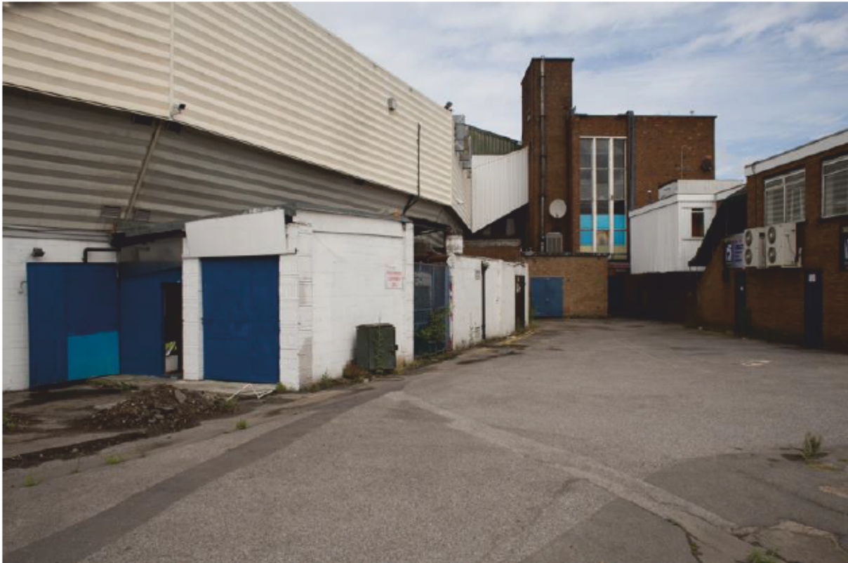
Plate 15 Rear of stand to south-east, looking north towards Main Grandstand stair bay
