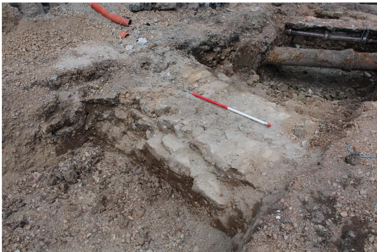
Plate 5, Photo of the Portwall (1166) within the district heating main trench looking northwest.
