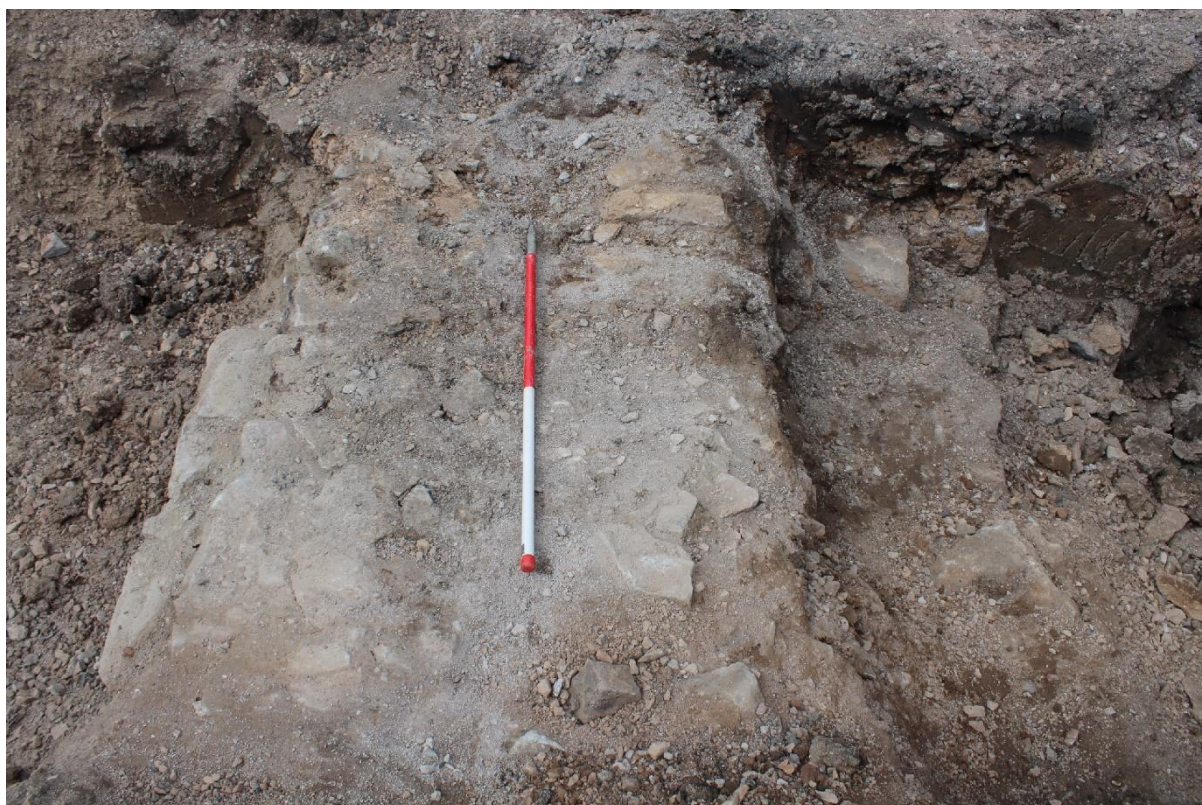
Plate 4, Photo of the Portwall (1166) within the district heating main trench, looking west
