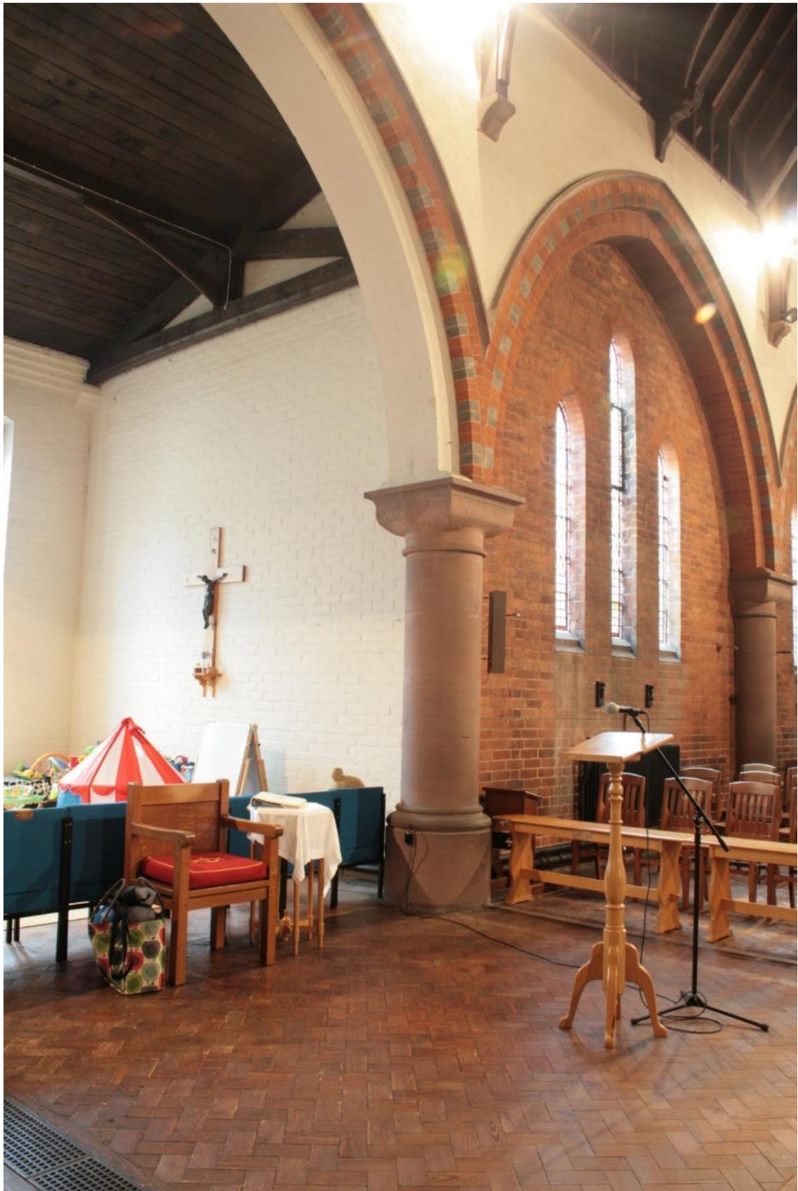
Plate 54: Circa 1936 partial south aisle (left) and south wall (right) of St George's Church, looking south-west
