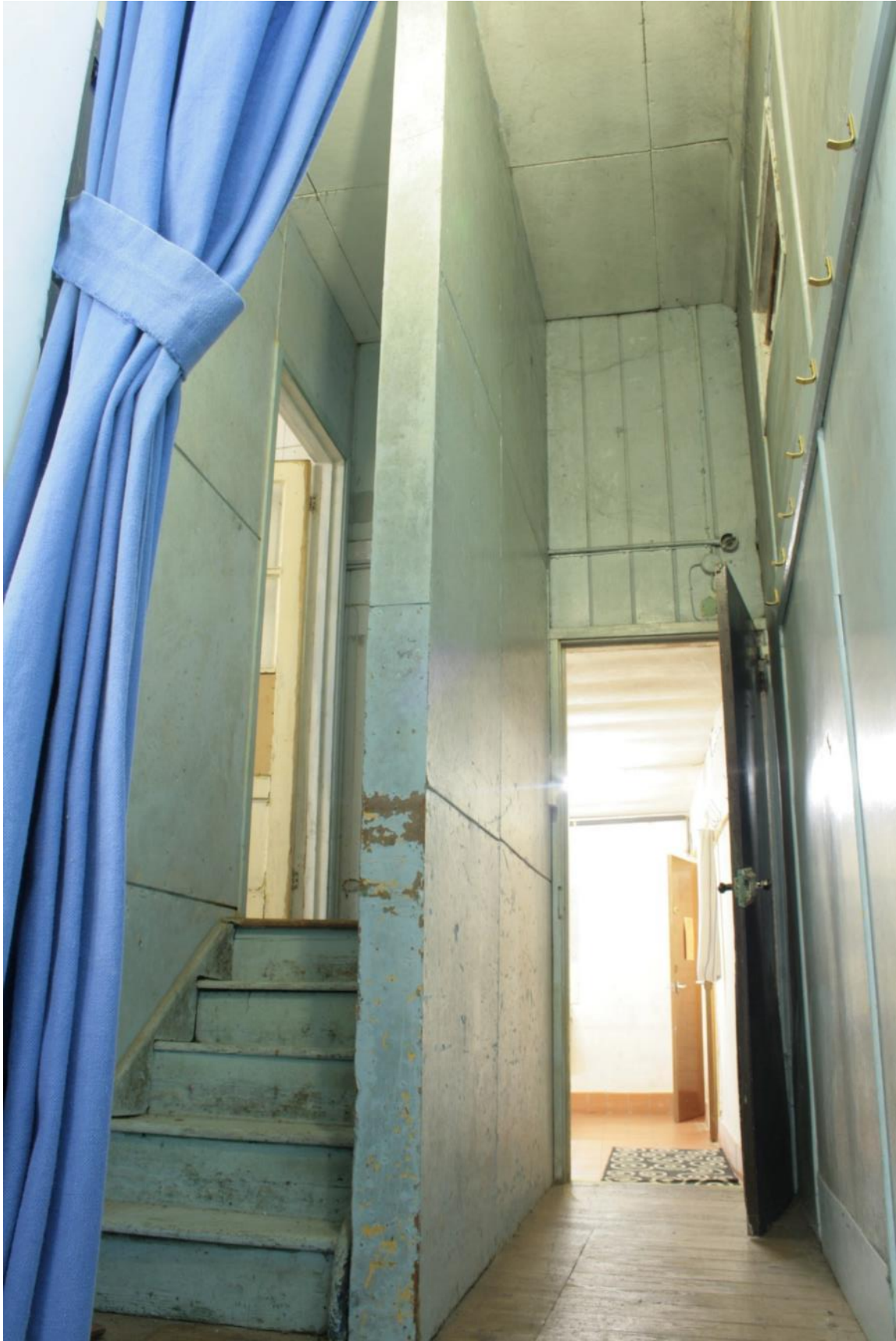
Plate 34: Entrance stairs to stage (left) and toilet entrance (right) on south side of St George's Hall, looking east
