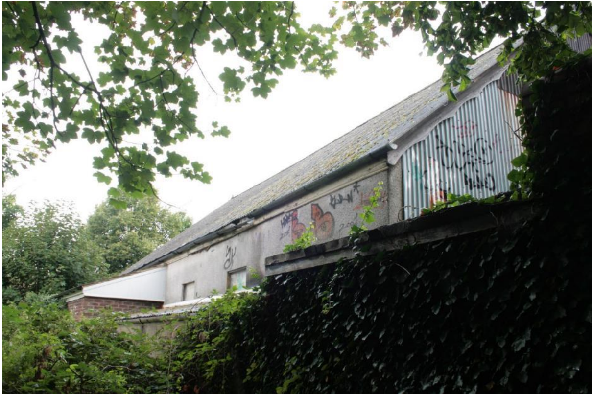
Plate 11: South (rear side) elevation and brick extension of St George's Hall, looking north-west
