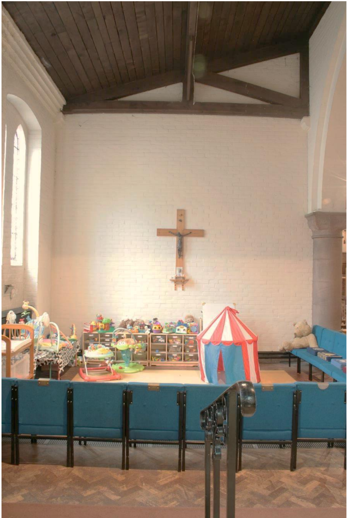
Plate 55: West wall of c.1936 partial south aisle extension in St George's Church, looking west
