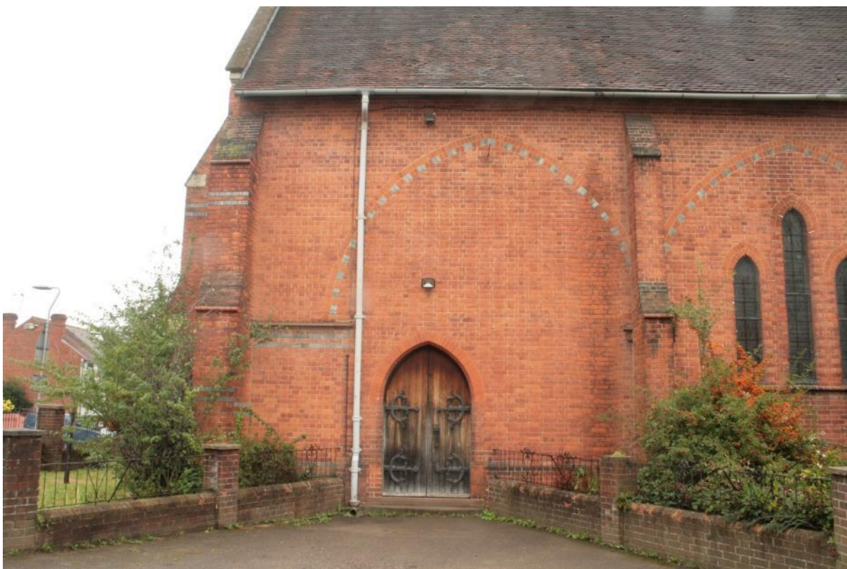
Plate 49: West end of the south elevation of St George's Church, looking north
