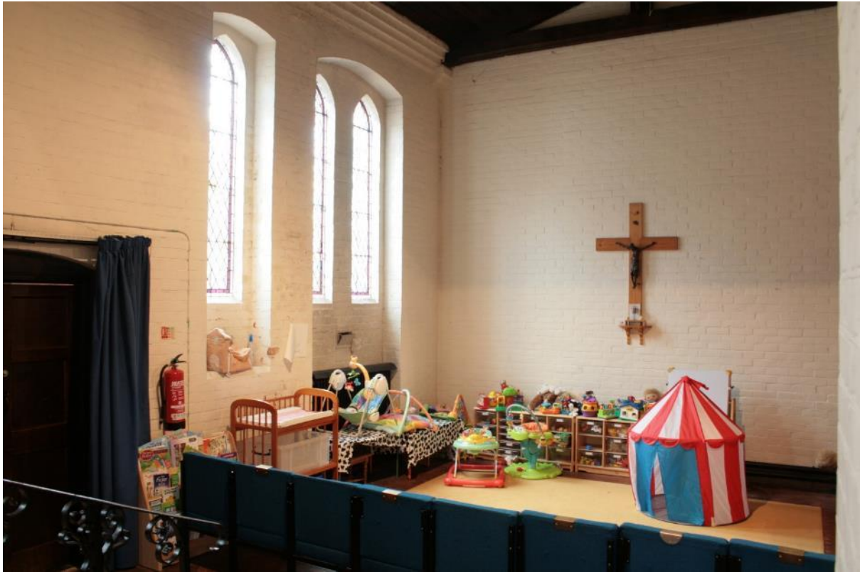
Plate 56: South-west corner of c.1936 partial south aisle extension in St George's Church, looking south-west
