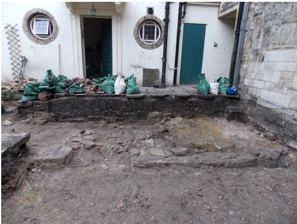
Plate 4: West facing view of ground reduction area within the Receiver General's garden
