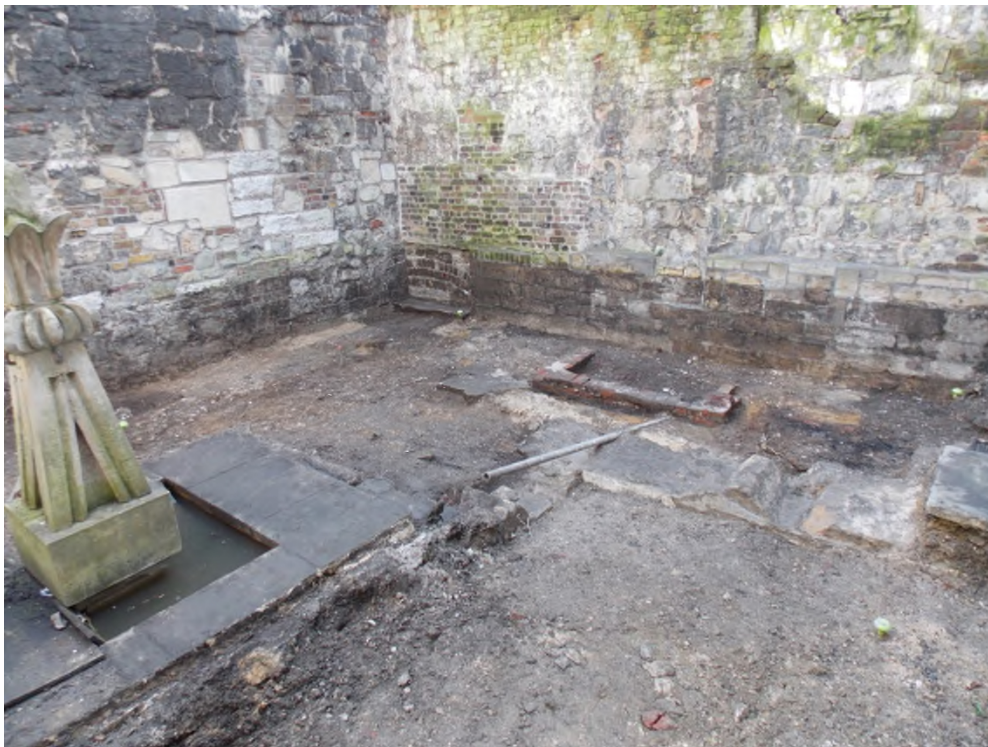
Plate 2: South-east facing view of ground reduction area within the Receiver General's garden
