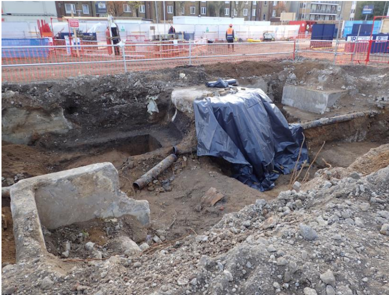
Plate 25 Southern end of trench with Area A on the top left and Area B on the top right. Asbestos was found in the shuttering for the concrete foundation between the two areas, hence the blue plastic cover
