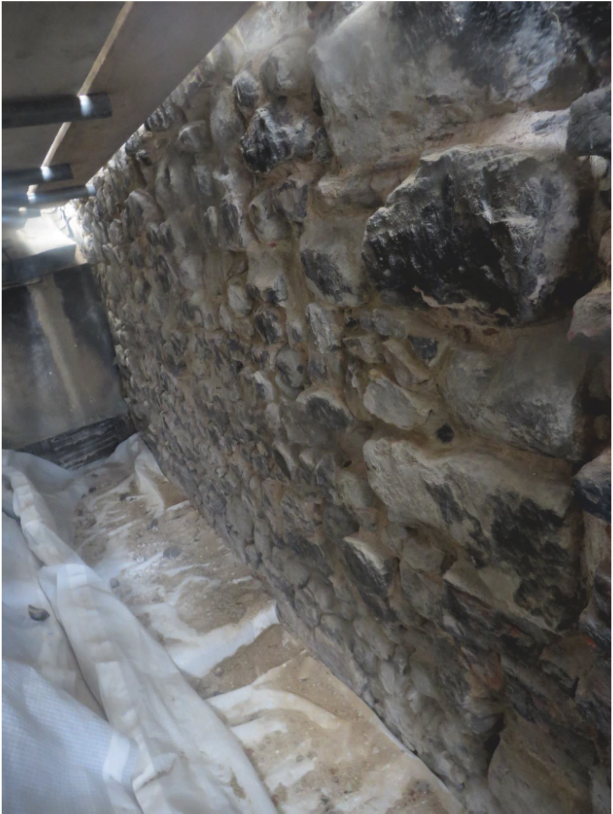
Plate 11: Lower part of the east gable wall of the Queen's House from the lower scaffold level, looking south-west
