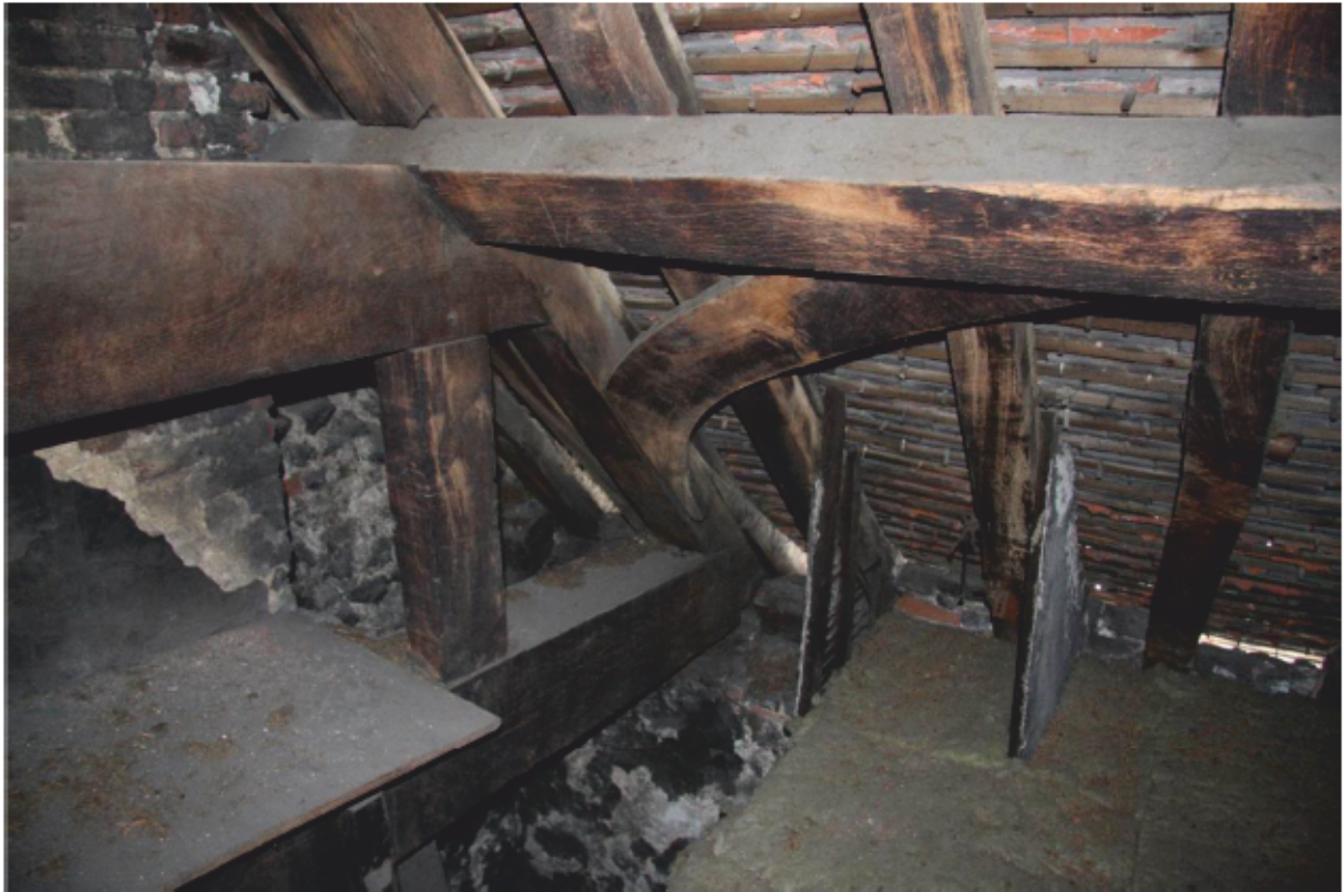
Plate 21: The east gable end wall of the Queen's House Kitchen (left), looking south-east from the roof space (photograph provided by HRP)
