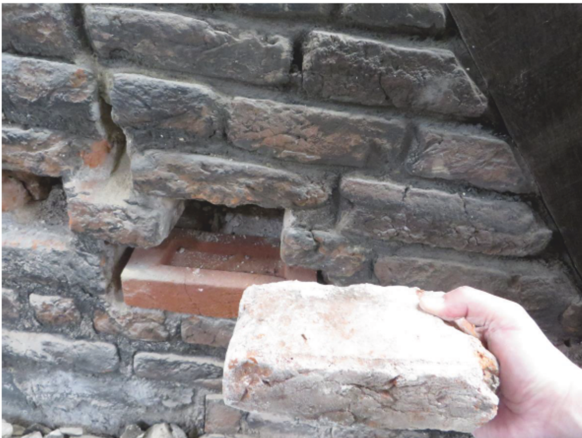
Plate 6: Brick from the north side of the east gable wall of the Queen's House, looking west
