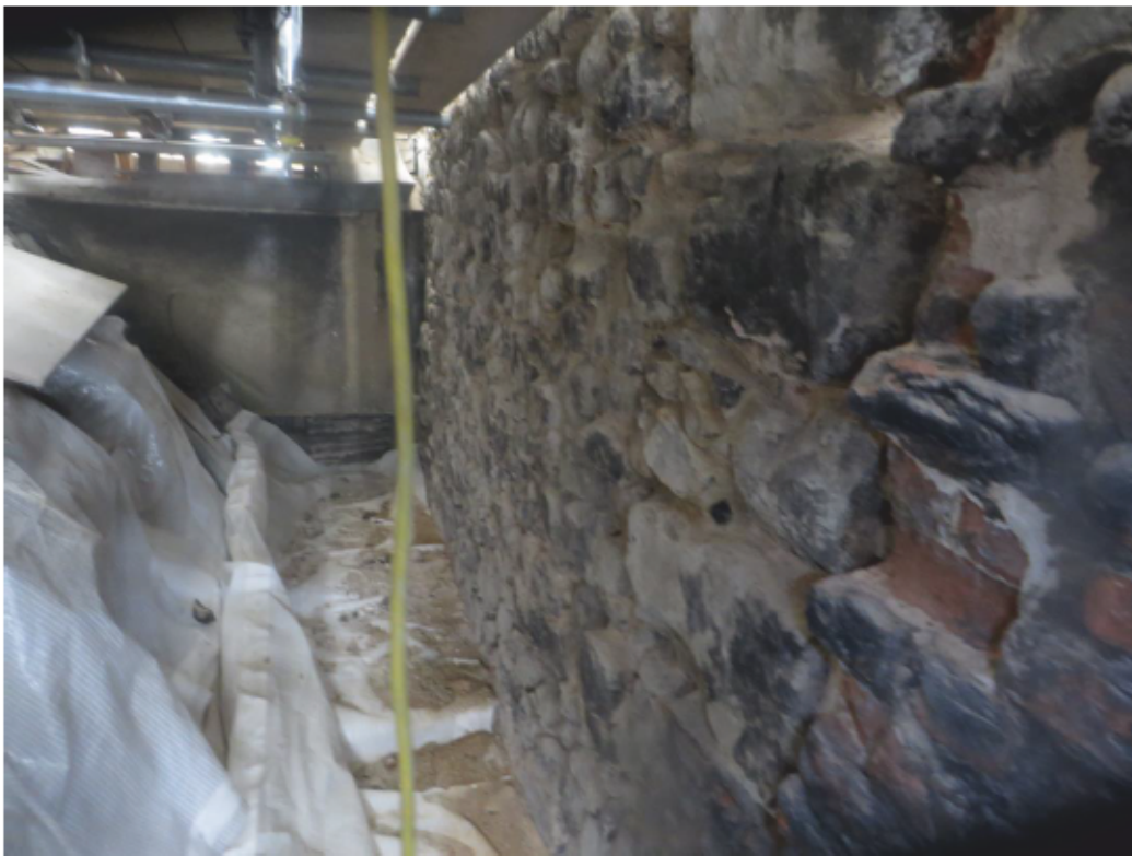
Plate 10: Lower part of the east gable wall of the Queen's House from the lower scaffold level, looking south
