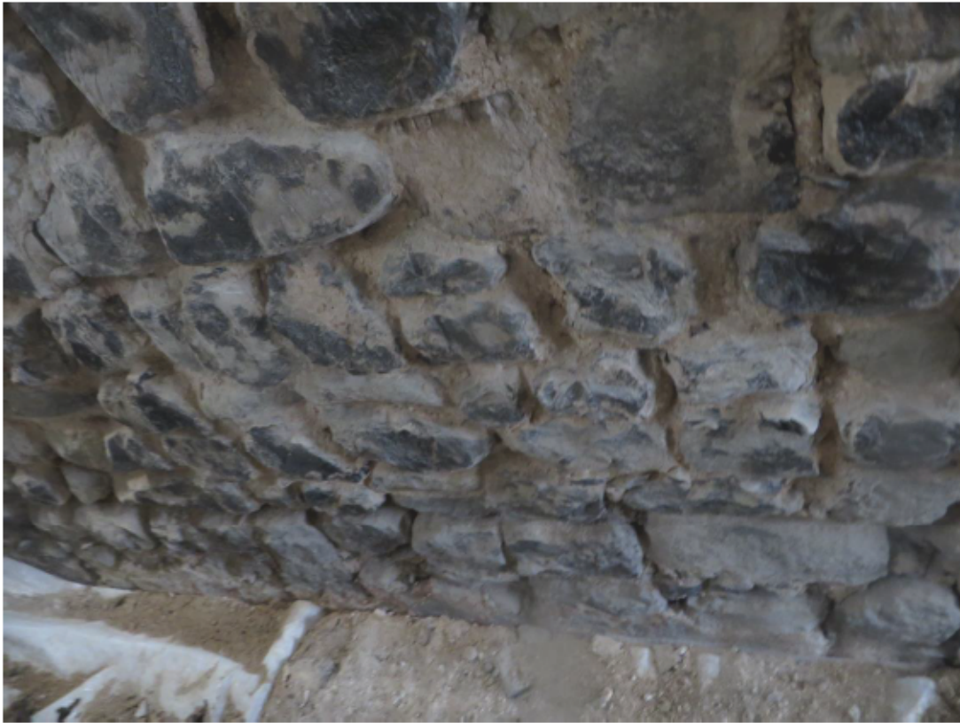
Plate 9: Lower part of the east gable wall of the Queen's House from the lower scaffold level, looking west
