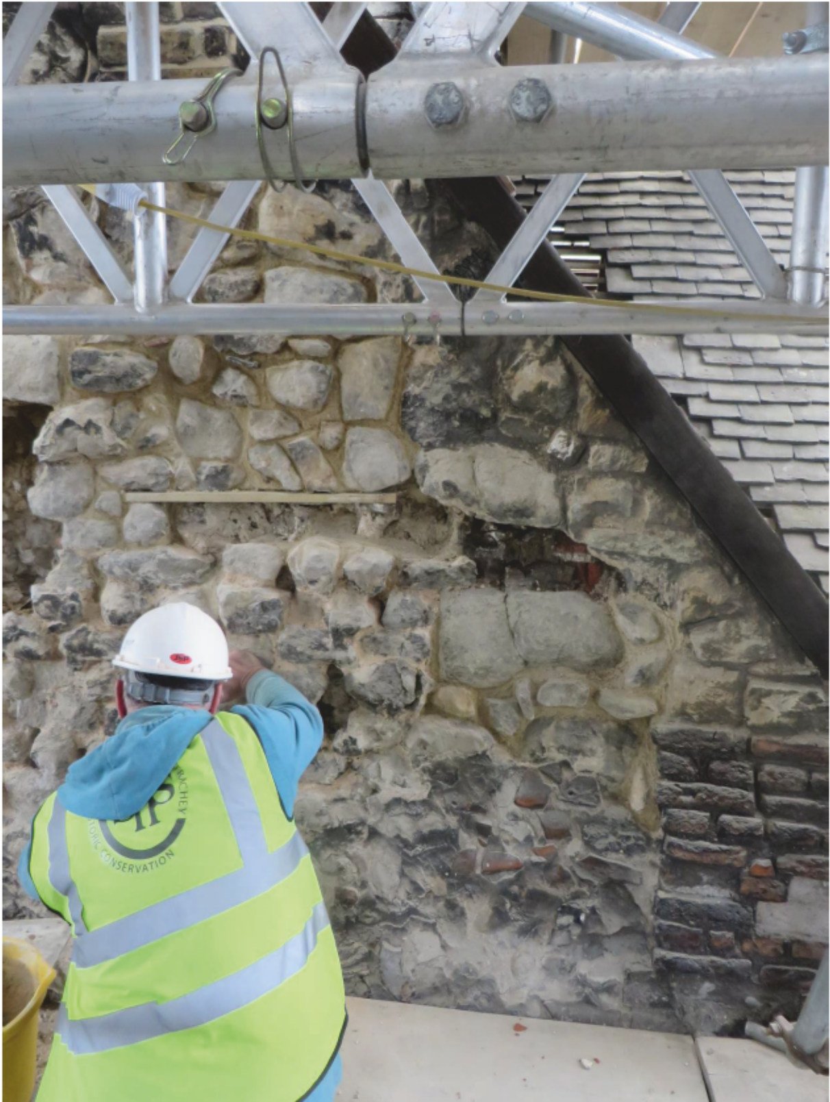
Plate 3: North side of the east gable wall of the Queen's House, looking west
