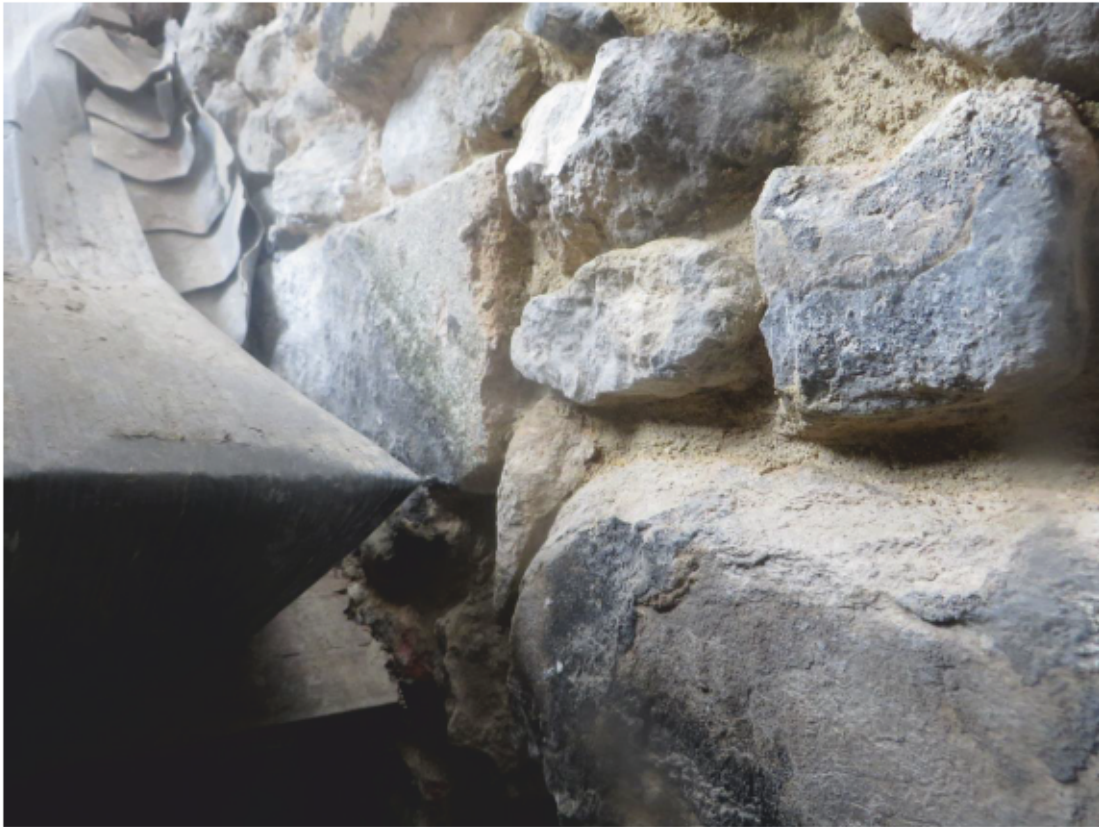
Plate 13: South end of the lower part of the east gable wall of the Queen's House from the lower scaffold level, looking south-west
