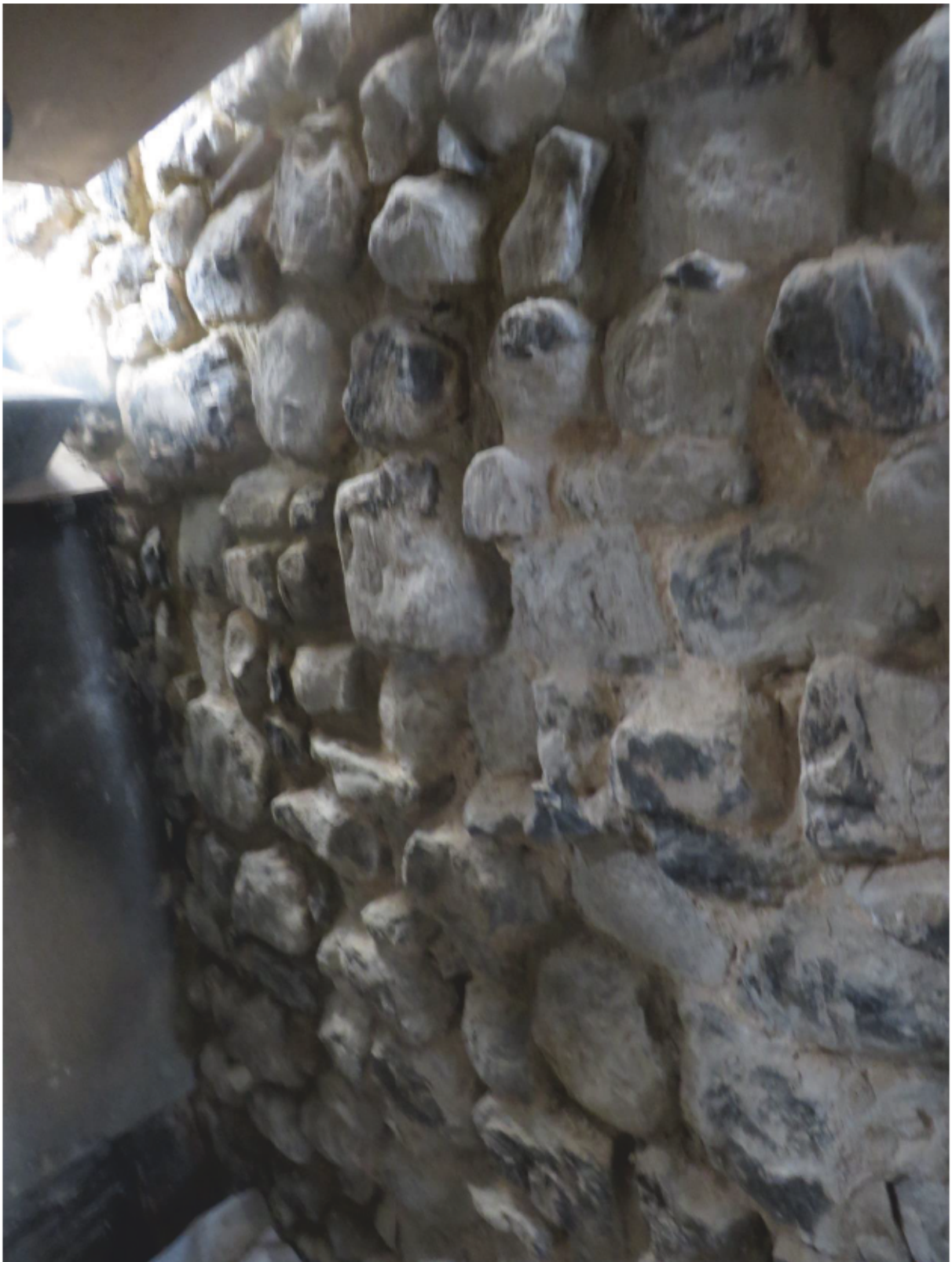
Plate 12: South end of the lower part of the east gable wall of the Queen's House from the lower scaffold level, looking south-west
