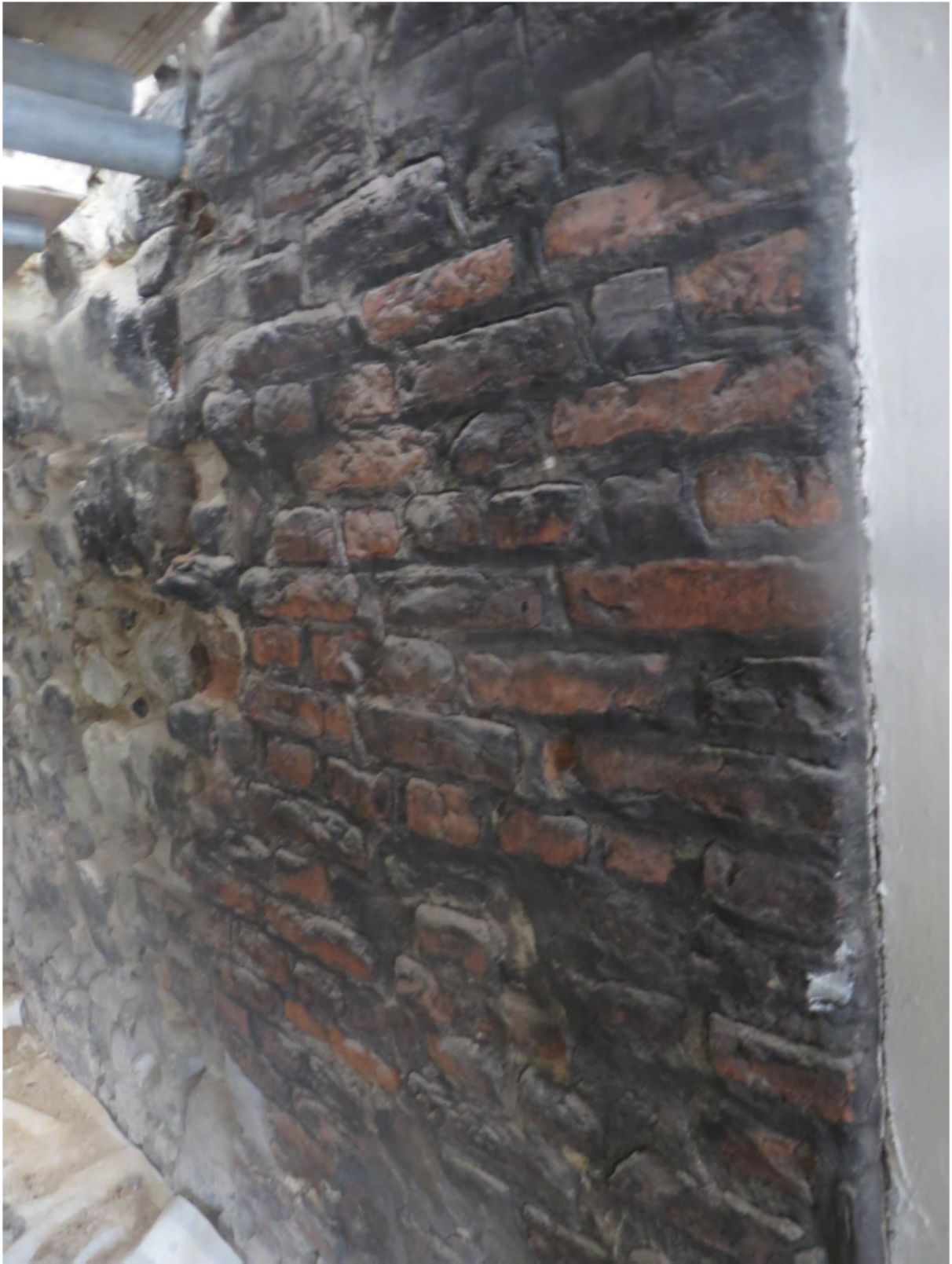
Plate 8: North side of the east gable wall of the Queen's House from the lower scaffold level, looking south-west
