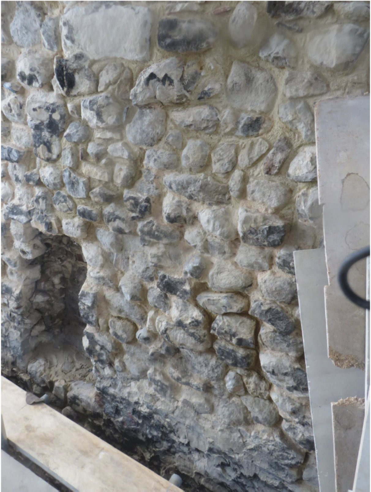
Plate 19: Void marking the position of a former window in the east gable wall of the Queen's House, looking south-west
