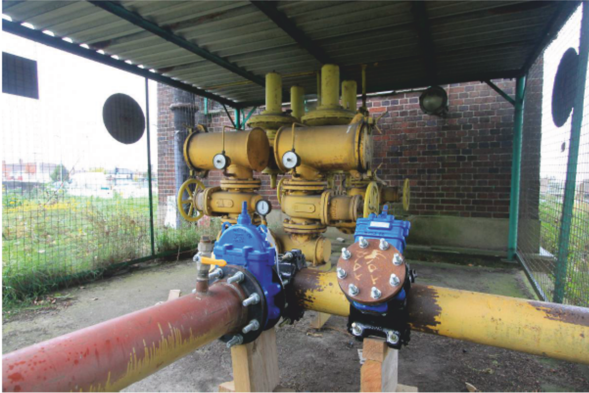
Plate 3 Gas plant to rear of Building 1
