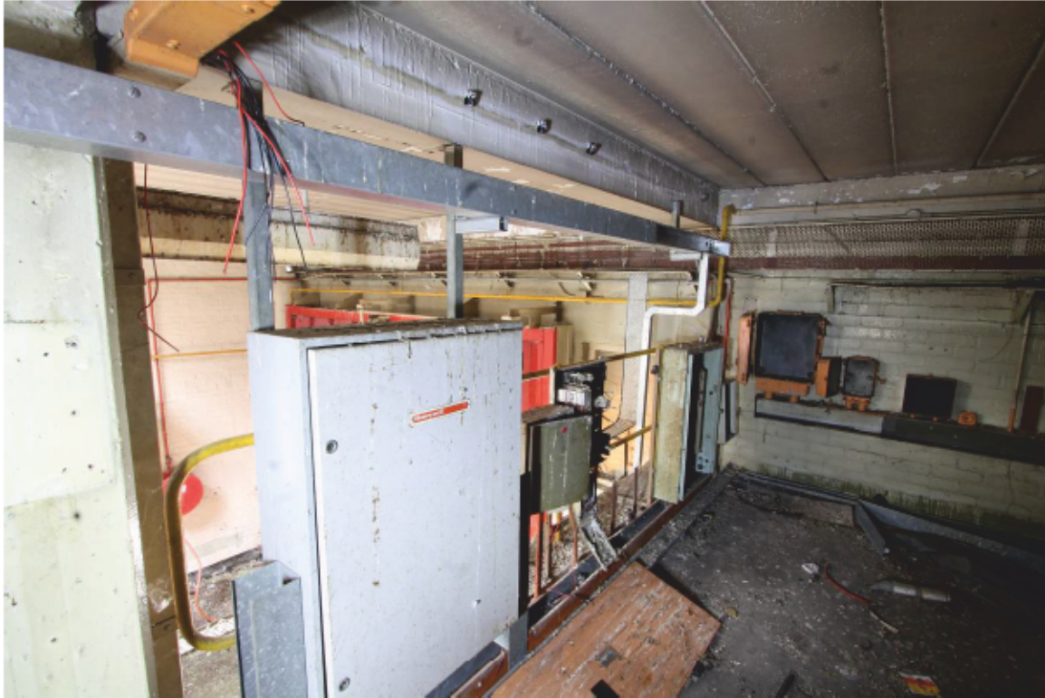
Plate 35 Building 13: Electrical switch gear above central offices, looking south-east
