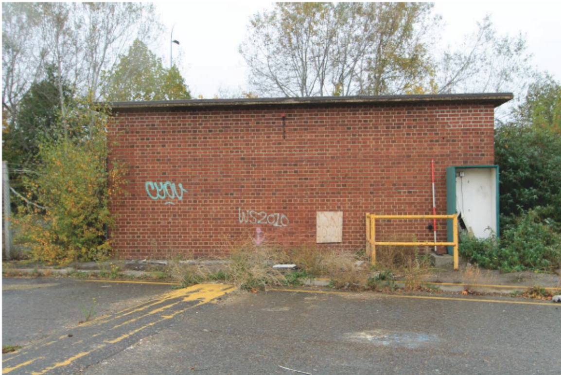
Plate 24 Building 12: Sewage Pump House, looking east
