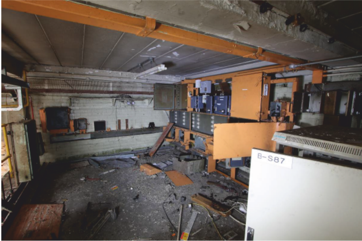
Plate 34 Building 13: Electrical switch gear above central offices, looking south-west
