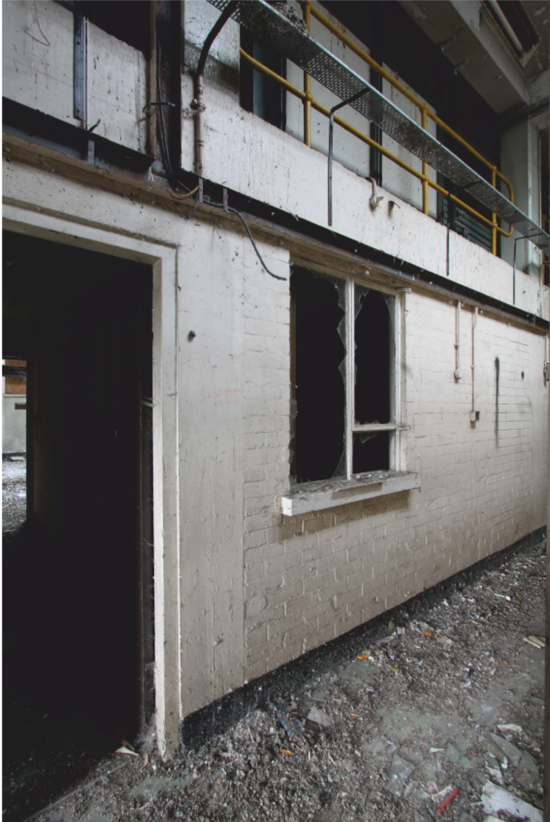
Plate 33 Building 13: Central brick and concrete framed offices, with switchgear and telecoms above
