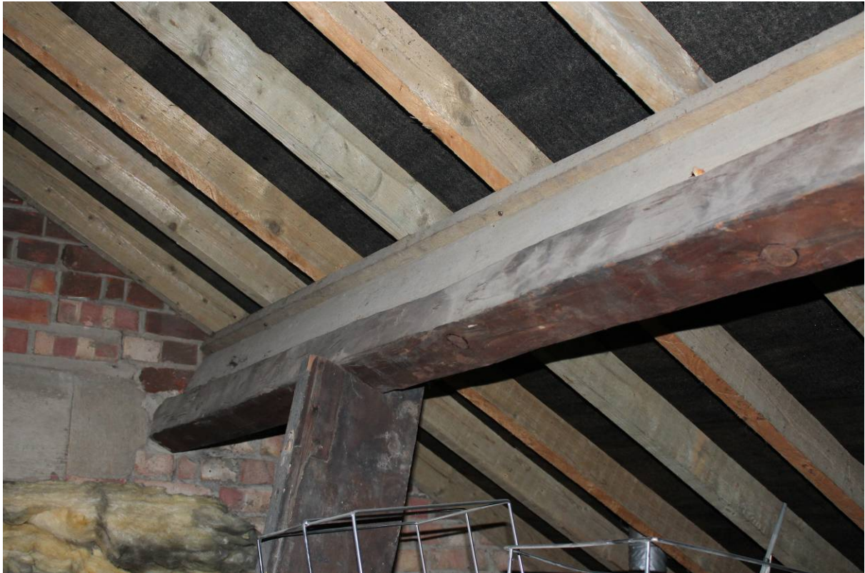
Plate 3 19 th century and modern roofs over FF09 seen through hatch (F3), looking south-east
