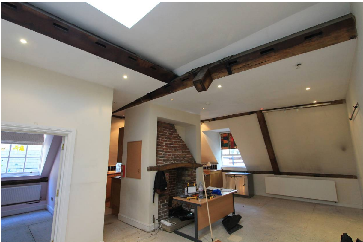
Plate 16 East roof with cut off principal rafters and butt purlins to former central roof well in SF03, looking north-east
