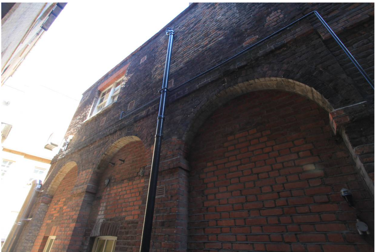
Plate 1b Rebuilt and blocked arches of early 19 th century 'covered way' extension, looking north-west
