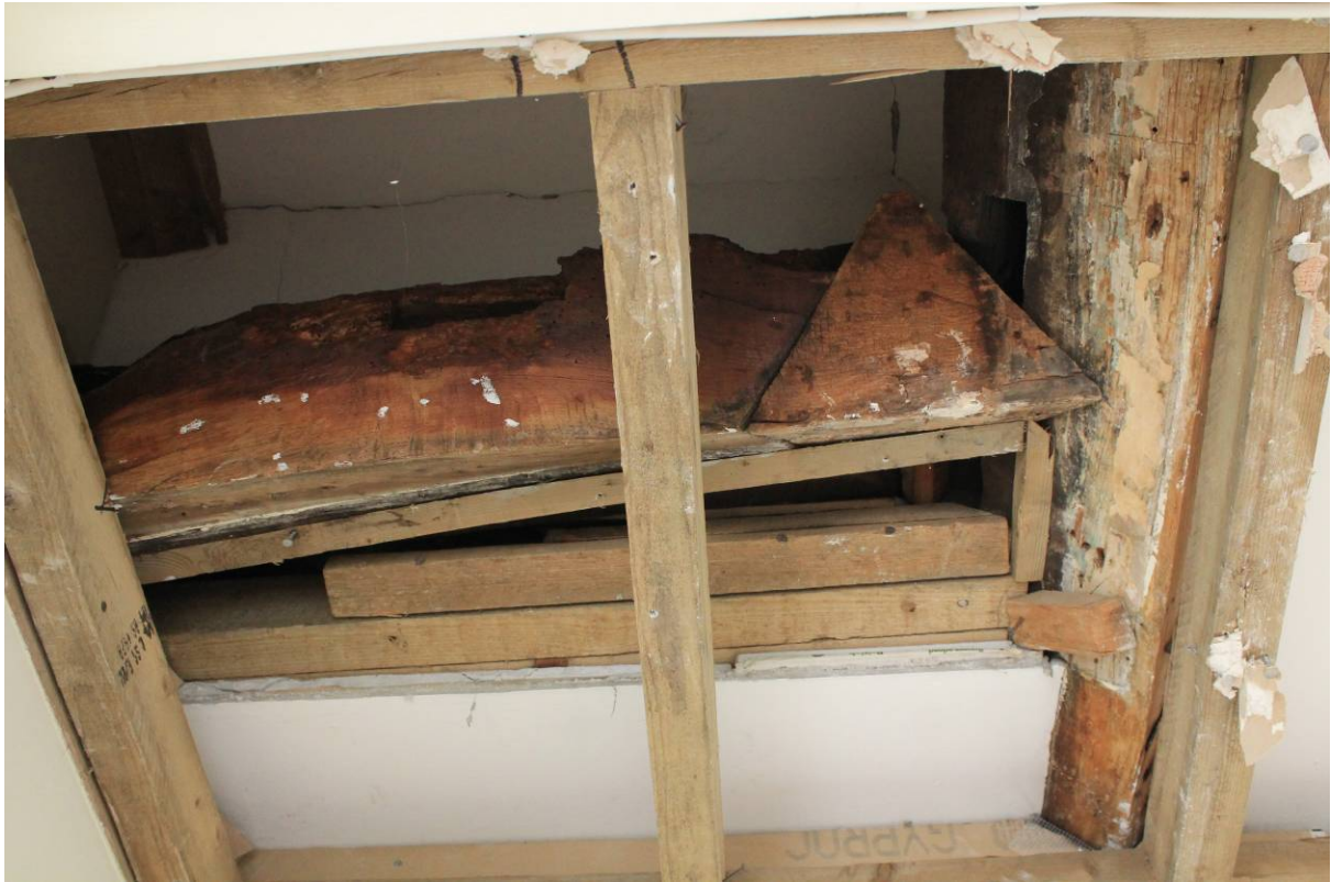
Plate 15 Collar, purlin and cut-off hip rafter over cupboard (S14) in SF07, looking south
