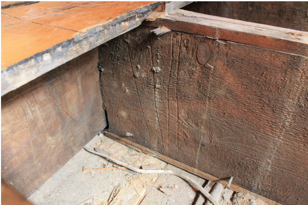
Plate 2 Floor Joist and bridging beam showing carpenter's marks (scribed IIII) following removal of floorboards (F1) in FF01, looking north-west
