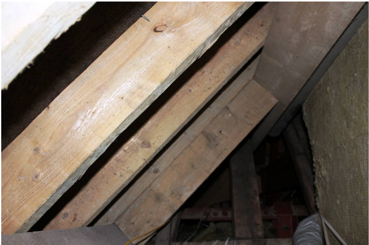
Plate 12 View east from (S11) showing modern roof over (SF08) towards the historic western roof
