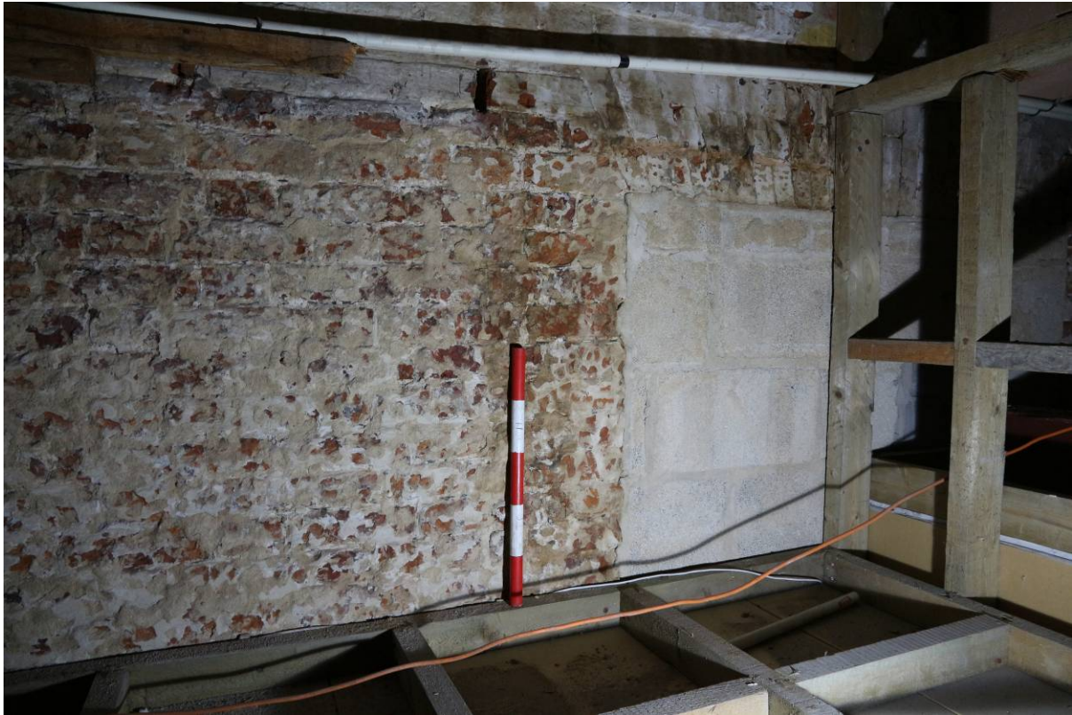
Plate 1c Blocked window in former external south wall visible in void above hatch (G1) above GF09, looking north-east
