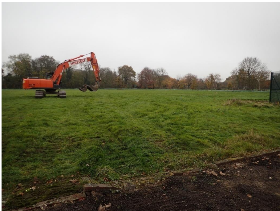
Plate 1. Area of south tennis courts (Area 1), compound and central tennis court (Area 2), facing south.
