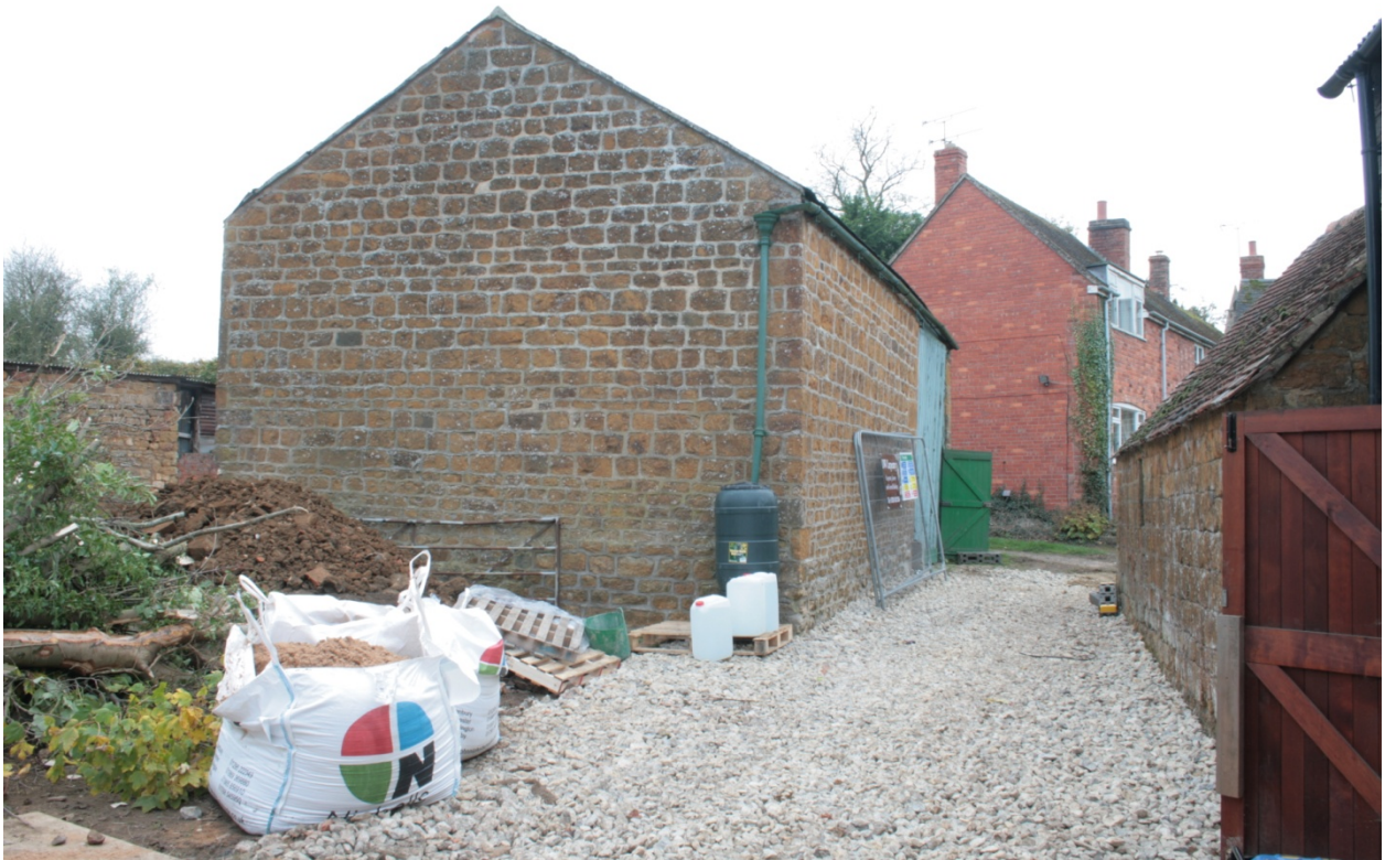
Plate 29: North gable of main barn (Building B), looking south (CSFS17 D100 (76)) (viewpoint on Figure 9)
