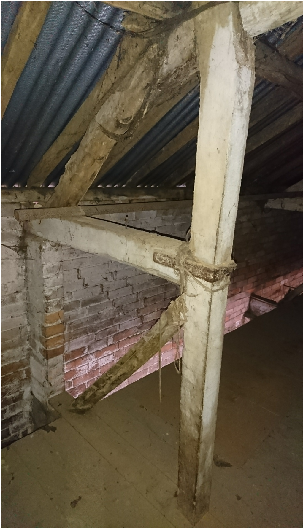
Plate 21: West end of south truss at first floor level in Building A, looking north-west (DSC_2325) (viewpoint on Figure 10)
