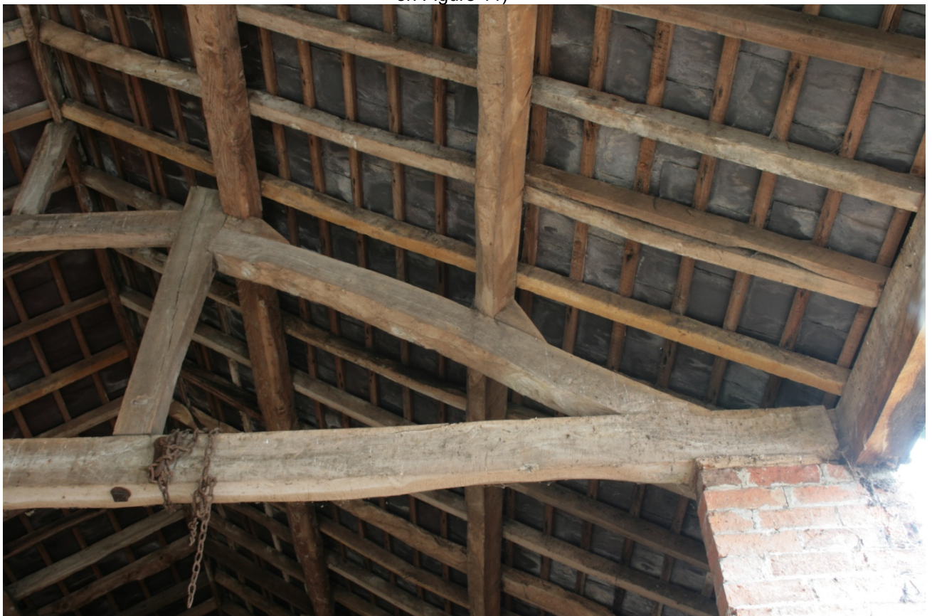
Plate 45: East end of south queen post truss in main barn (Building B), looking north (CSFS17 D100 (28)) (viewpoint on Figure 11)
