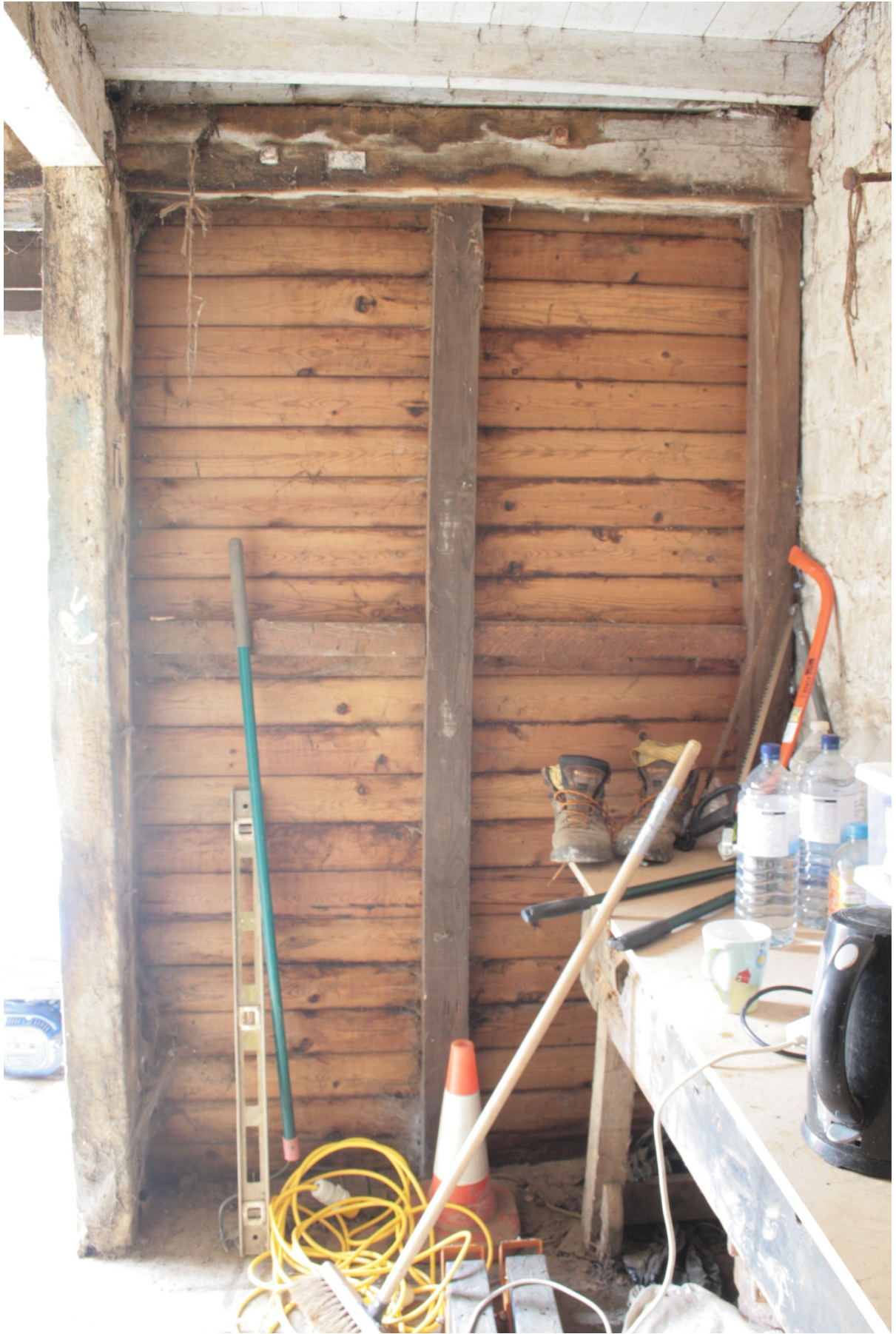
Plate 15: South end of the east wall of Building A, looking east (CSFS17 D100 (94)) (viewpoint on Figure 10)
