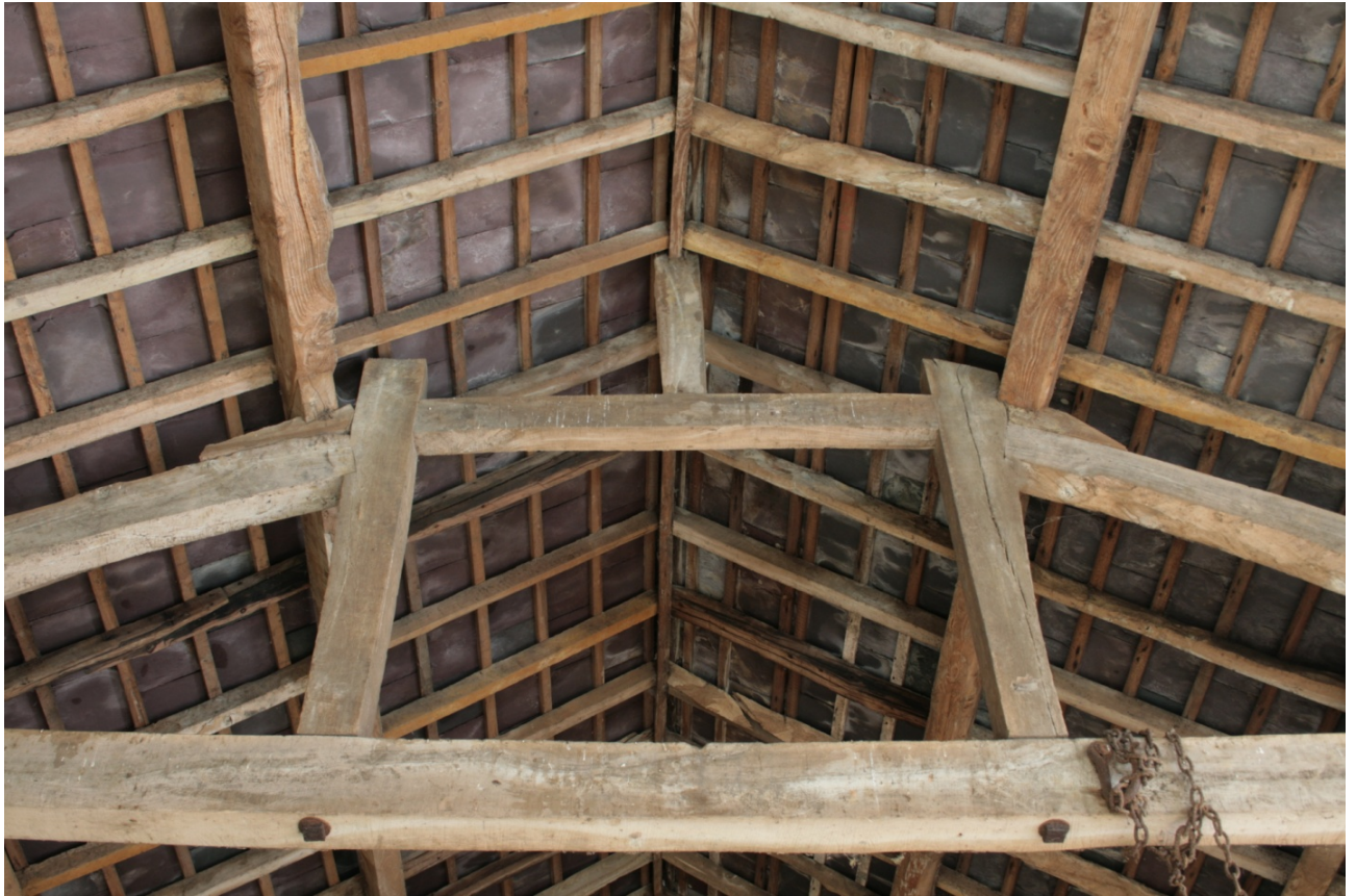
Plate 44: South queen post truss in main barn (Building B), looking north (CSFS17 D100 (29)) (viewpoint on Figure 11)
