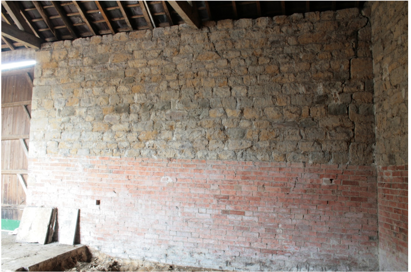
Plate 33: North end of internal east wall, looking west (CSFS17 D100 (10)) (viewpoint on Figure 11)
