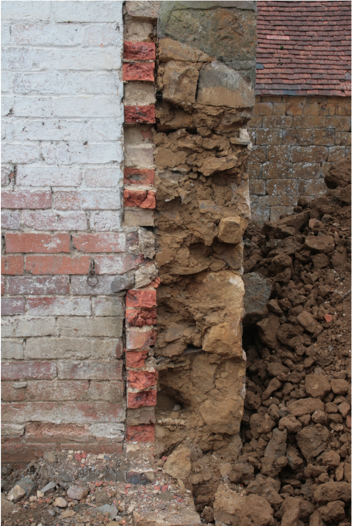
Plate 28: North end of the east elevation of main barn (Building B), looking west (CSFS17 D100 (66)) (viewpoint on Figures 9 and 11)
