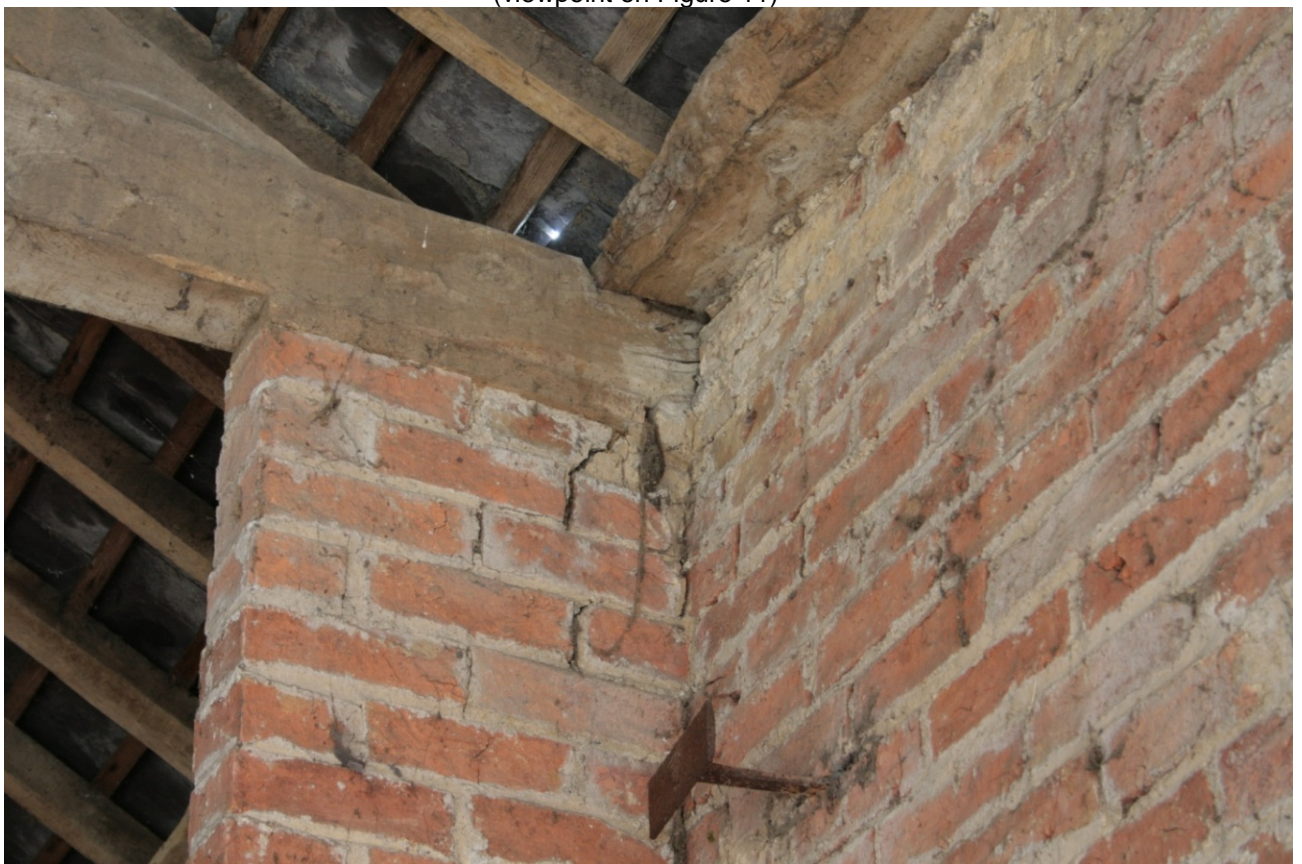
Plate 41: East end of north tie-beam in main barn (Building B), looking north (CSFS17 D100 (7)) (viewpoint on Figure 11)
