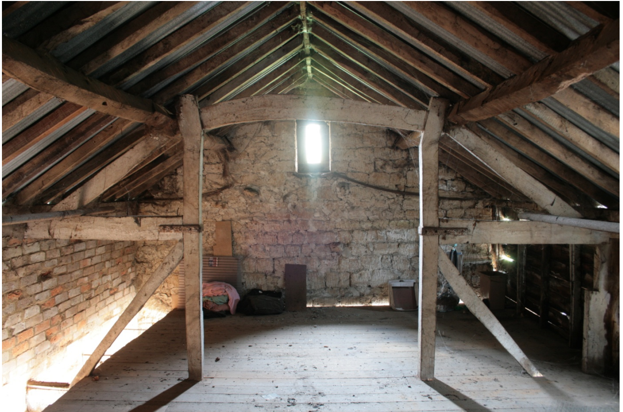
Plate 22: North truss at first floor level in Building A, looking north (CSFS17 D100 (102)) (viewpoint on Figure 10)
