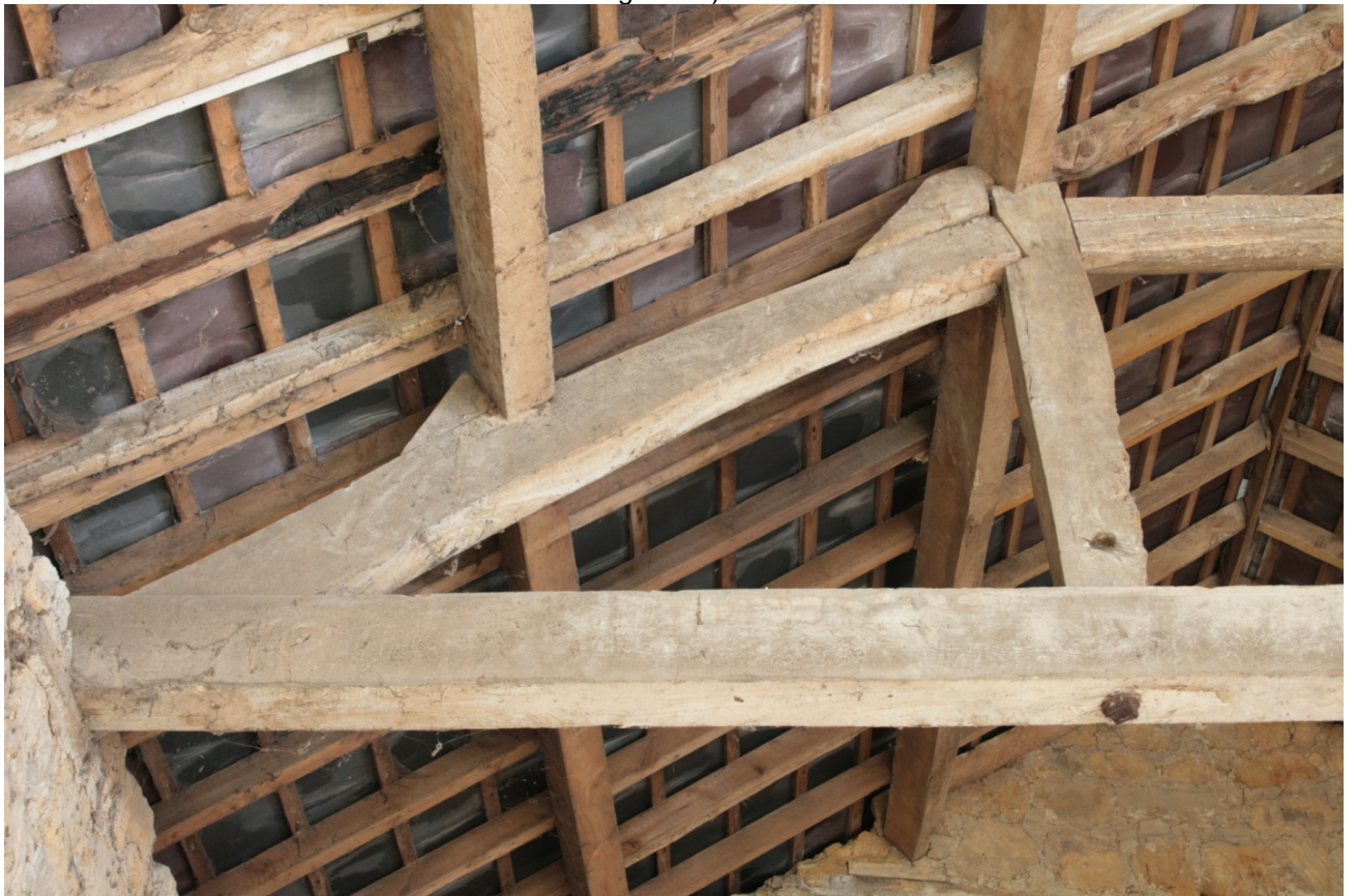
Plate 39: West end of north queen post truss in main barn (Building B), looking north (CSFS17 D100 (3)) (viewpoint on Figure 11)
