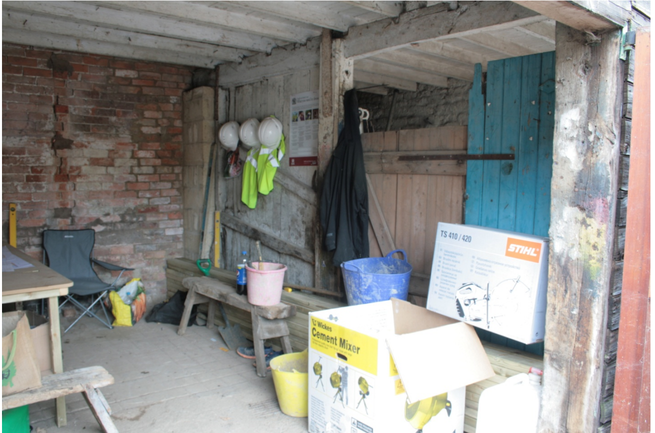
Plate 13: North side of ground floor of Building A, looking north-west (CSFS17 D100 (88)) (viewpoint on Figure 10)
