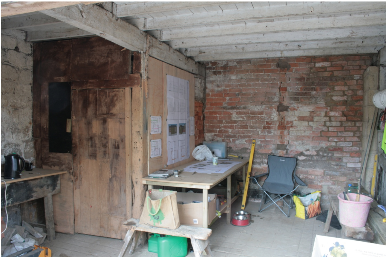
Plate 12: South side of ground floor of Building A, looking west (CSFS17 D100 (81)) (viewpoint on Figure 10)
