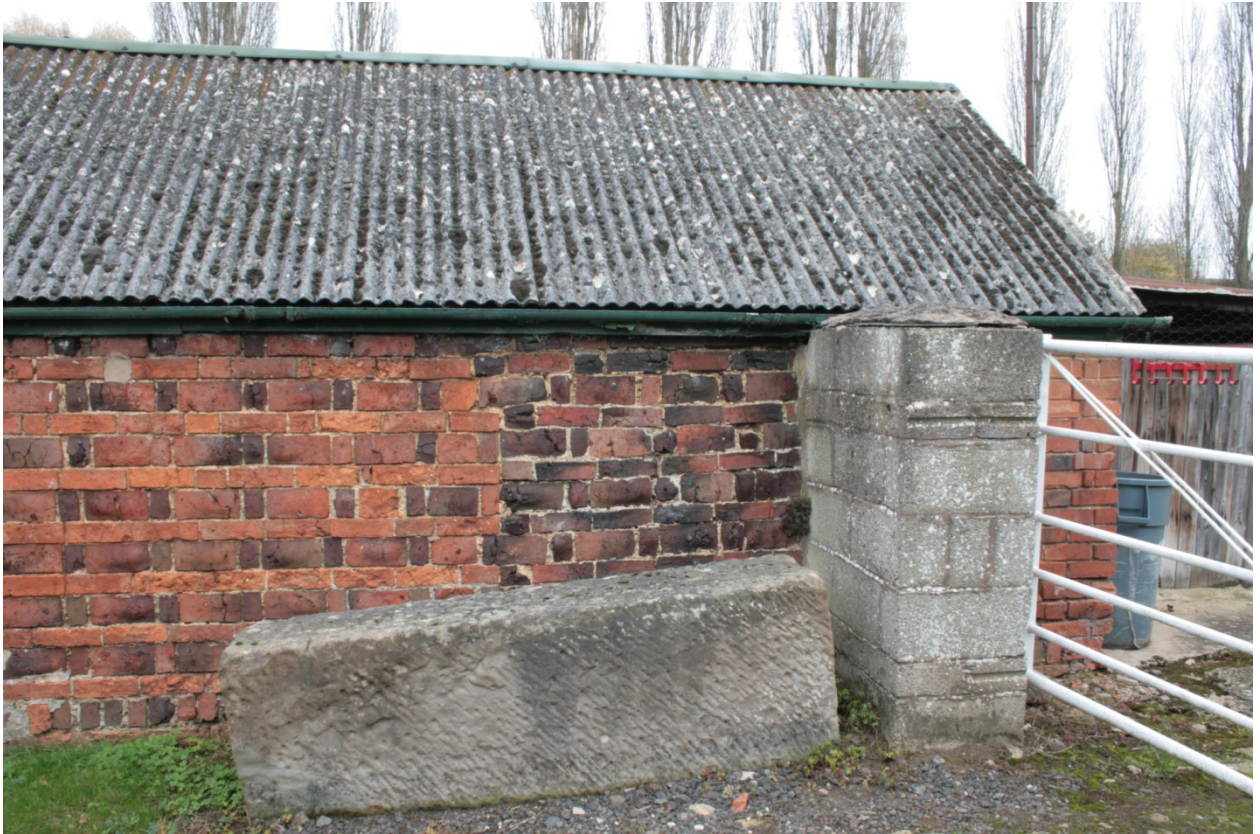
Plate 50: South elevation of Building C, looking north (CSFS17 D100 (63)) (viewpoint on Figures 9 and 12)
