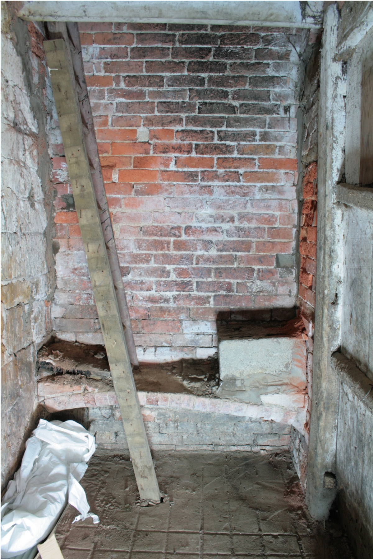
Plate 17 : Ladder access from ground to first floor, looking west (CSFS17 D100 (101)) (viewpoint on Figure 10)
