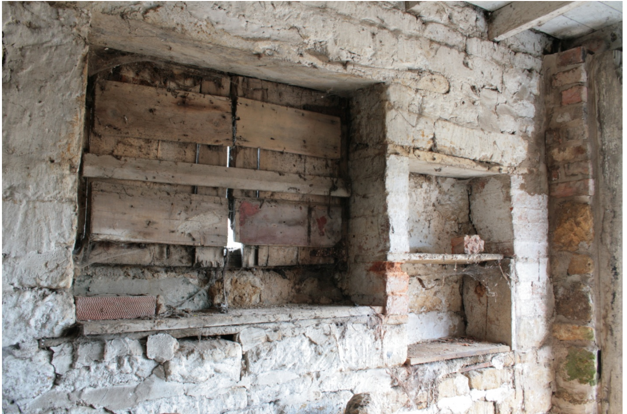
Plate 11: Window and niche in north gable wall of Building A, looking north (CSFS17 D100 (86)) (viewpoint on Figure 10)
