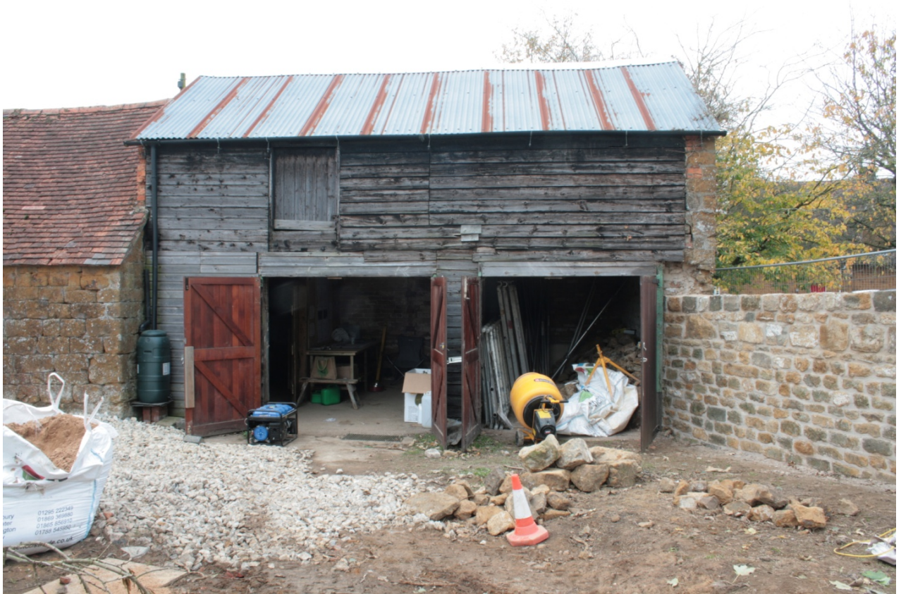
Plate 5: East front elevation of Building A, looking west (CSFS17 D100 (78)) (viewpoint on Figure 9)
