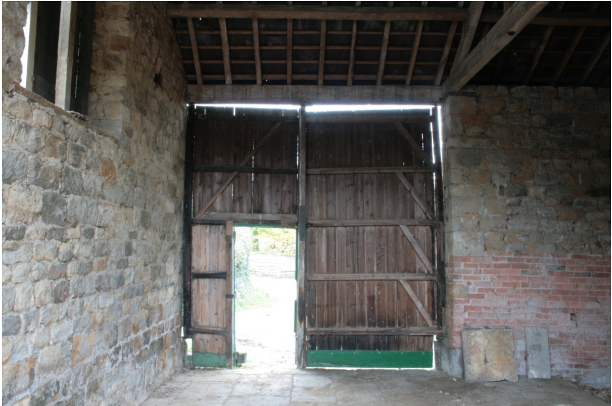
Plate 31: Front west barn door in main barn (Building B), looking west (CSFS17 D100 (35)) (viewpoint on Figure 11)
