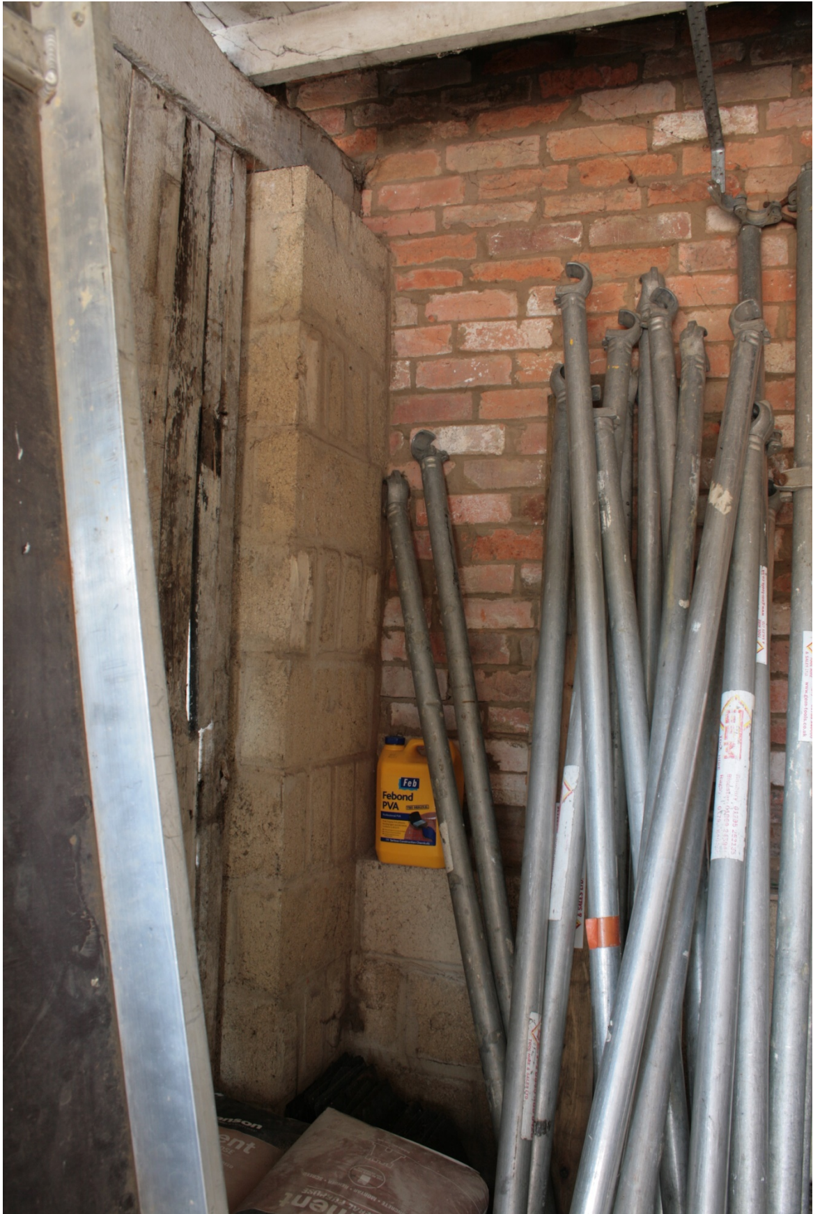
Plate 10: North side of ground floor of Building A, looking west (CSFS17 D100 (87) (viewpoint on Figure 10)
