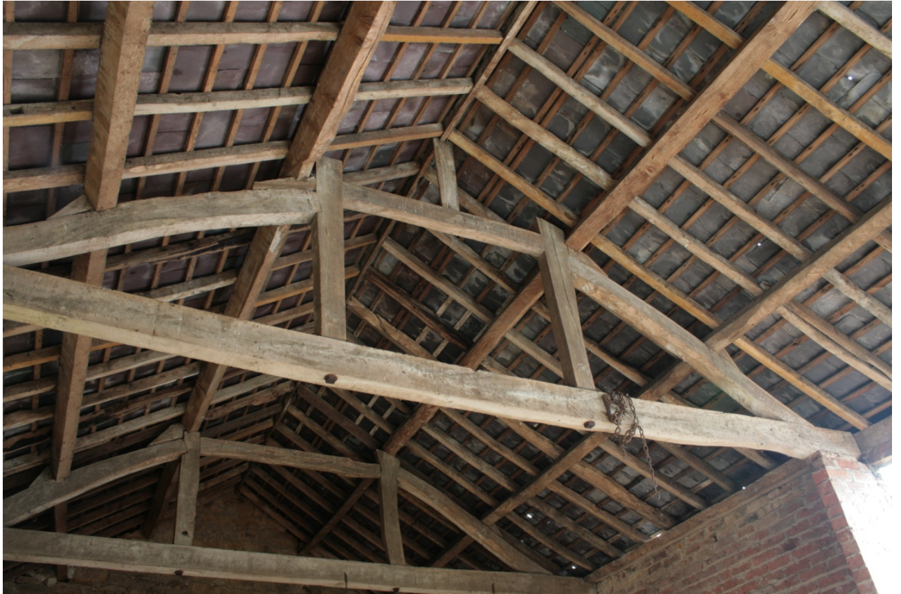
Plate 42: South queen post truss in main barn (Building B), looking north-east (CSFS17 D100 (26)) (viewpoint on Figure 11)
