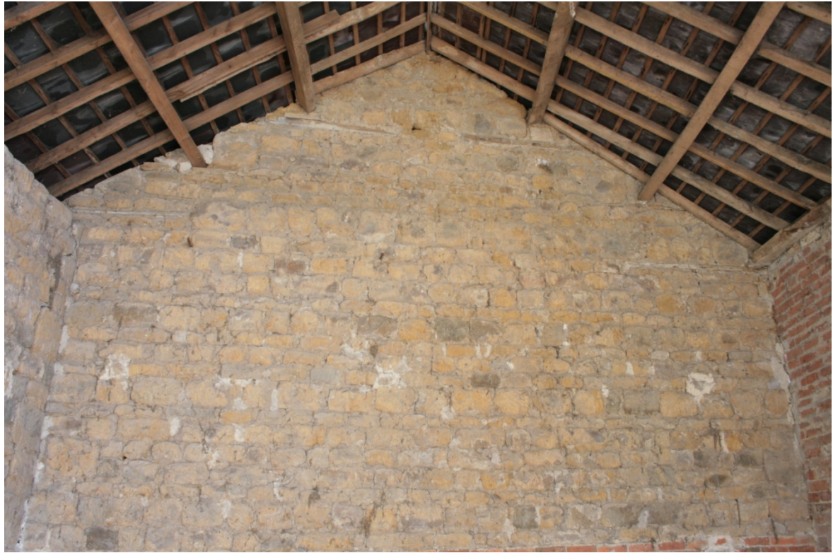
Plate 35: North gable wall in main barn (Building B), looking north (CSFS17 D100 (8)) (viewpoint on Figure 11)
