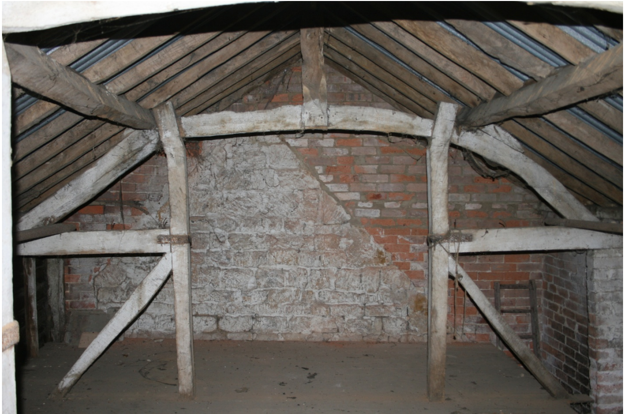
Plate 18: South truss in first floor of Building A, looking south CSFS17 D100 (108) (viewpoint on Figure 10)
