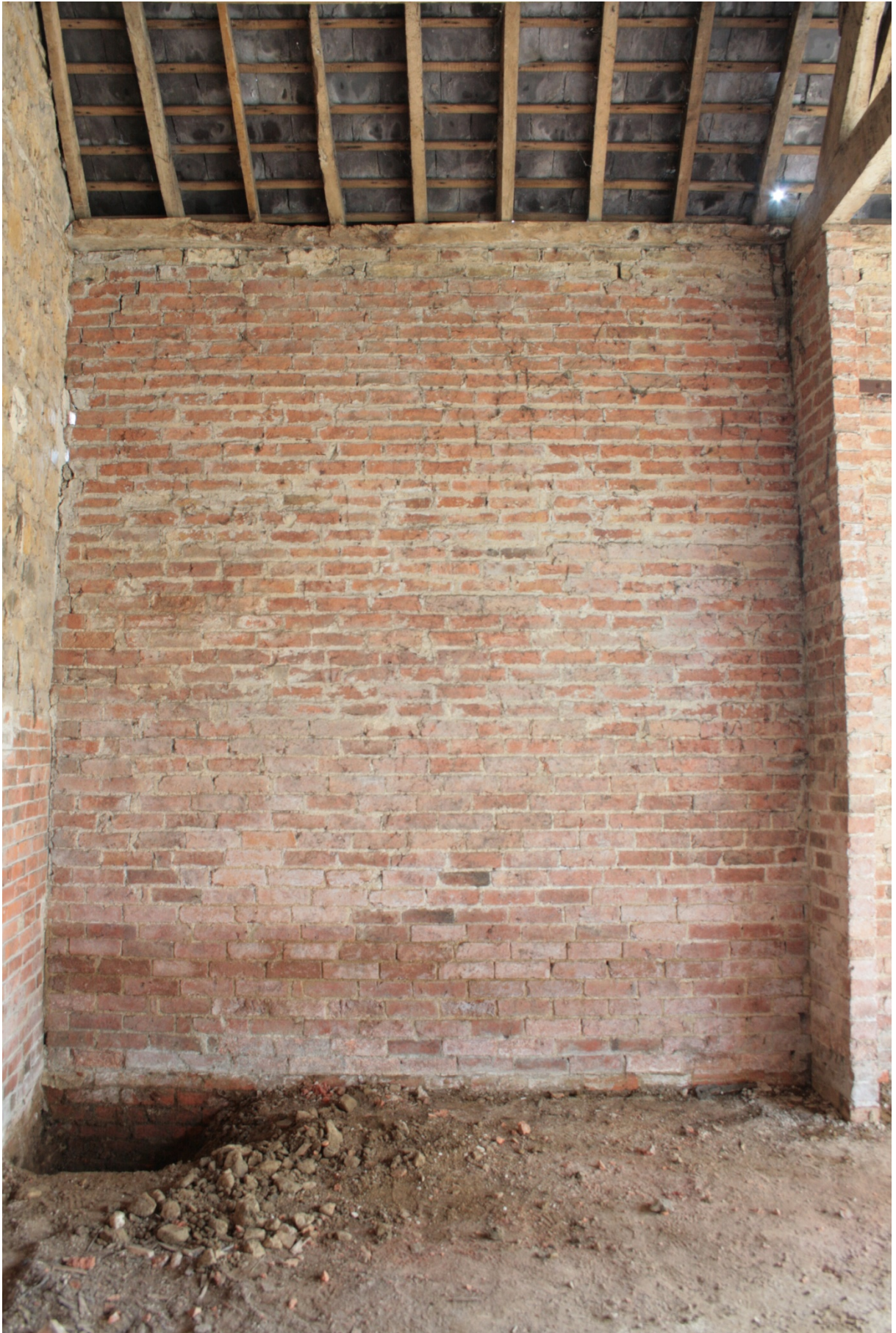
Plate 37: Northern part of the east wall, looking east (CSFS17 D100) (viewpoint on Figure 11)
