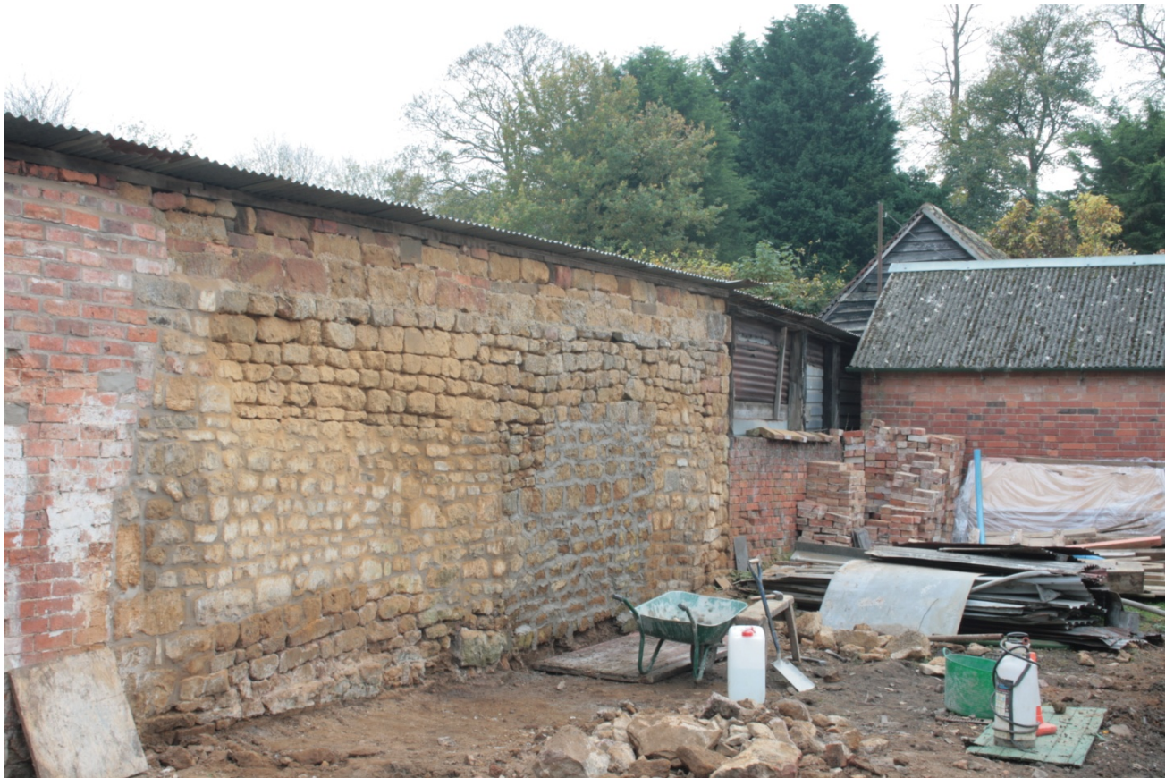
Plate 52: Building C (right) and west elevation of buildings to the east, looking south (CSFS17 D100 (71)) (viewpoint on Figure 9)
