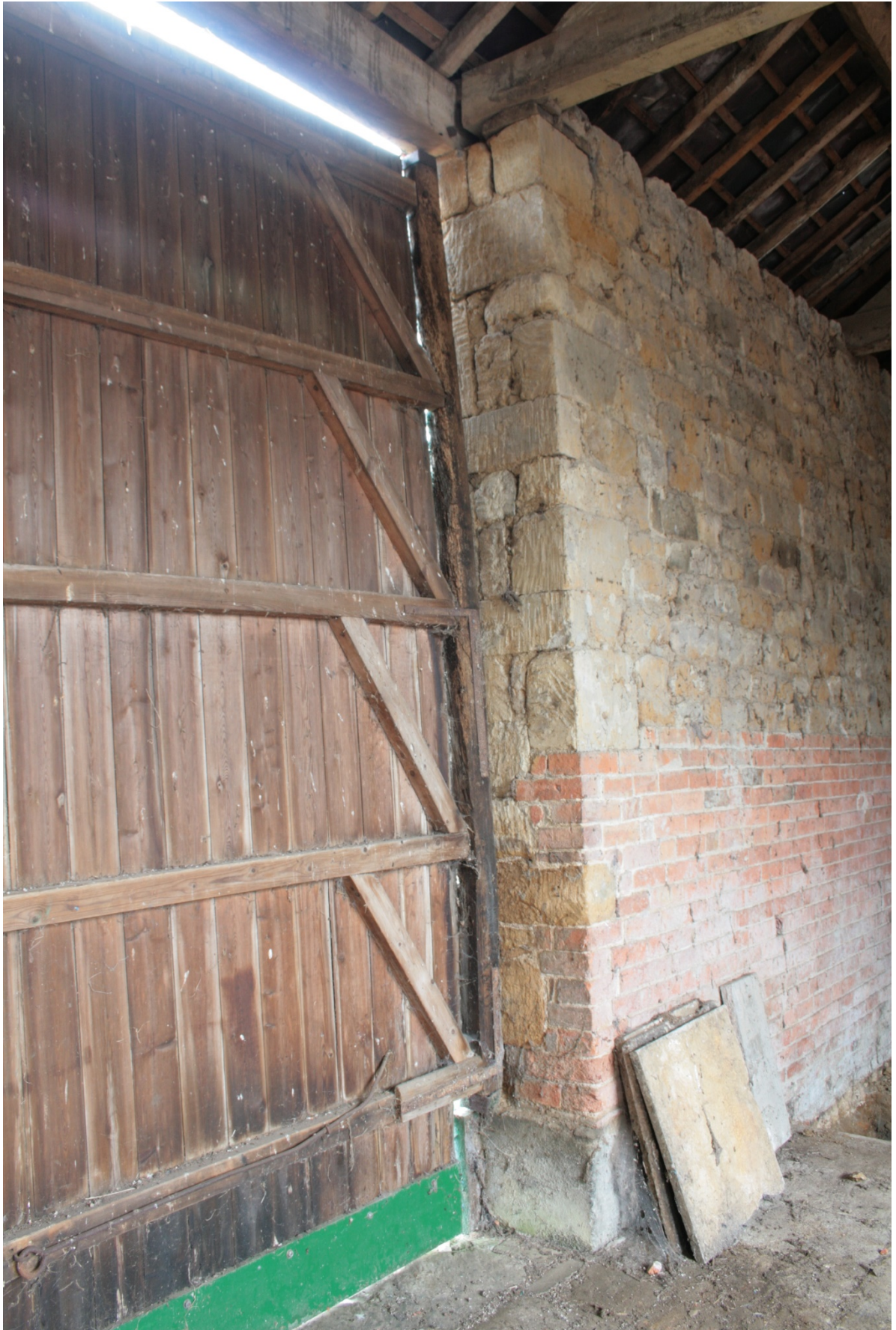
Plate 32: North side of front west barn door in main barn (Building B), looking north-west (CSFS17 D100 (38)) (viewpoint on Figure 11)
