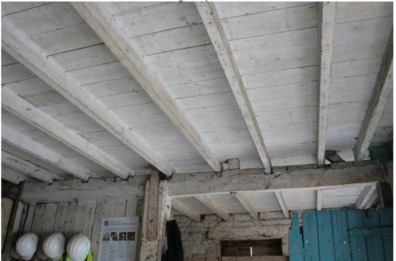
Plate 14: First floor joists in Building A, looking north (CSFS17 D100 (92)) (viewpoint on Figure 10)
