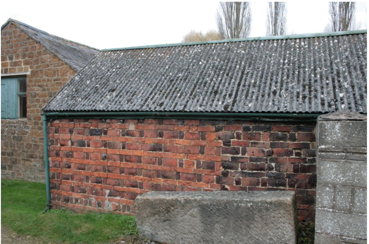
Plate 49: South elevation of Building C, looking north (CSFS17 D100 (62)) (viewpoint on Figures 9 and 12)
