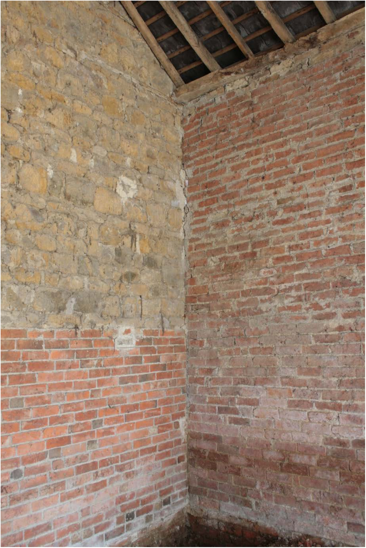
Plate 36: Corner of the north gable wall (left) and east wall (right), looking north-east (CSFS17 D100 (41)) (viewpoint on Figure 11)
