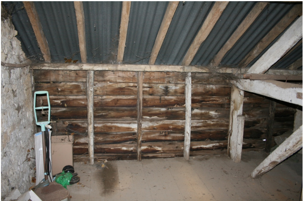
Plate 23: Timber boarding along the north part of the east wall of Building A, looking east (CSFS17 D100 (115)) (viewpoint on Figure 10)
