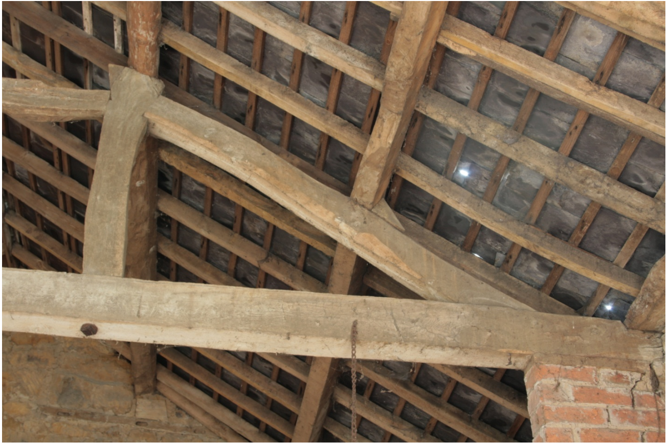
Plate 40: East end of north queen post truss in main barn (Building B), looking north (CSFS17 D100 (5)) (viewpoint on Figure 11)
