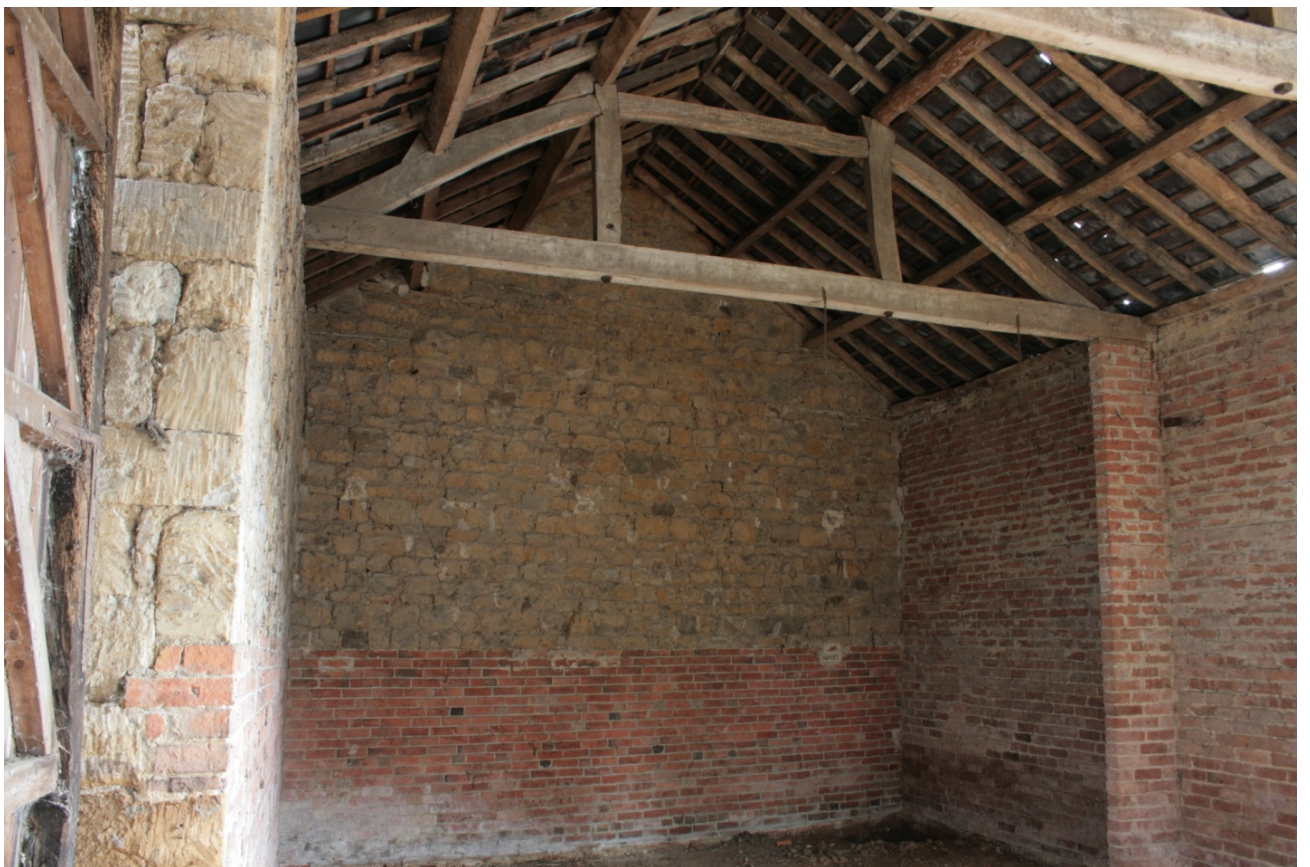
Plate 34: North gable of the main barn (Building B), looking north (CSFS17 D100 (37)) (viewpoint on Figure 11)
