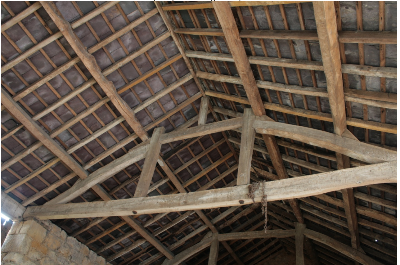
Plate 43: South queen post truss in main barn (Building B), looking north-west (CSFS17 D100 (27)) (viewpoint on Figure 11)
