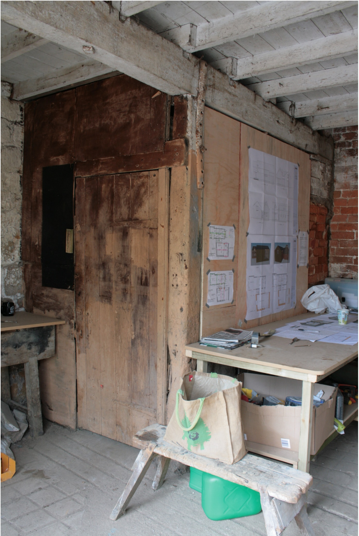
Plate 16: Enclosed entrance to first floor ladder access, looking west (CSFS17 D100 (95)) (viewpoint on Figure 10)
