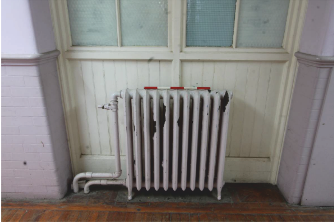
Plate 28 Typical floor mounted heater radiator (16)
