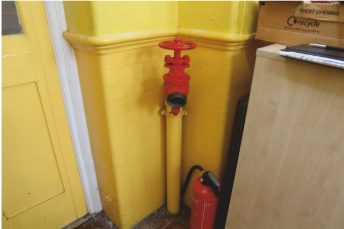
Plate 55: Fire hydrant in Assembly Hall (36), looking north-west
