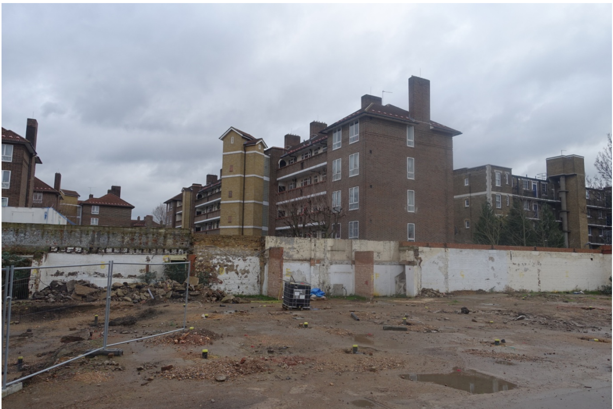
Plate 35 Photograph taken in early 2017 (CField Construction) of the boundary wall with Southey House beyond, looking east (viewpoint on Figure 18)
