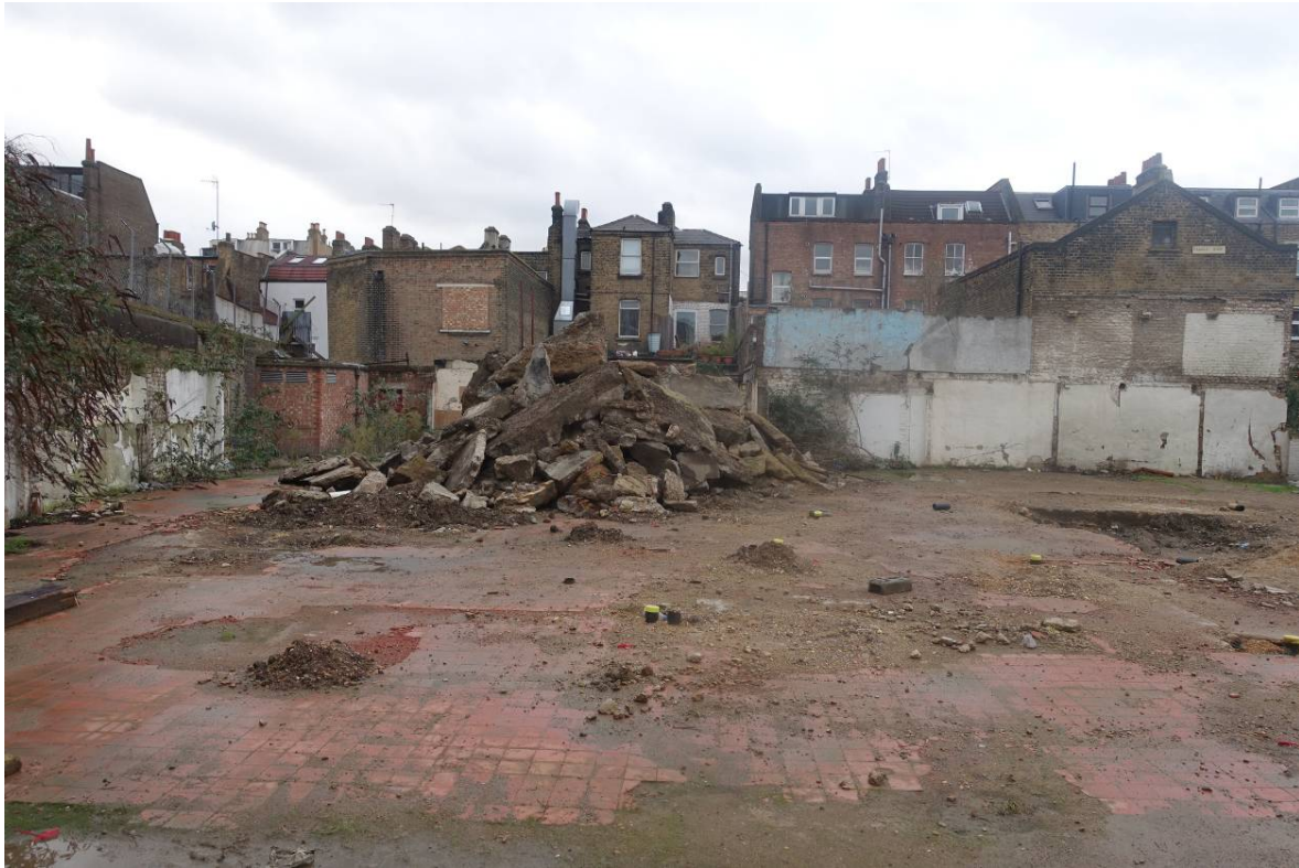
Plate 42 Photograph of the south end of the site taken in early 2017 (CField Construction) showing rear (east) elevations of buildings along Walworth Road, looking west (viewpoint on Figure 18)
