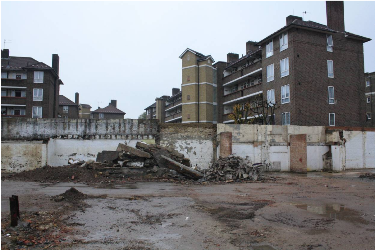
Plate 9 Photograph taken in March 2014 (CgMs part of RPS) of site boundary wall with Cowper House (right) and Southey House (left) beyond, looking east (viewpoint on Figure 17)
