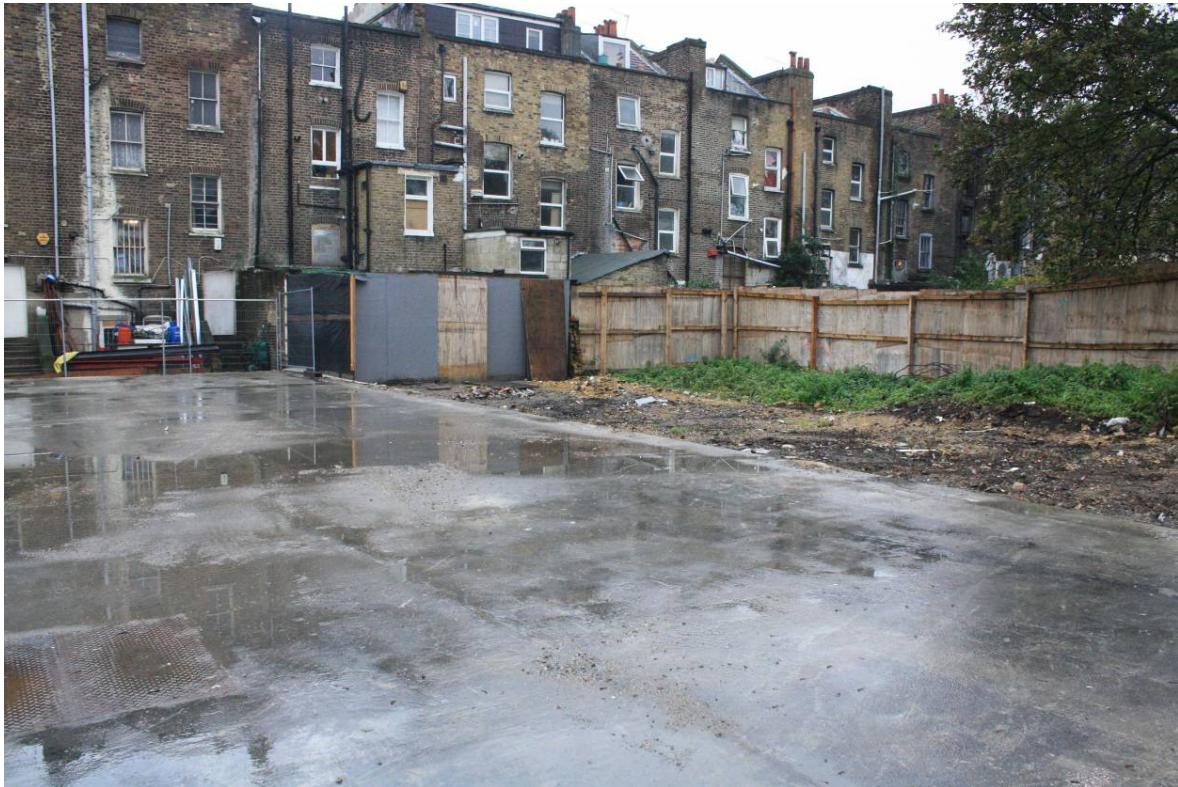
Plate 6 Photograph taken in March 2014 (CgMs part of RPS) showing concrete slab of Building 5 and rear (east) elevations of buildings along Walworth Road, looking north-west (viewpoint on Figure 17)
