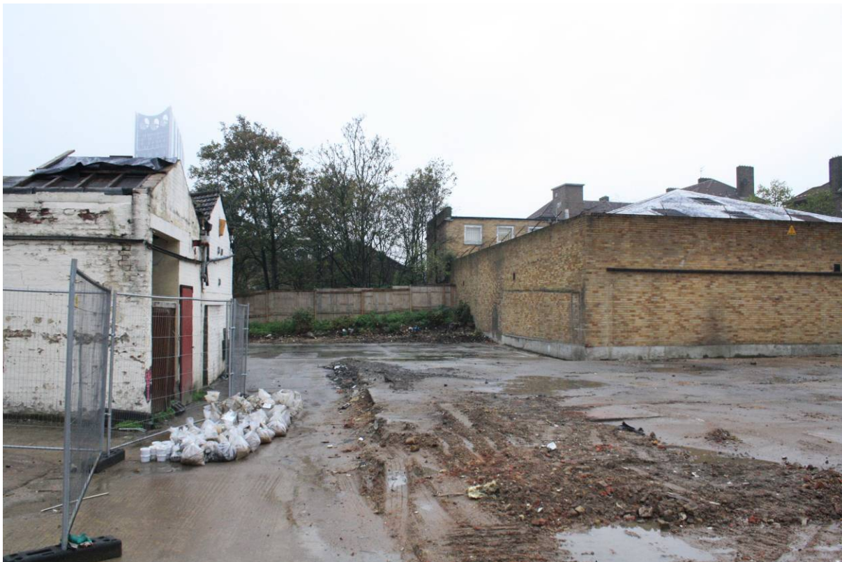
Plate 4 Photograph taken in March 2014 (CgMs part of RPS) of Buildings 3 and 4 (left) and boundary wall around York House, looking north (viewpoint on Figure 17)
