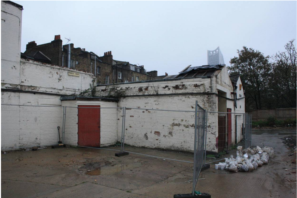
Plate 3 Photograph taken in March 2014 (CgMs part of RPS) of Buildings 1 to 4, looking west (viewpoint on Figure 17)
