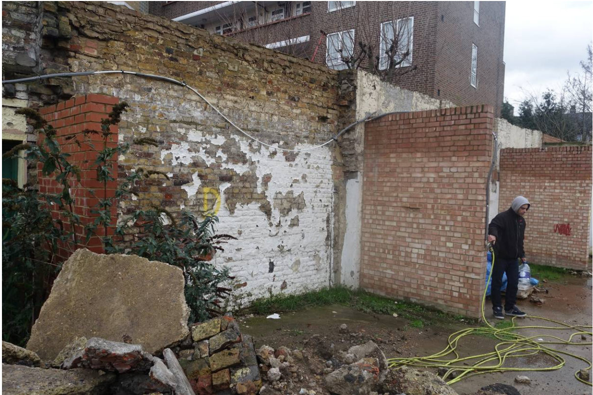
Plate 38 Photograph taken in early 2017 (CField Construction) of the boundary wall with Southey House beyond, looking south-east (viewpoint on Figure 18)
