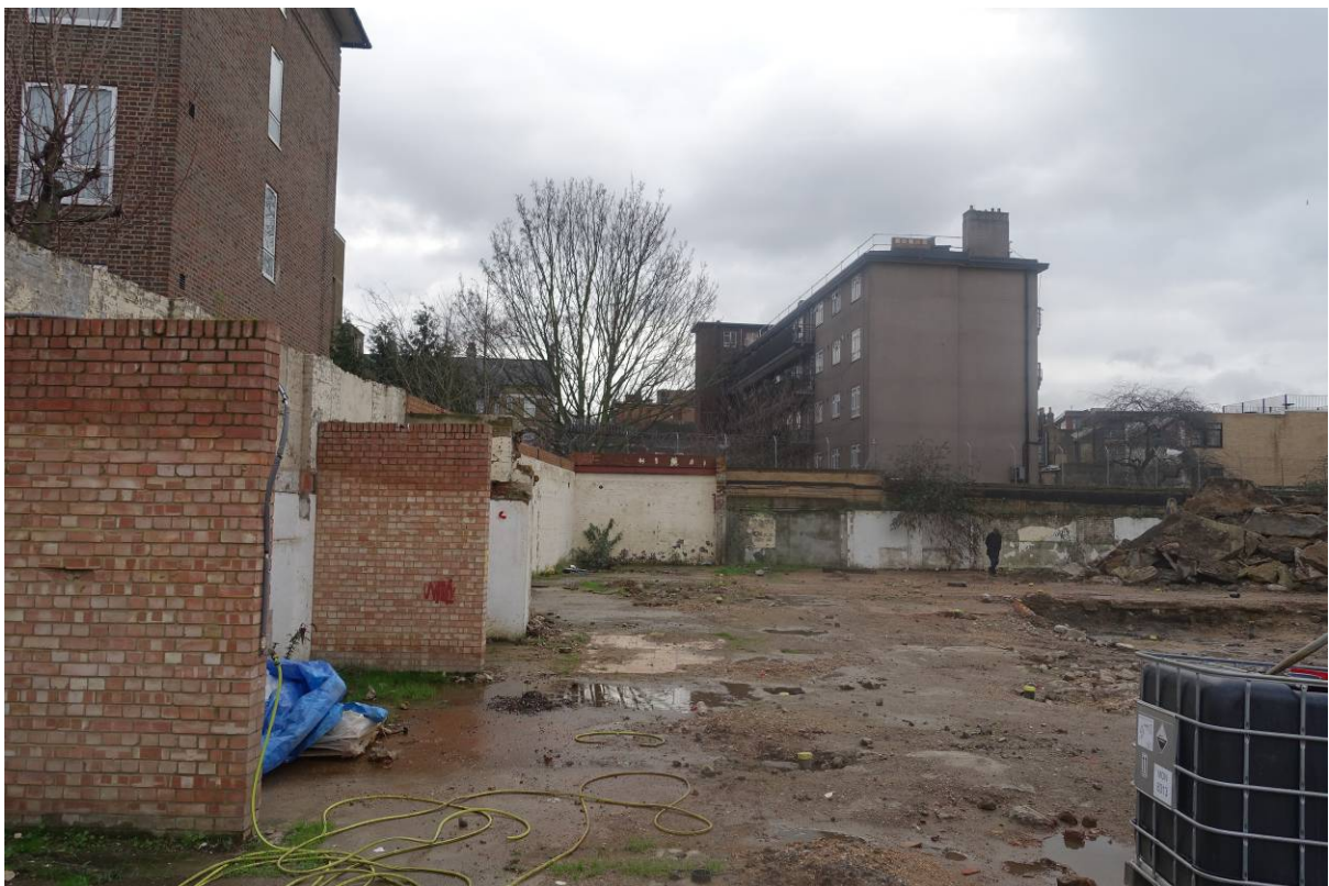
Plate 39 Photograph taken in early 2017 (CField Construction) of the boundary wall with Southey House (left) and Manchester House (centre) beyond, looking south (viewpoint on Figure 18)
