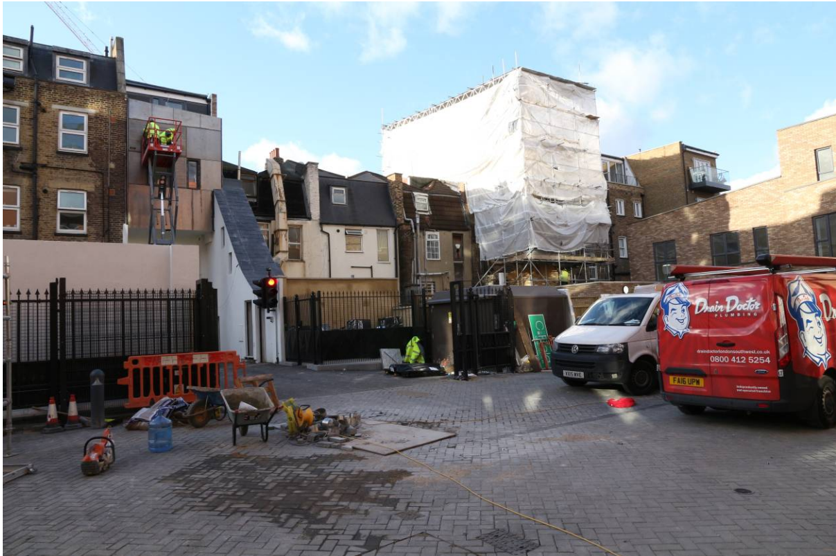
Plate 46 Photograph taken in December 2017 (PCA) of site entrance (left) and rear (east) elevations of properties along Walworth Road, looking north-west (viewpoint on Figure 19)
