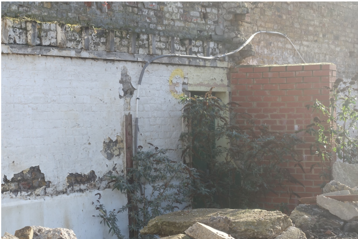
Plate 33 Photograph taken in early 2017 (CField Construction) of the boundary wall, looking south-east (viewpoint on Figure 18)
