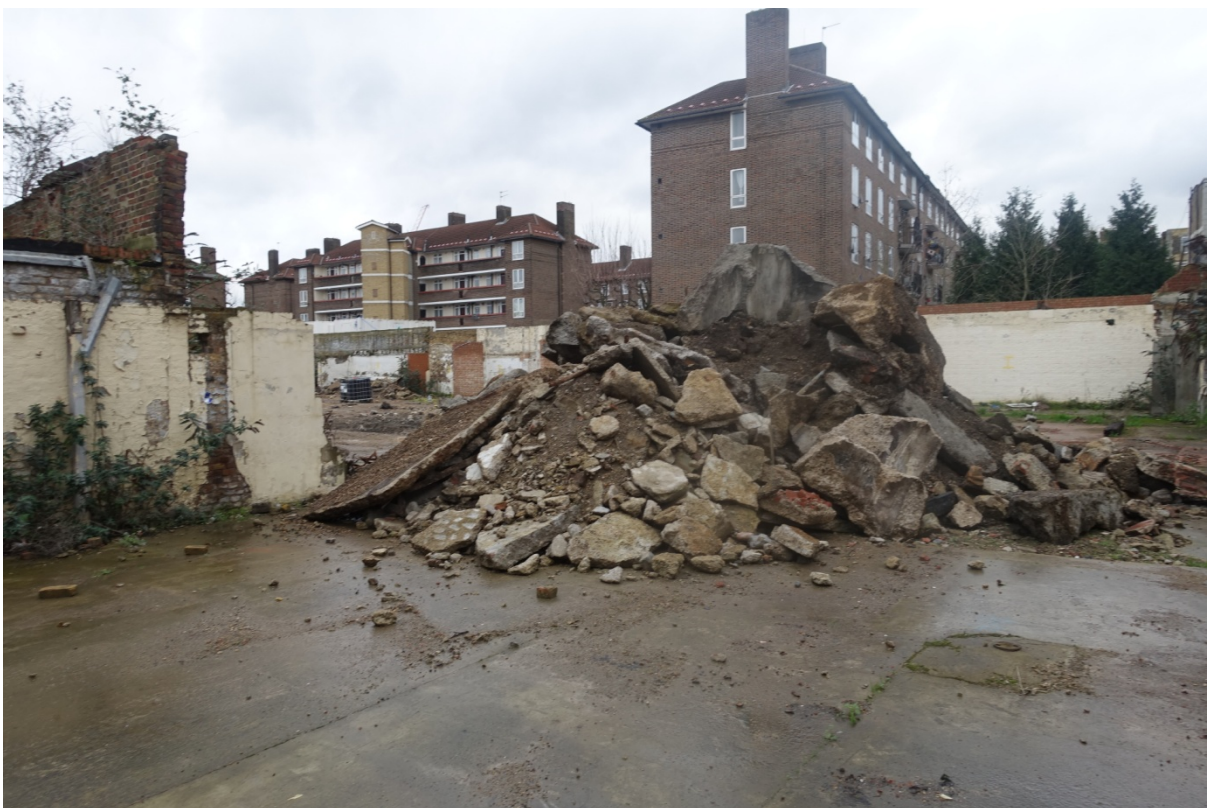
Plate 37 Photograph taken in early 2017 (CField Construction) of the boundary wall with Cowper House (left) and Southey House (right) beyond, looking north-east (viewpoint on Figure 18)
