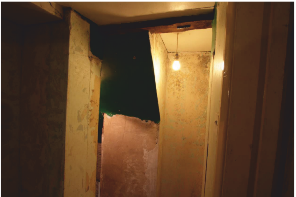
Plate 39: First floor Landing looking south (D2 016)
