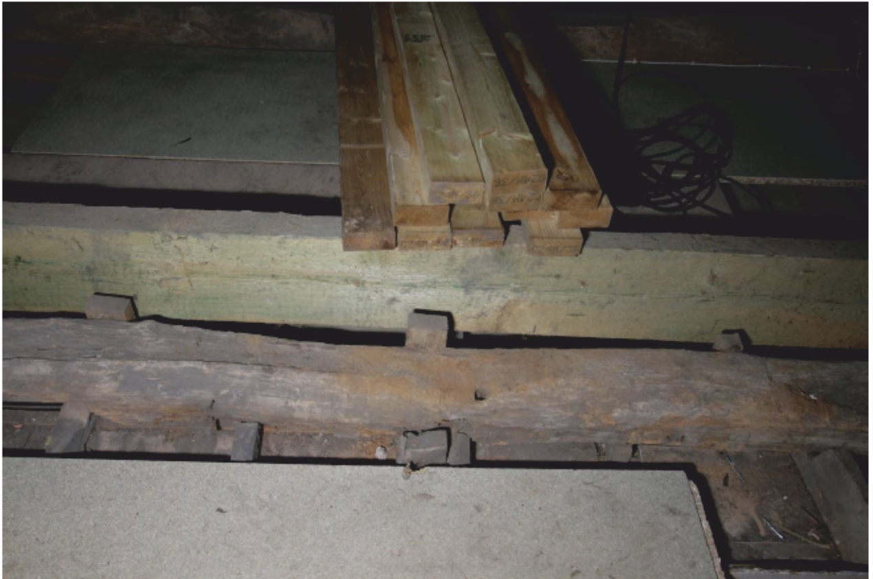
Plate 59: Tie beam in roof space over Bedroom 3 and Landing, looking east (D3 023)
