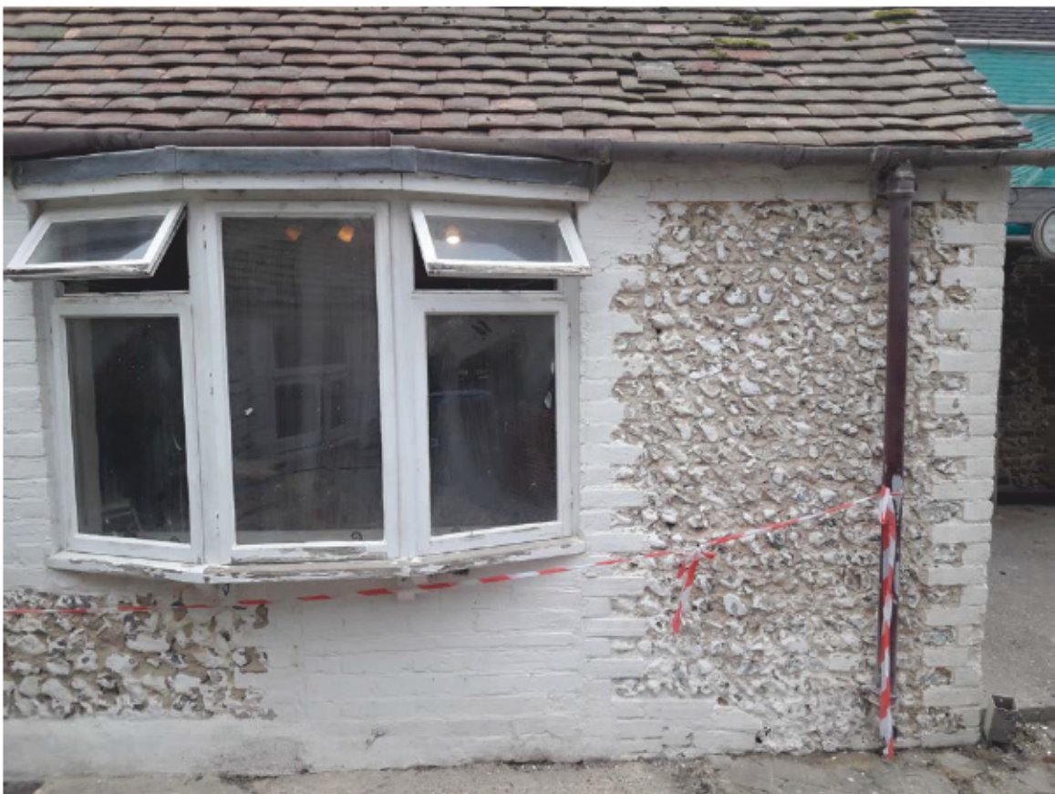
Plate 11: South elevation of the Kitchen, looking north (photograph provided by George Roberts)
