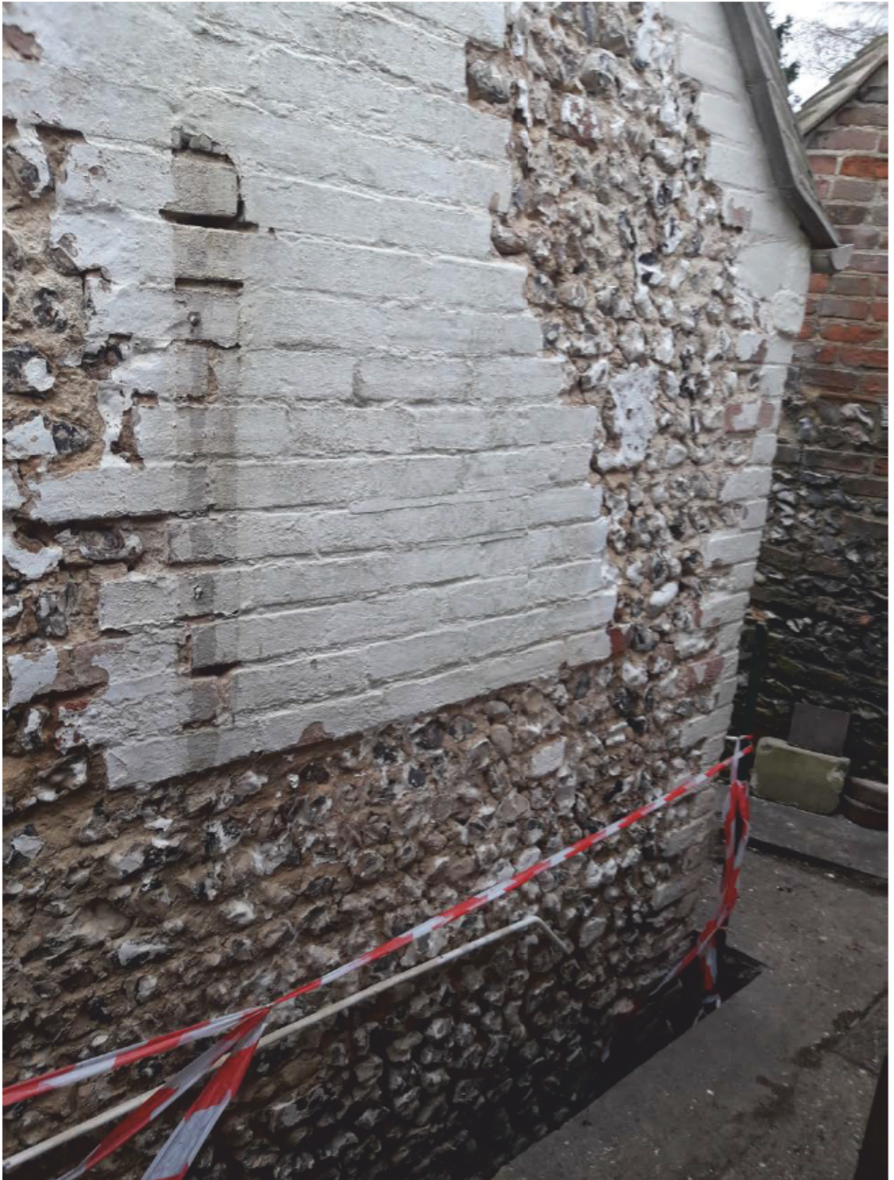
Plate 9: South end of the side (west) elevation of the Old Bakery, looking south-east (photograph provided by George Roberts)
