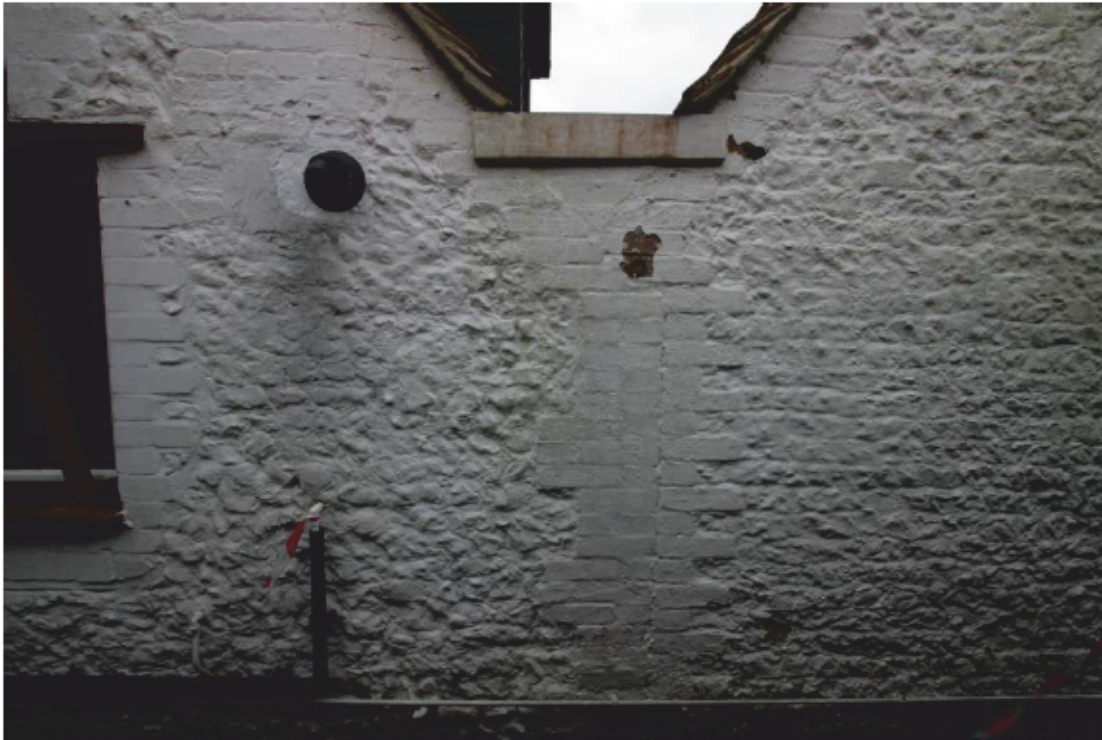
Plate 5: West elevation showing straight joint between Utility Room and Kitchen, looking east (D3 005)
