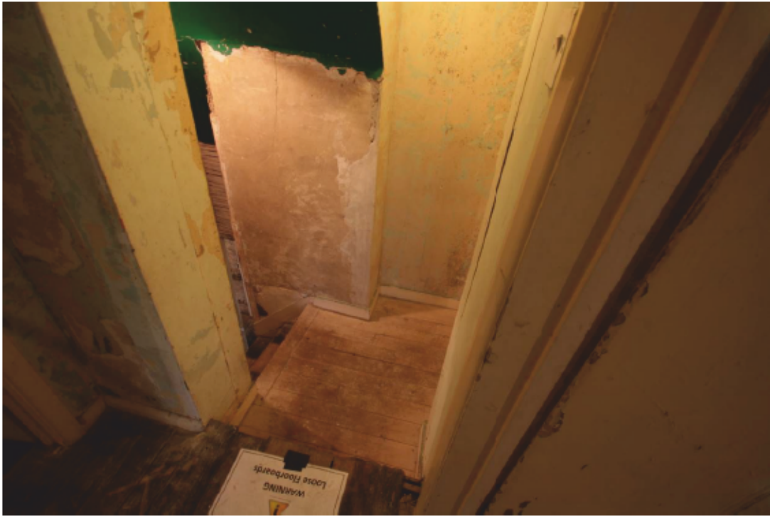
Plate 40: First floor Landing, looking south (D2 017)
