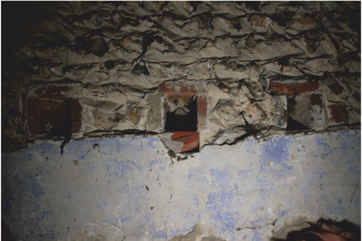
Plate 31: Joist sockets in north wall of roof space above Study, looking north (D1 018)
