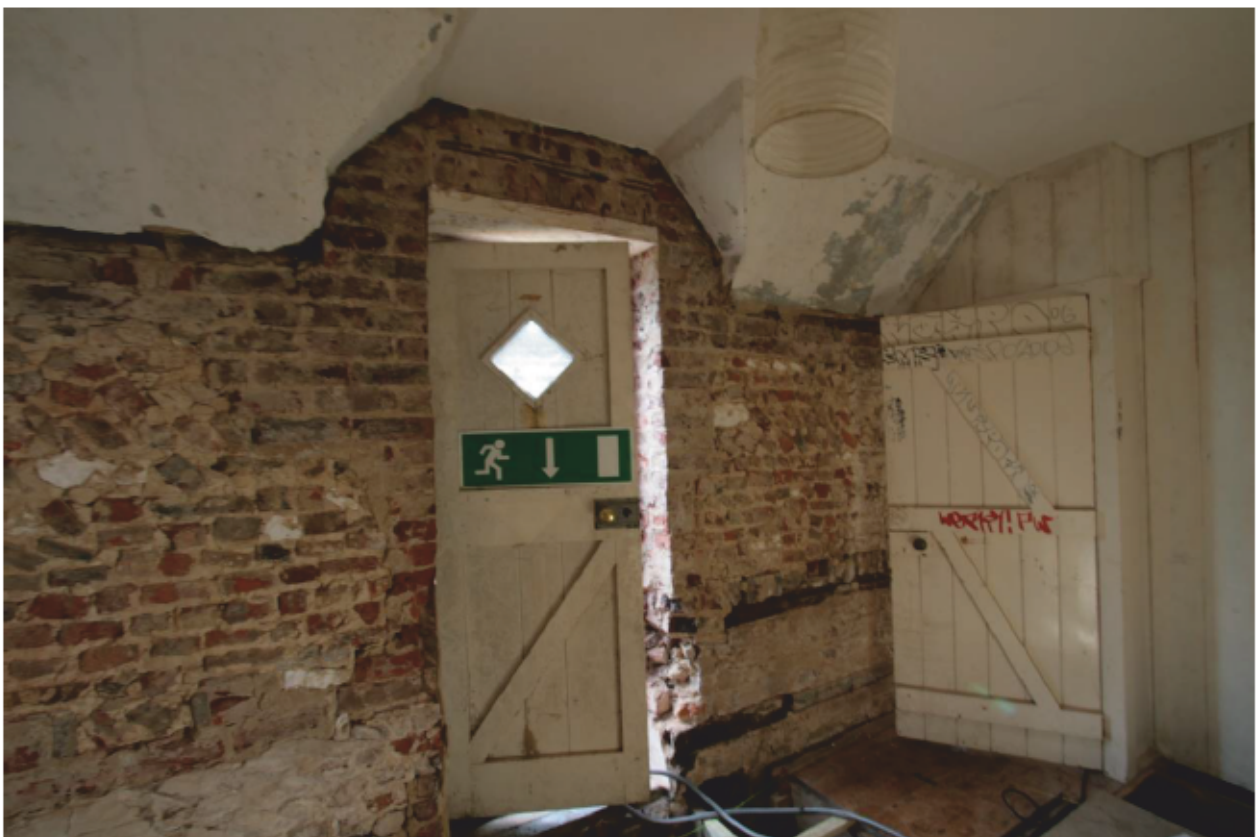
Plate 28: South (left) and west (right) walls of the Study, looking south-west (D1 005)
