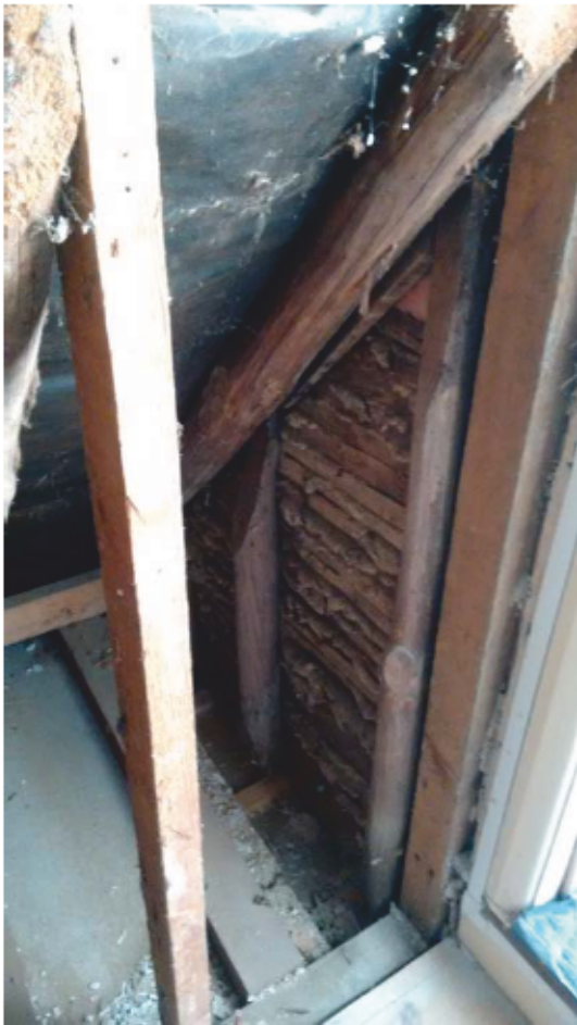
Plate 41: South and west walls of first floor Landing, looking south-west (photograph provided by George Roberts)
