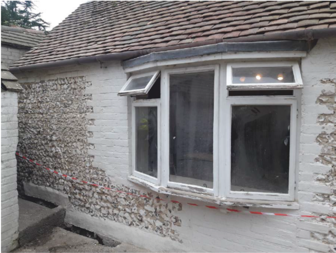
Plate 10: South elevation of the Kitchen, looking north (photograph provided by George Roberts)
