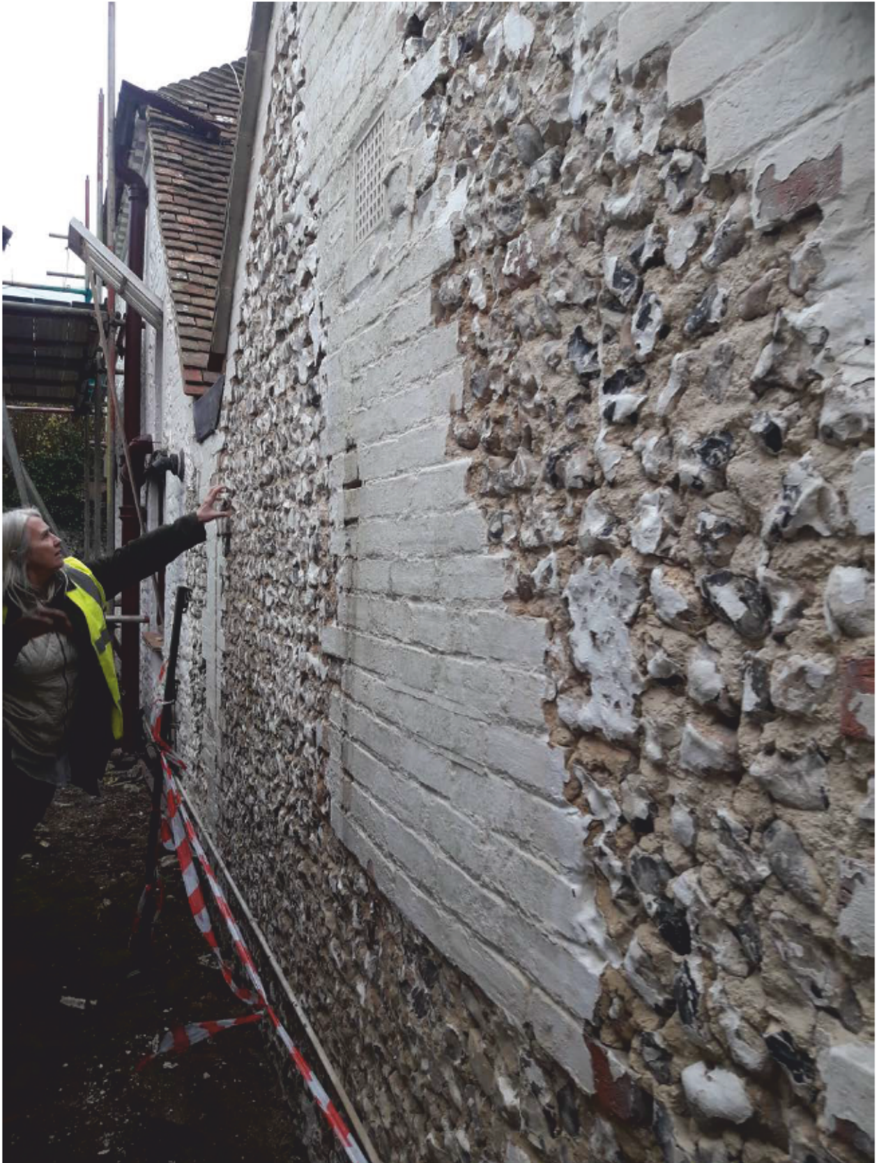
Plate 8: Side (west) elevations of the Old Bakery, looking north-east (photograph provided by George Roberts)
