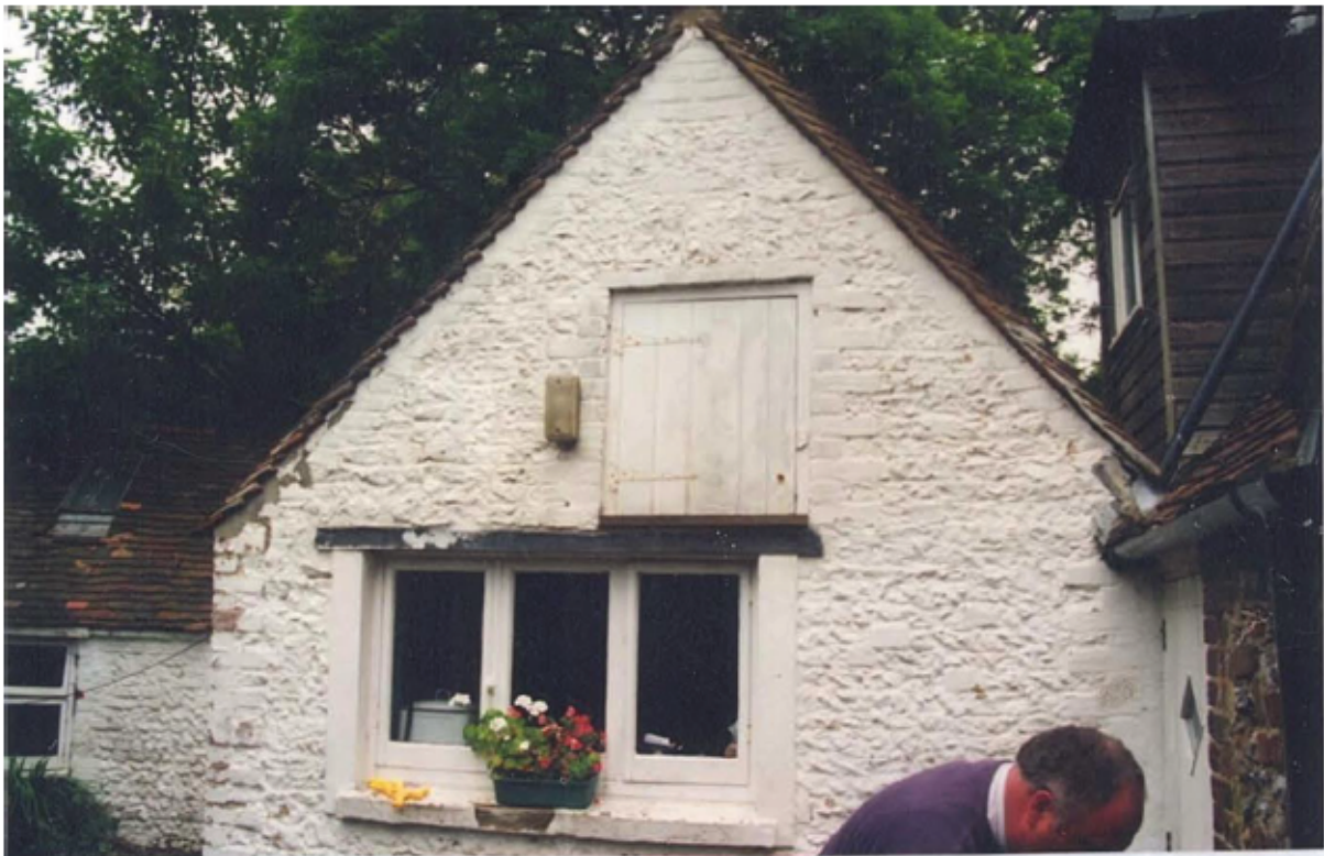
Historic Plate 37 Photograph taken in May 2000 of the former bakehouse (now Kitchen) extension at the Old Bakery, looking west (© NT Wisley)
