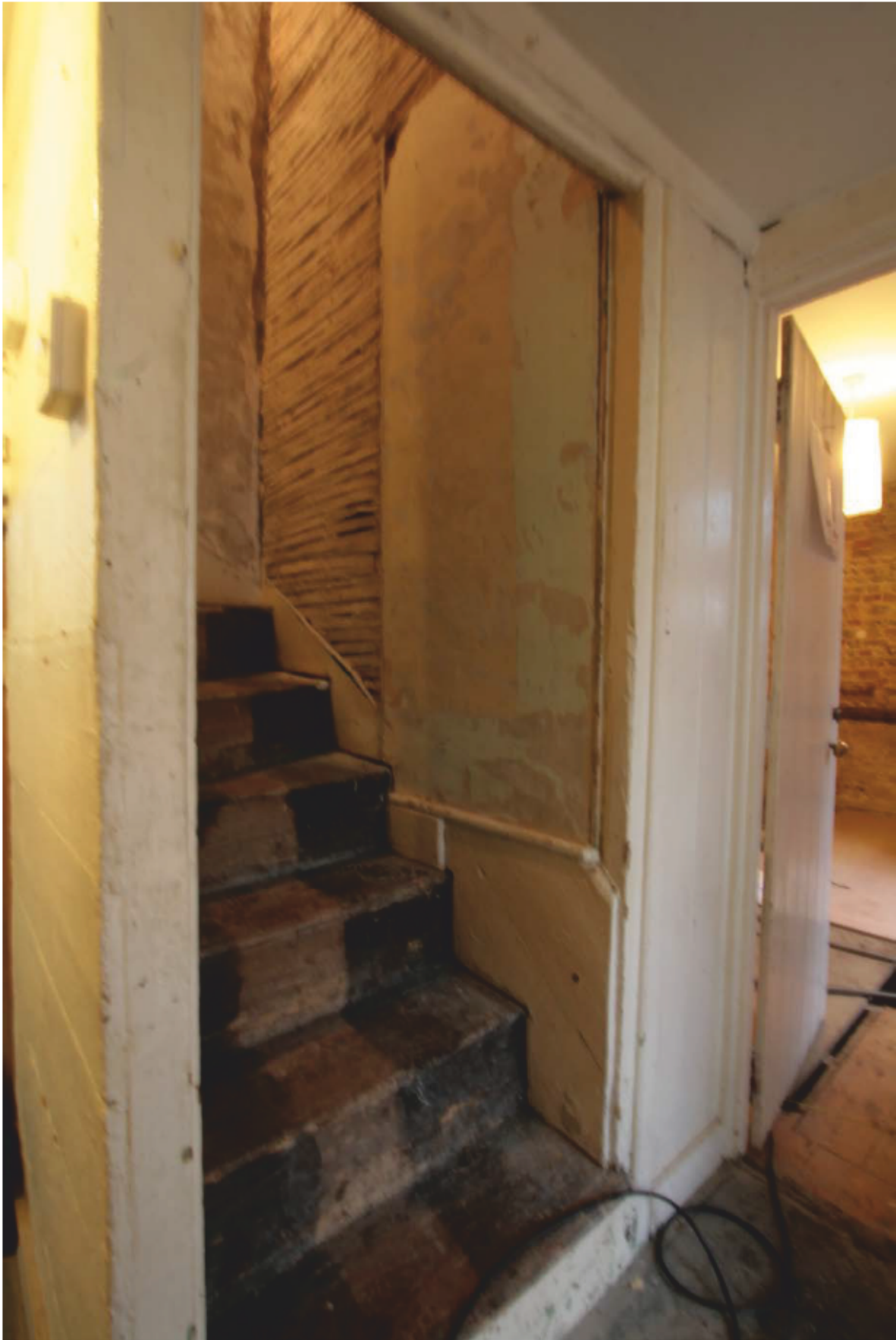
Plate 35: Ground floor hall showing blocked doorway and Study (right), looking north-east (D1 025)
