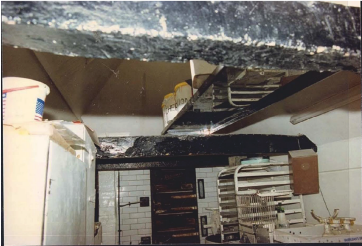
Historic Plate 26 Photograph taken by Sara Squires in September 1991 of the oven in the south elevation of the bakery building at the Old Bakery, looking south (© NT Wisley)
