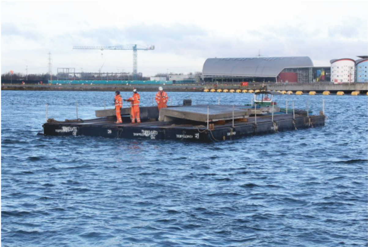
Plate 45: Floating platform/barge used to transfer sections of Dolphin 7's cap to Topbond's Compound, looking north (CIY17 D2 9)
