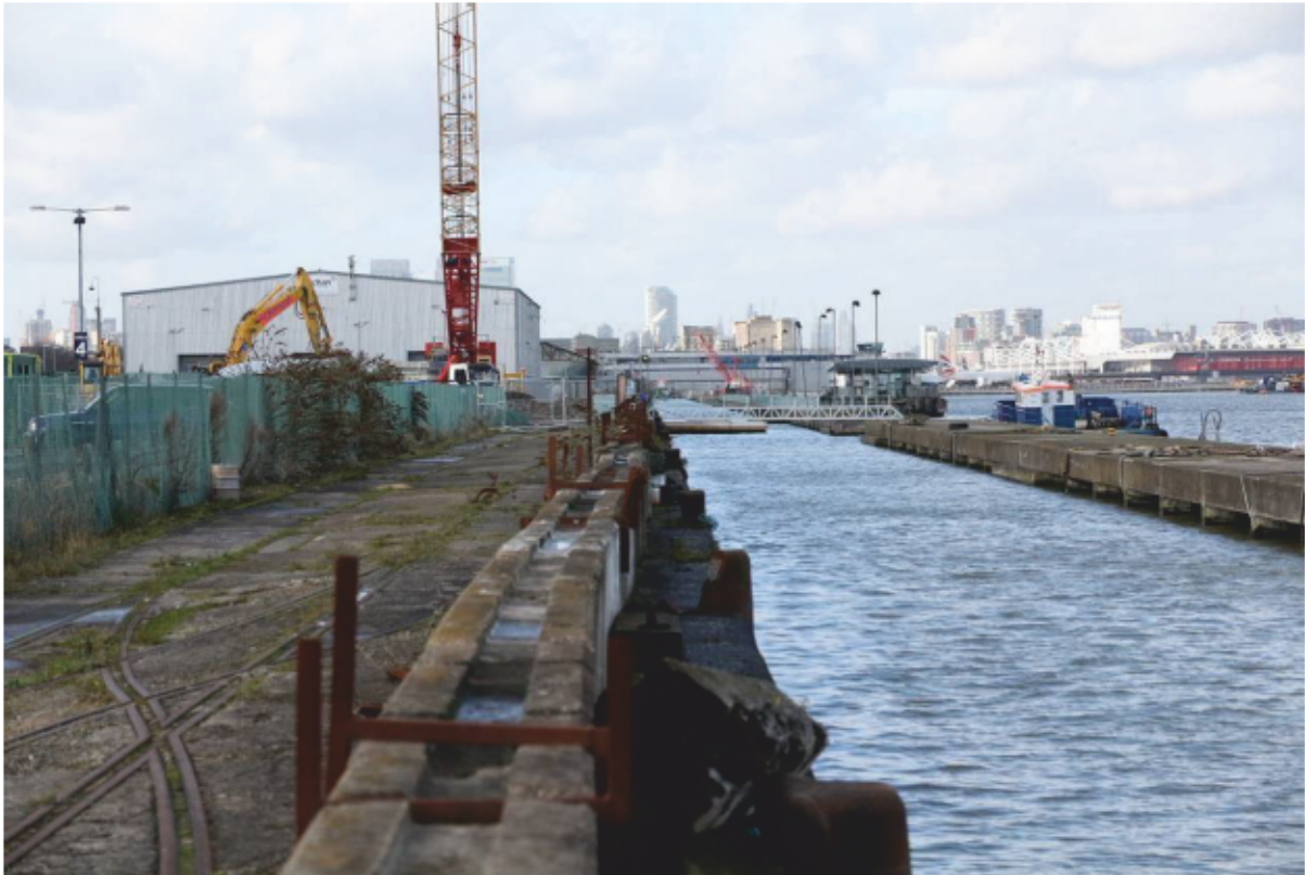
Plate 13: Railway tracks and mooring posts along the east end of the south side of King George V Dock with the Dolphins 2 and 3 to the right, looking west (CIY17 D5 48)
