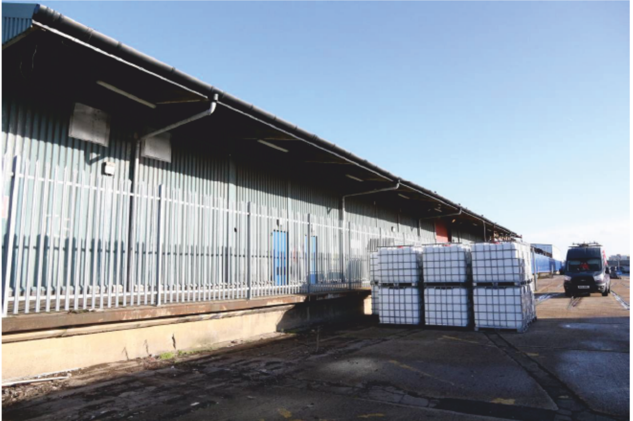
Plate 23: Original steel frame of Transit Shed 4 re-clad on the south side of King George V Dock, looking north-east (CIY17 D5 12)
