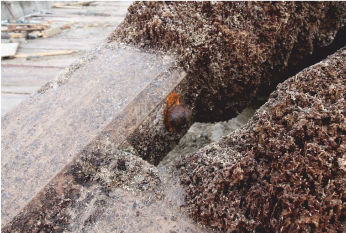
Plate 63: Detail of steel bolt, possibly used to secure timber facing to Dolphin 7, looking east (CIY17 D3 29)
