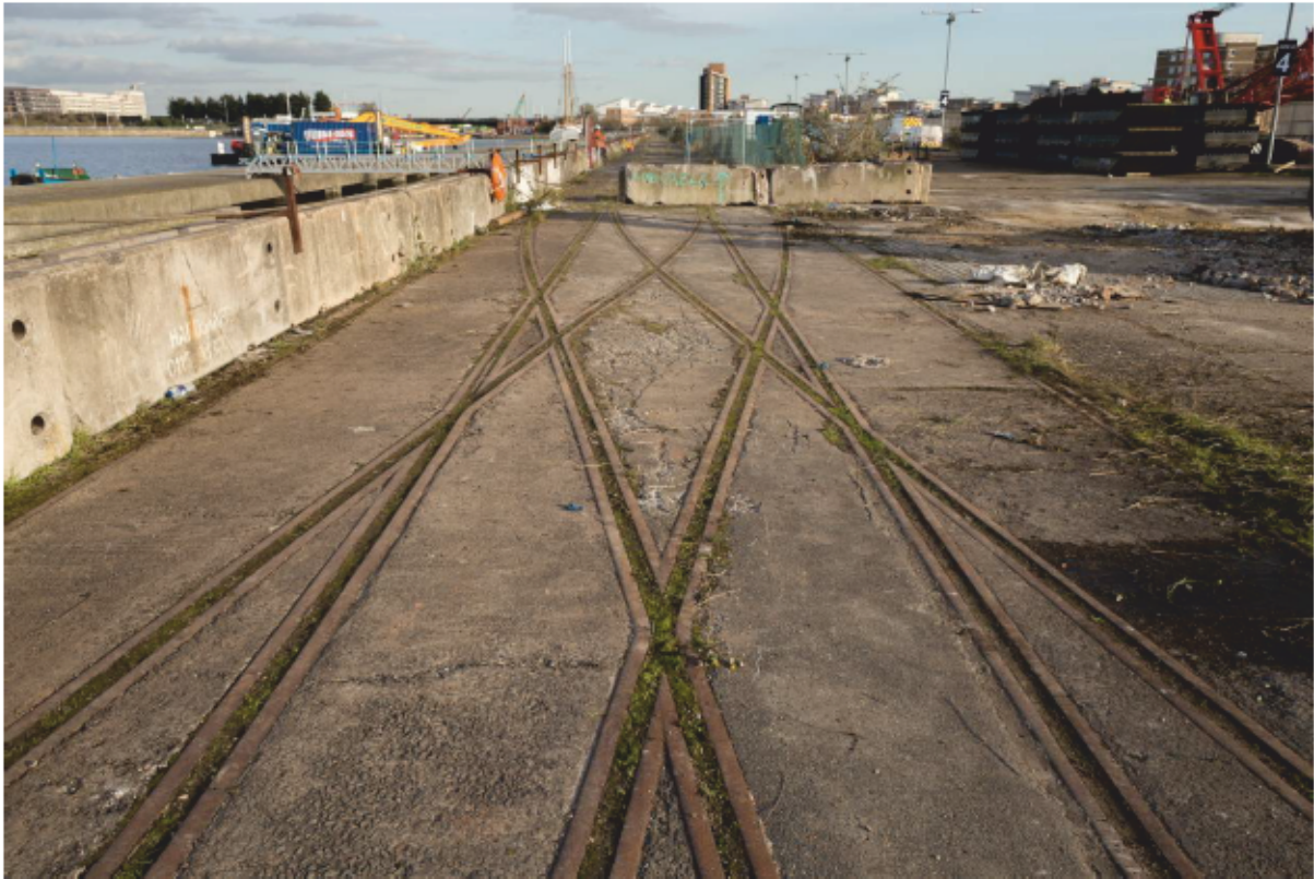
Plate 19: Railway line crossover towards the east end of south quay of King George V Dock originally to the north of the gap between former Transit Sheds 2 and 3, looking east (CIY17 D100 033)
