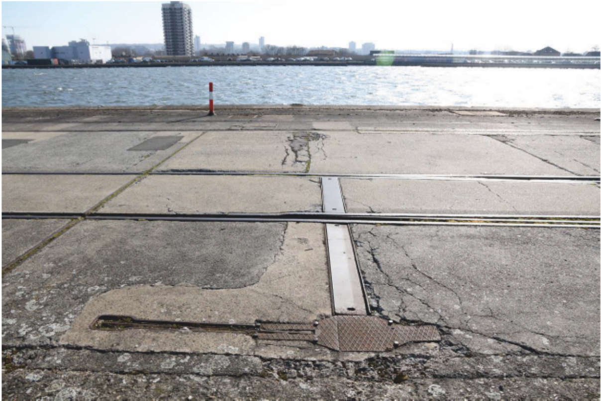
Plate 85: Manual railway track switch along north quayside of King George V Dock, looking south
