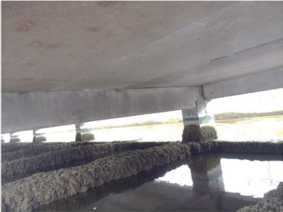
Historic Plate 26: Photograph taken in 2016 of the underside of Dolphin 7 by Constructex following the lowering of the water in King George V Dock, looking south-east
