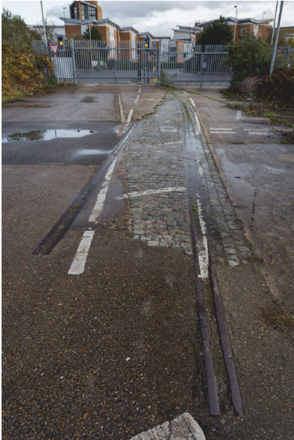
Plate 31: Patch of granite setts and railway lines at the east end of the south side of King George V Dock, looking east (CIY17 F100 048)
