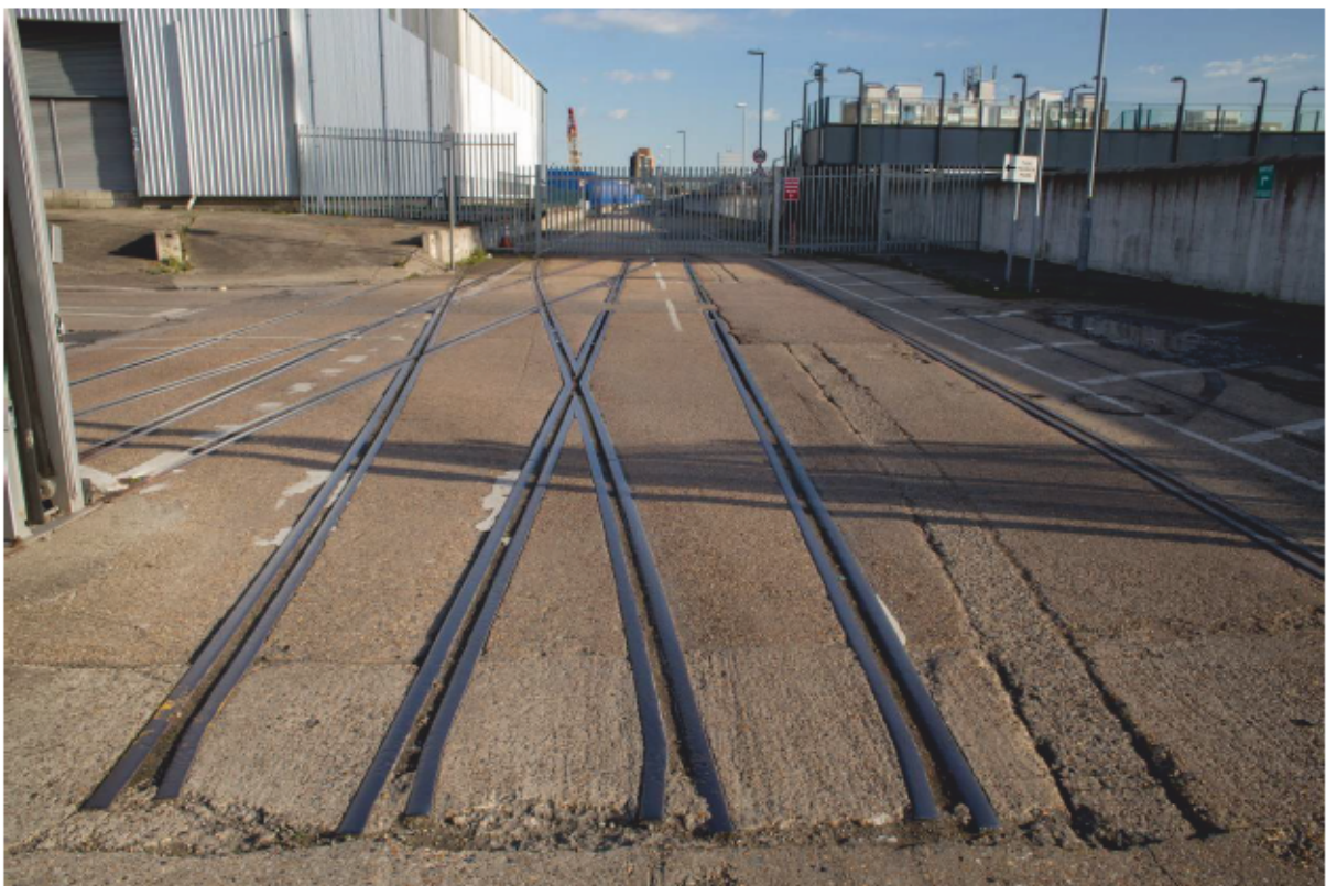
Plate 30: Railway line crossover to the south of the gap between former Transit Sheds 3 and 4 on the south side of King George V Dock, looking east (CIY17 D100 025)
