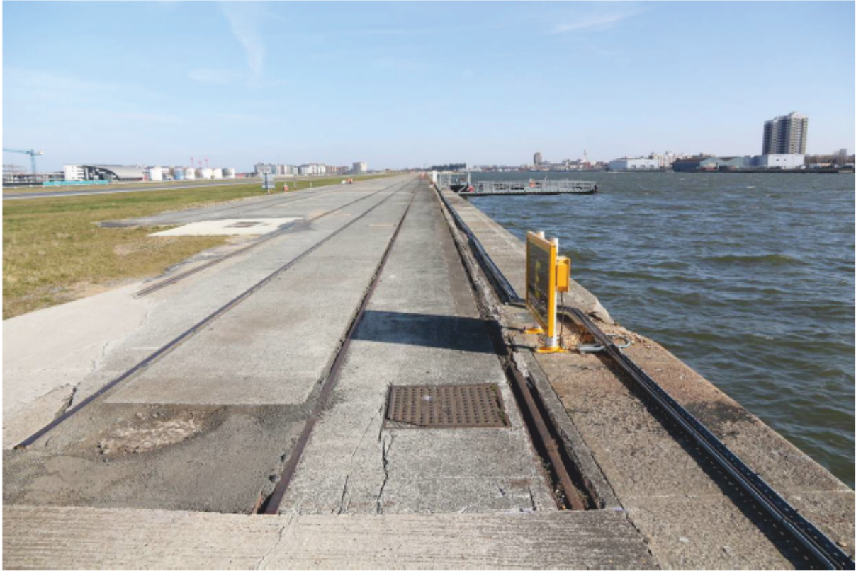
Plate 69: Railway tracks and coping stones along north quayside of King George V Dock, looking east
