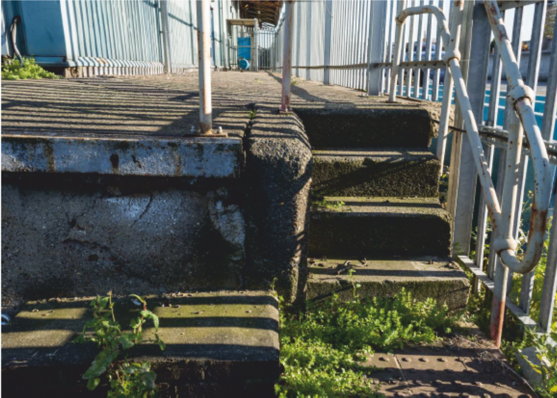
Plate 37: Stairs at the east end of the platform to the south of Transit Shed 4, looking east (CIY17 D100 018)
