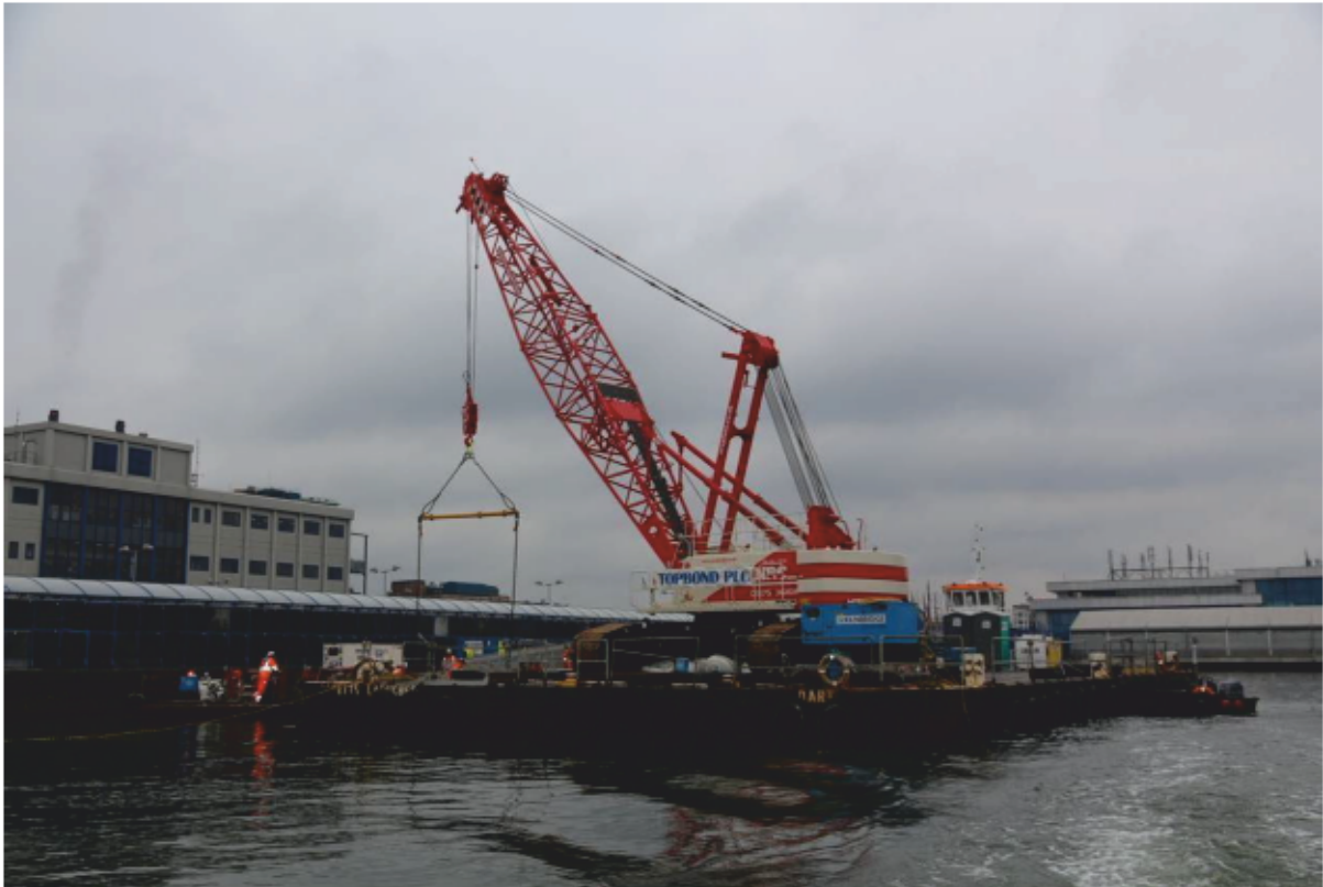
Plate 43: Waterborne crane used to cradle sections of Dolphin 7, looking south-west (CIY17 D3 122)
