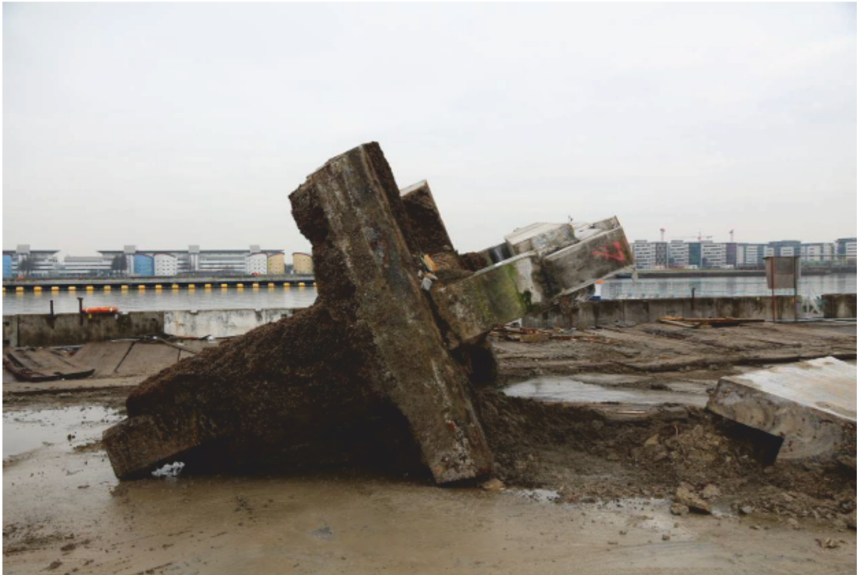
Plate 61: Modern cap and original Dolphin 7 structure in Topbond Compound, looking north (CIY17 D3 3)
