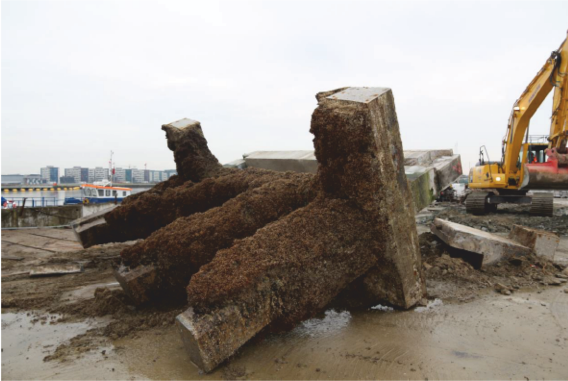
Plate 57: Aquatic growth on below water Dolphin 7 brace, looking north (CIY17 D3 5)
