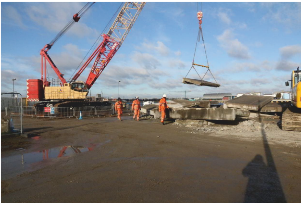
Plate 46: Lifting Dolphin 7's cap sections from the floating platform into Topbond's Compound, looking north (CIY17 D2 13)
