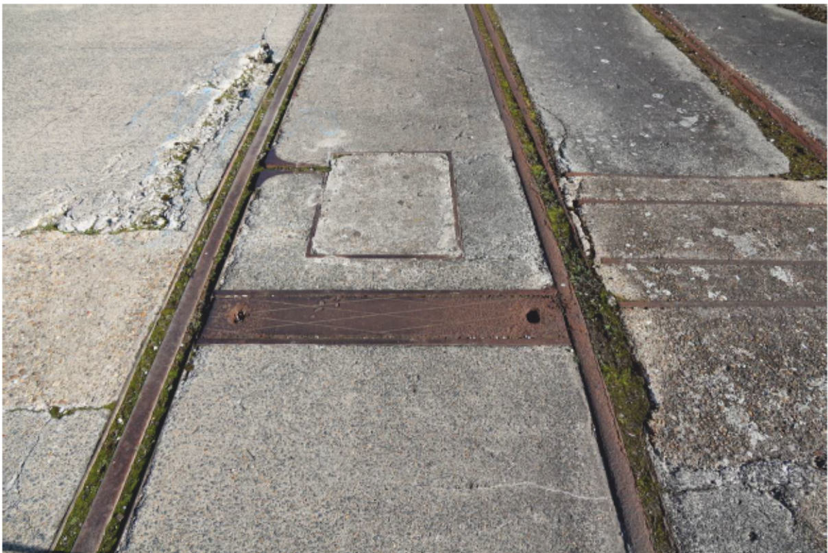
Plate 82: Brace bar on railway track along north quayside of King George V Dock, looking east
