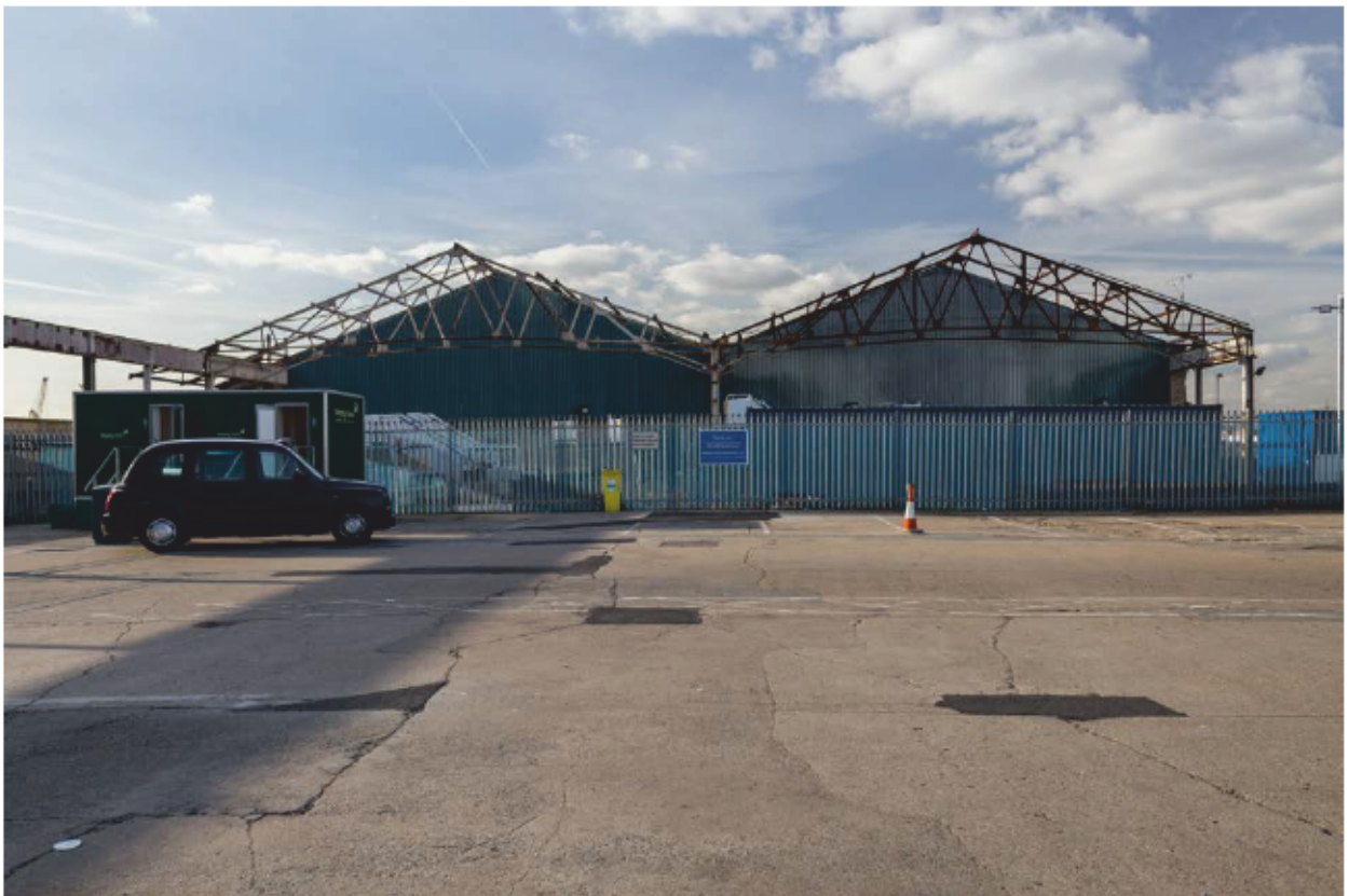
Plate 24: Steel angle roof trusses of Transit-Shed 4 on the south side of King George V Dock, looking west (CIY17 D100 026)
