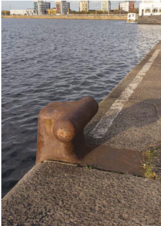
Plate 15: Mooring post on the east side of King George V Dock, looking north (CIY17 D100 039)
