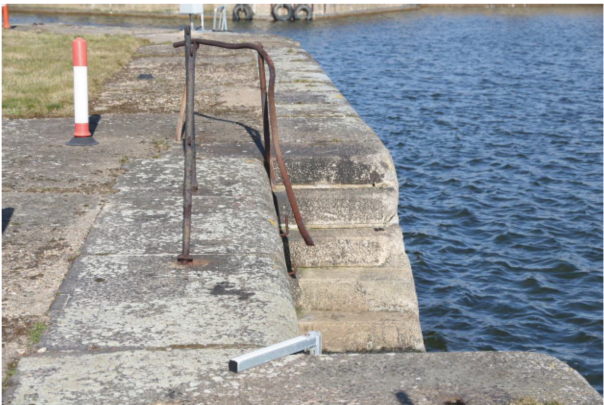
Plate 76: Coping stones and stairs at east end of north quayside of King George V Dock, looking north-east
