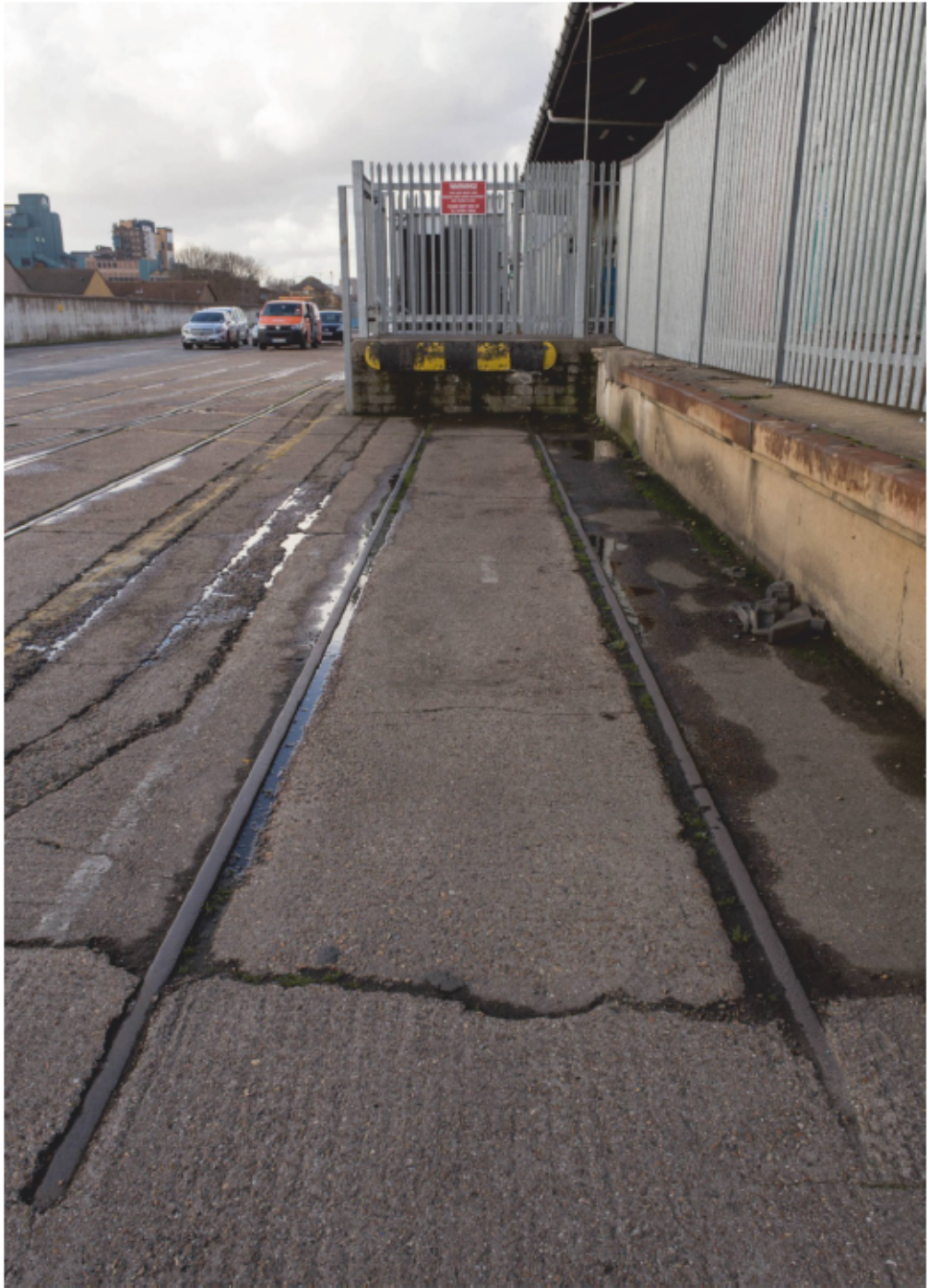
Plate 32: Later extension to the platform over the railway line to the south of former Transit Shed 4, looking west (CIY17 D101 051)
