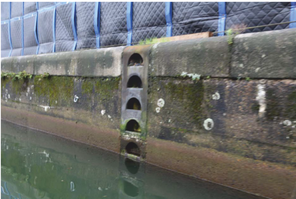
Plate 18: Coping stones and steps along the west end of the south quay of King George V Dock, looking south-east (CIY17 D3 87)
