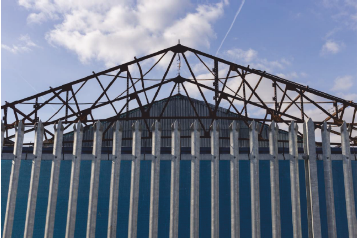
Plate 25: Steel angle roof trusses of Transit-Shed 4 on the south side of King George V Dock, looking west (CIY17 D100 027)
