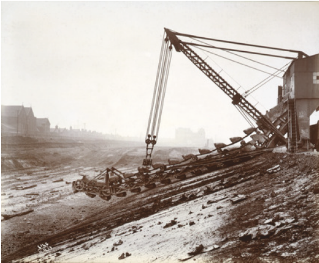
Historic Plate 1: Photograph taken on 11 September 1913 showing the excavation of King George V Dock using a steam-powered excavator (© PLA collection/Museum of London)
