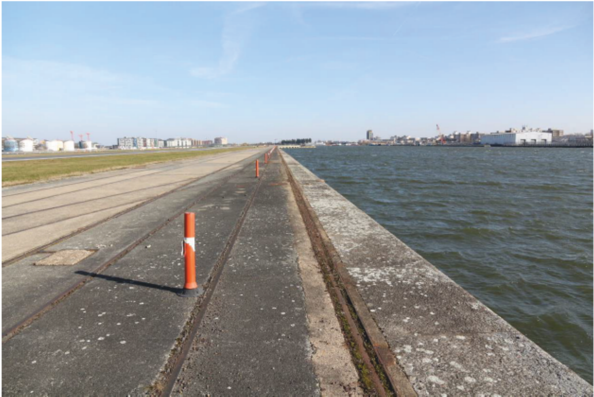
Plate 71: Railway tracks and coping stones along north quayside of King George V Dock, looking east
