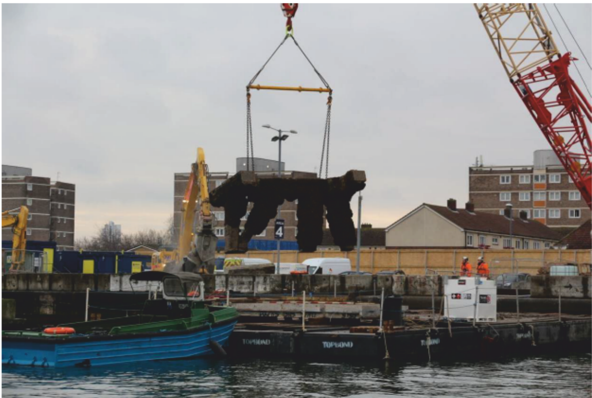
Plate 58: Lifting Dolphin 7 brace from King George V Dock into Topbond's Compound, looking south (CIY17 D3 148)
