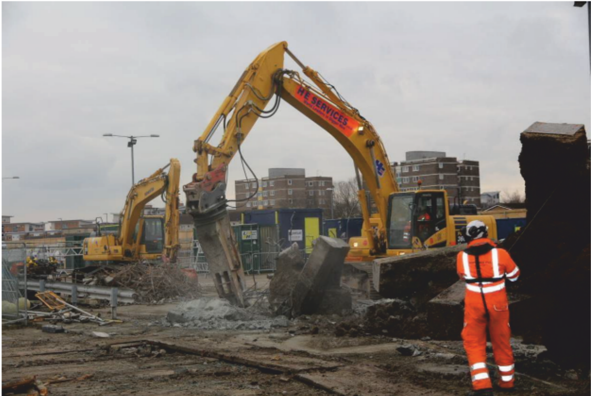
Plate 59: Demolition and separation of steel rebars and concrete from Dolphin 7's brace sections, looking east (CIY17 D3 160)
