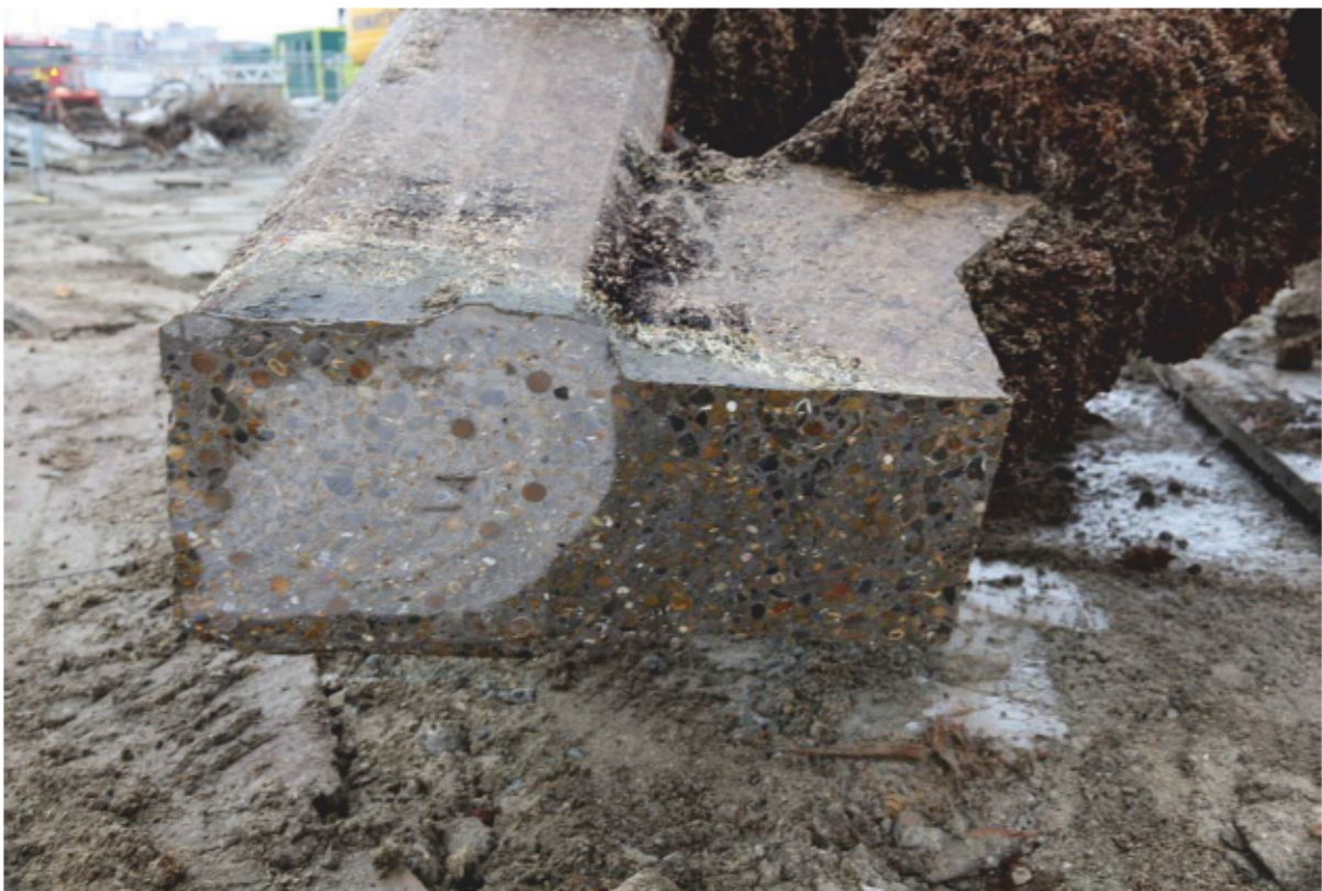
Plate 62: Cut section of Dolphin braced frame showing steel reinforcements, looking east (CIY17 D3 9)
