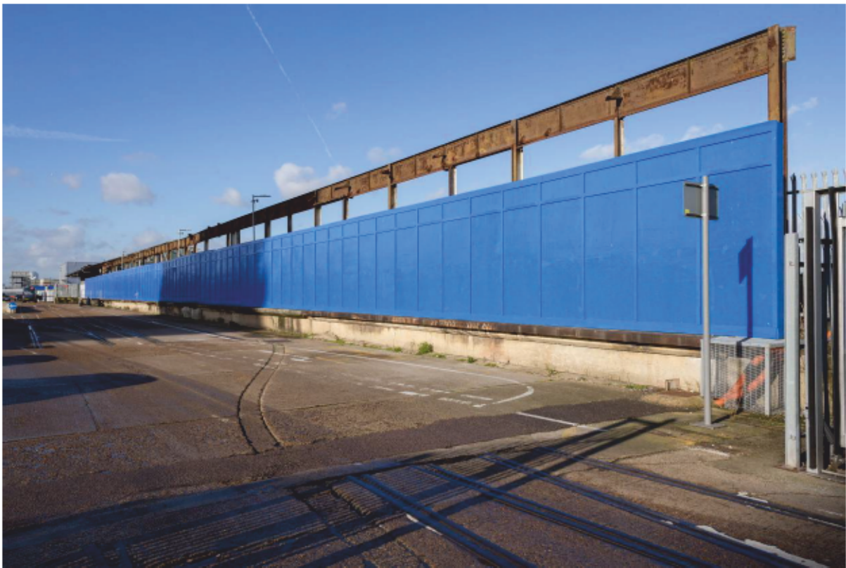
Plate 26: Platform and south steel wall frame of Transit-Shed 4 on the south side of King George V Dock, looking north-west (CIY17 D101 003)
