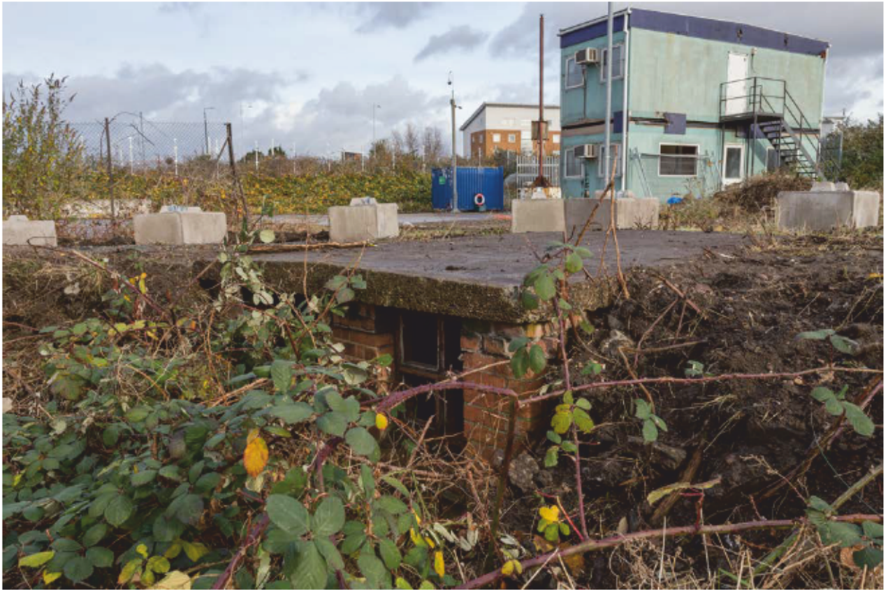
Plate 41: Brick building in the south-east corner of the Site, looking north-east (CIY17 D100 046)
