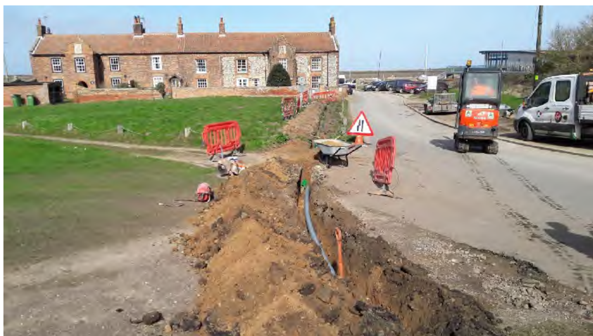
Plate 4 Cable-trench in the vicinity of Brancaster Staithe Green, with cable-pipe inserted, looking north towards Activity Centre,
