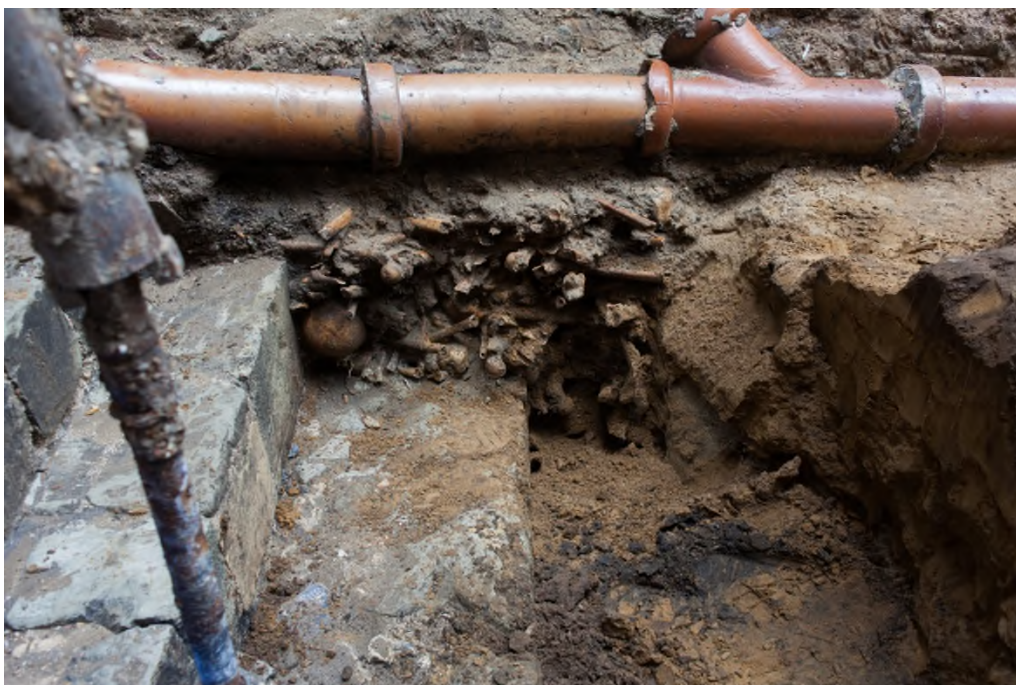
Plate 4: North facing view of channel within construction cut for limecrete raft foundation [233]
