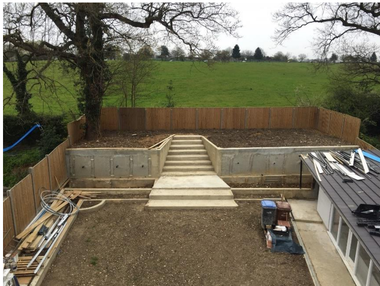
Plate 1: East facing view of recently constructed terrace, showing retaining wall and steps.
