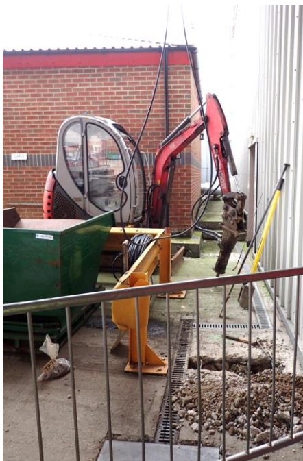
Plate 11a: Location of Borehole 7 against the Process Raw Materials building. View to NW.
