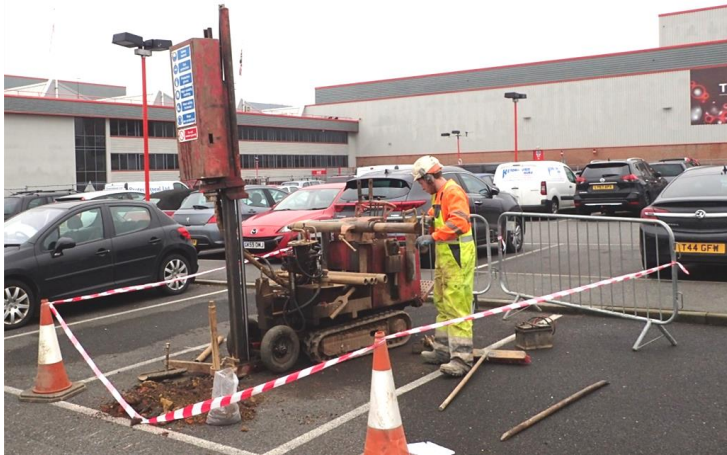
Plate 10: Location of Borehole 6 in the car park in the north-west area of the site, west of the Process Raw Materials building. View to the east.
