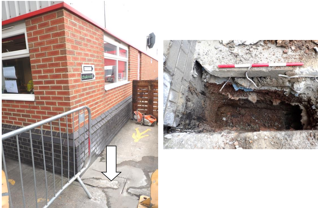
Plate 2a & 2b: Plate 2a of Test Pit 4 (left), view to the NE (concrete pad cut in preparation for excavation marked by arrow). Plate 2b shows made ground layers [7] and [8] below the concrete. View to SE, scale 0.5m.
