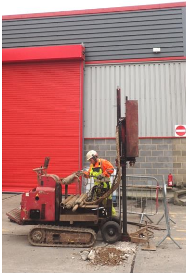
Plate 8a: Location of Borehole 4 at the south-west end of the Canning Flex Warehouse adjacent to Test Pit 5. View to NE.
