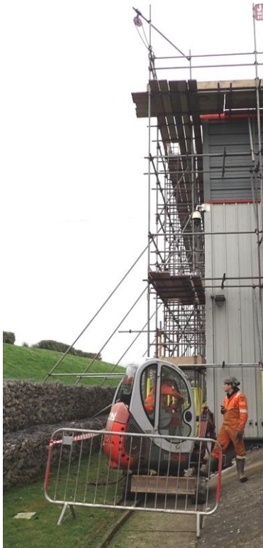
Plate 4a: View to NE of Test Pit 6 against the Process Raw Materials Building
