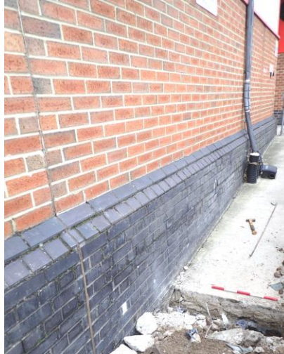
Plate 3a: General view of Test Pit 5 located against the exterior south wall of the Canning flex Warehouse. View to the SE, scale 0.5m
