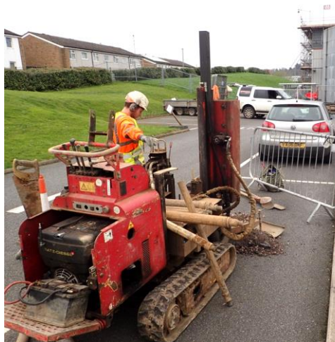
Plate 9a: Location of Borehole 5 in the car in the north-west corner of the site, west of the Process Raw Materials building. View to NE.
