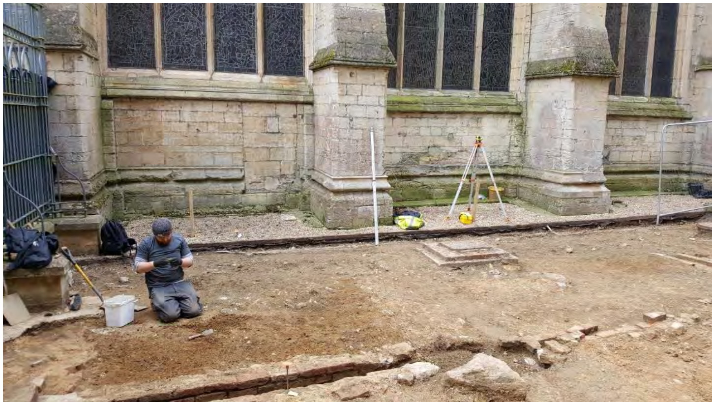
Plate 11: Work progressing in the eastern half of site, showing blocked up doorway in the north wall of the Presbytery (centre left beneath window), view south.
