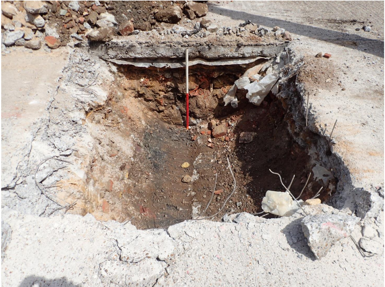
Plate 1: Test Pit 2, Modern material overlying a north-south concrete capped service, looking north (1m scale).
