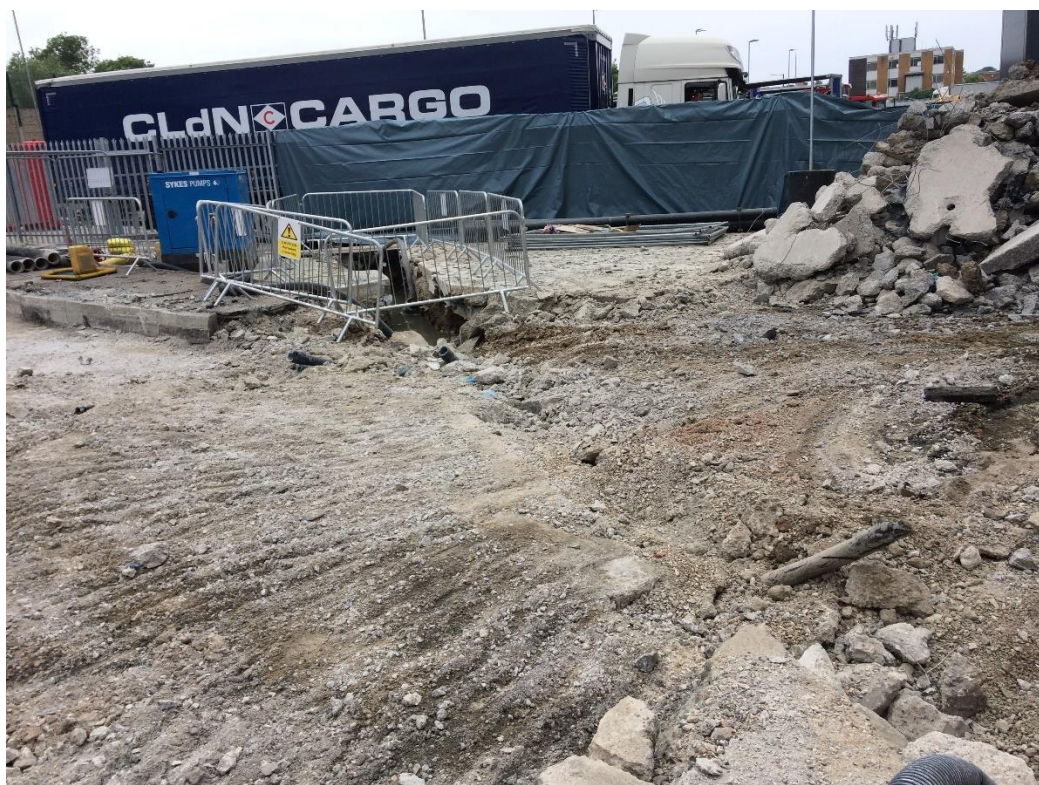
Plate 4: Central part of the site after removal of concrete slab, looking north-west.
