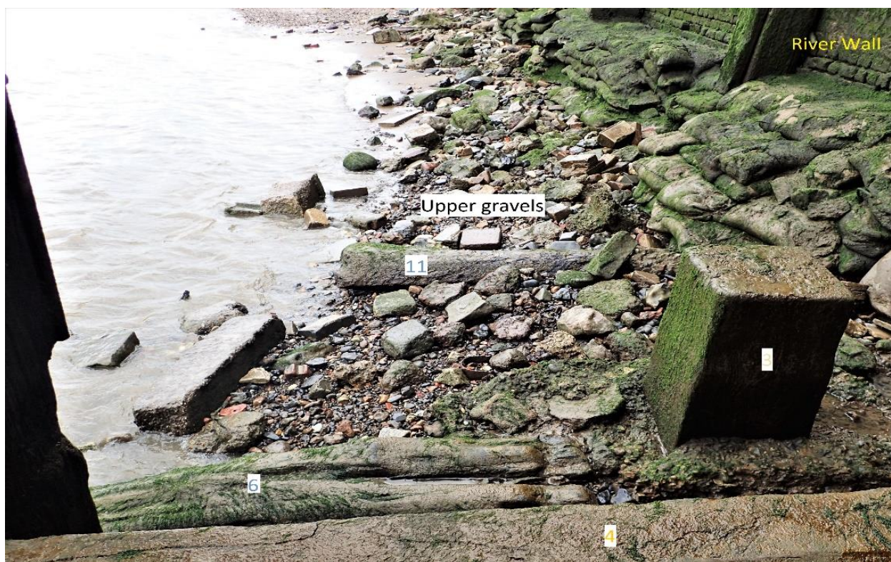
Plate 3: Phase 2 Grid iron structure, consisting of two horizontal land-tie timbers [6 & 11]. The large square timber to the right is part of the Phase 3 river wall revetment. View to east.
