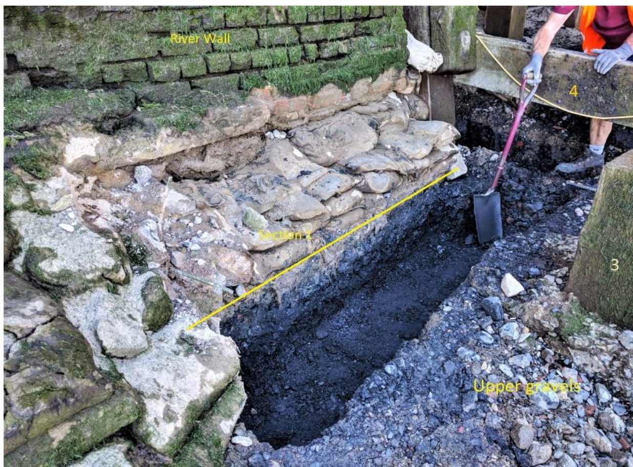
Plate 5: Section 1 showing modern upper gravels and lower, dark grey lower gravels [1] against the River wall. View to south-west.
