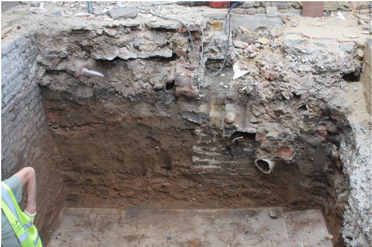
Plate 4: Excavation area showing rear (north-east) wall of closet wing [50] (left) and brick silt trap [44] towards the left side of the section (Section 5), looking north-west
