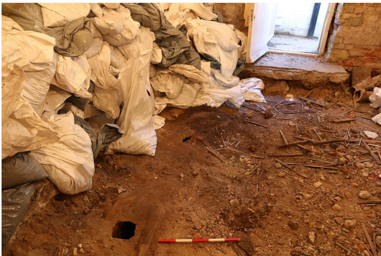
Plate 14: Brick drain under front basement room, looking south-west towards the front lightwell
