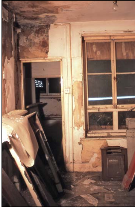
Plate 18: General view of room SNFo10, showing poor condition of building
