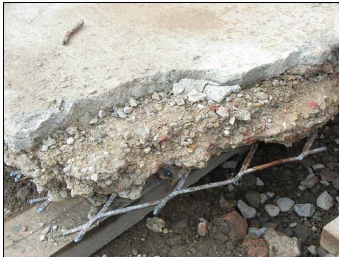
Plate 21: cross-section of concrete sample
