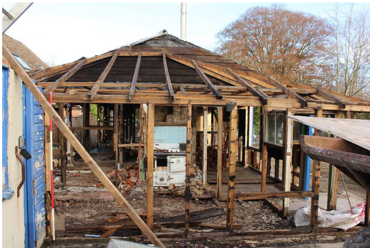
Plate 7: North-east facing view of south-west facing frontage, showing modern extension. 2m scale
