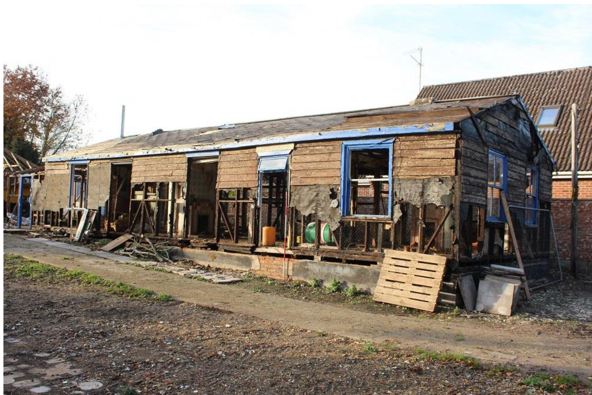
Plate 5: North-west facing view of structure, showing south-east and north-east facing frontage. 2m scale
