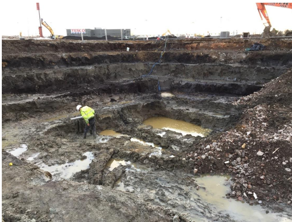
Plate 11: Excavation Area 2 looking south. Stepped trench excavated through a sequence of alluvium and peat deposits to the natural sand/gravel
