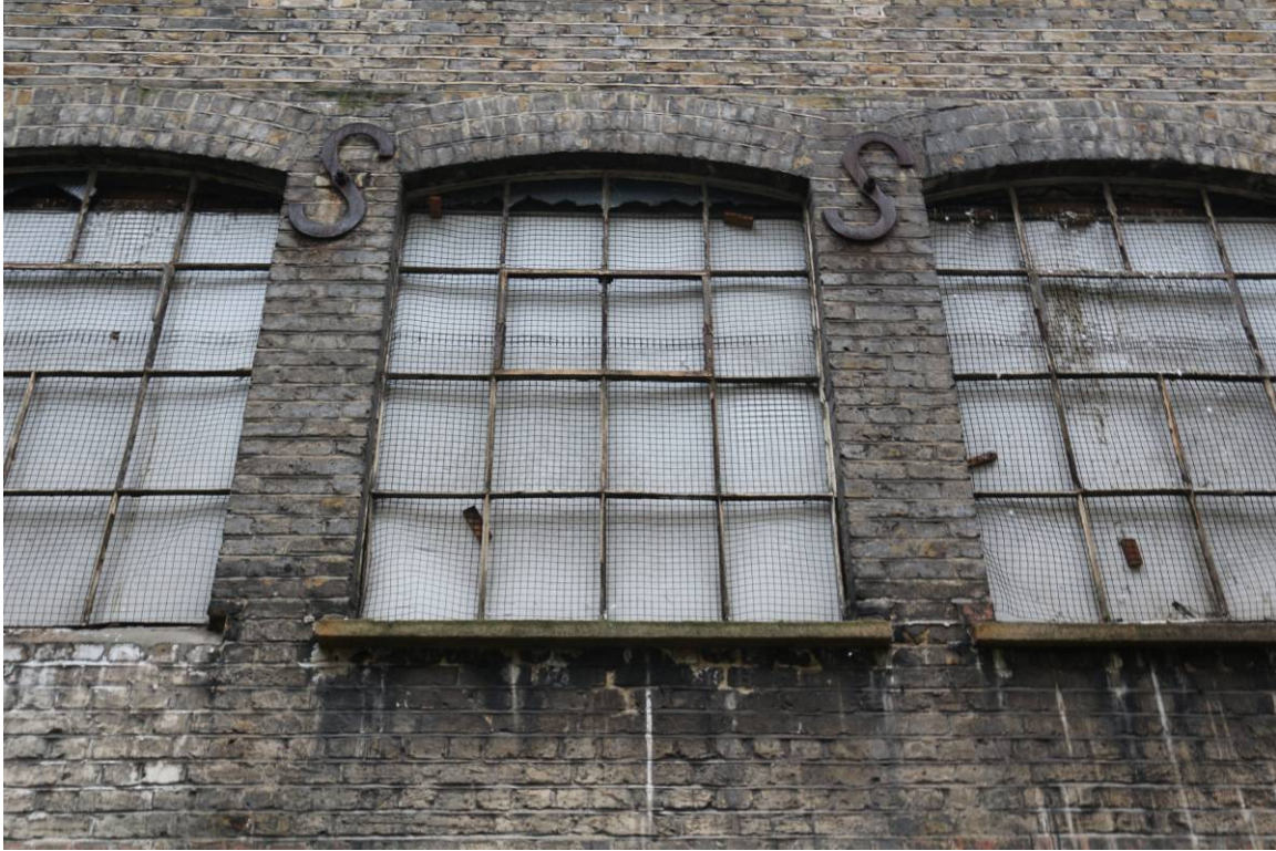
Plate 5 Detail of S-shaped tie-bar ends at upper ground floor level, looking north
