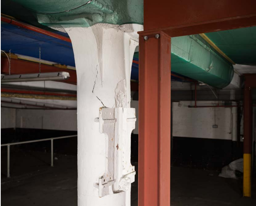
Plate 17b Lower ground floor level, detail of original column in western bays, looking west
