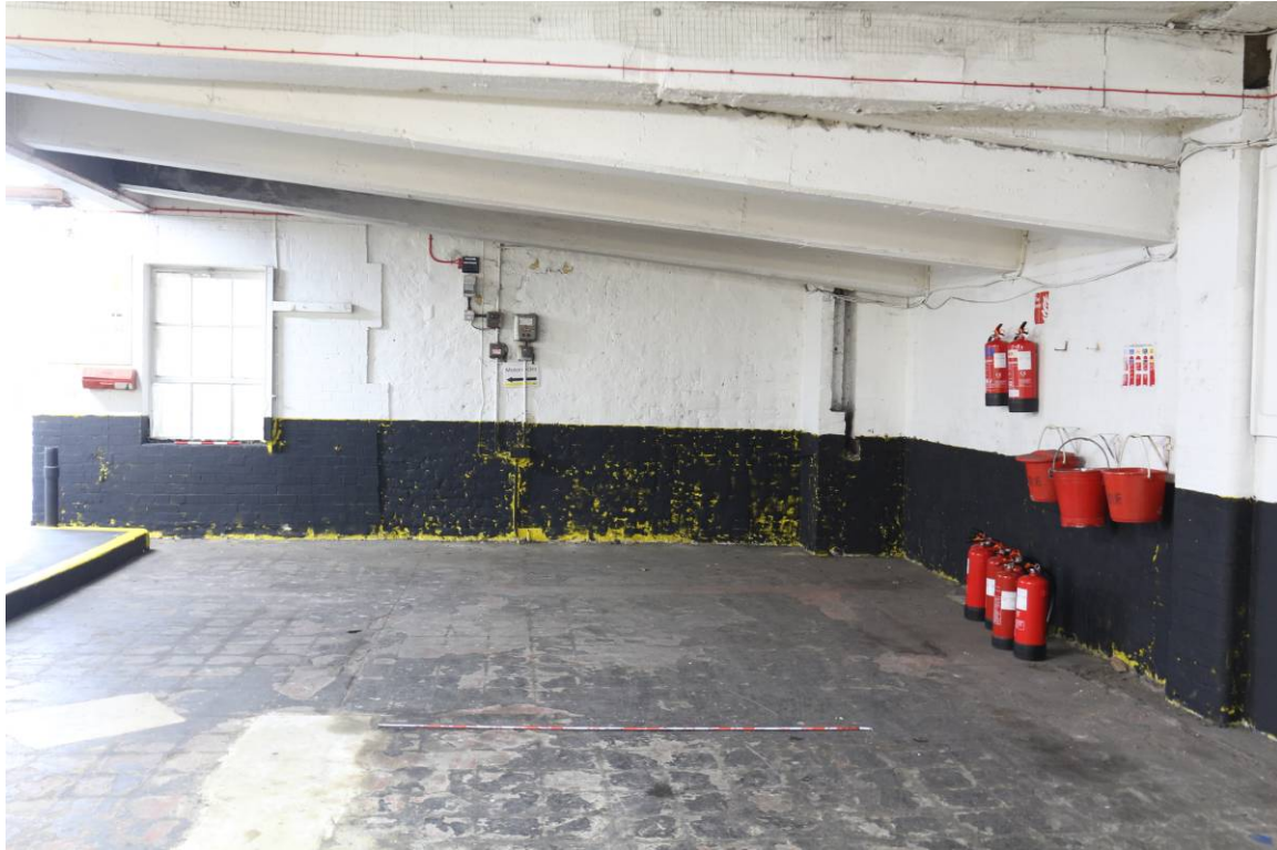
Plate 23 Upper ground floor level, central bays, tiled floor next to entrance and below ramp
