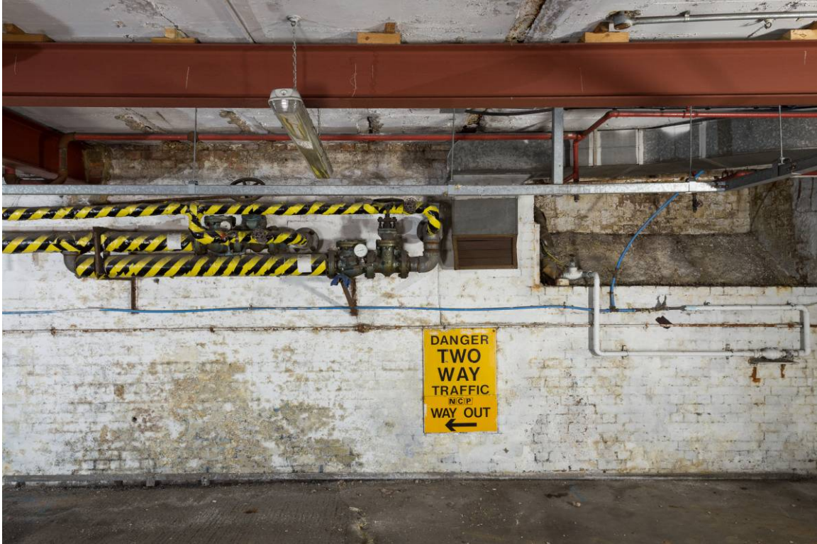
Plate 16 Lower ground floor level, central bays, water inlet to sprinkler system
