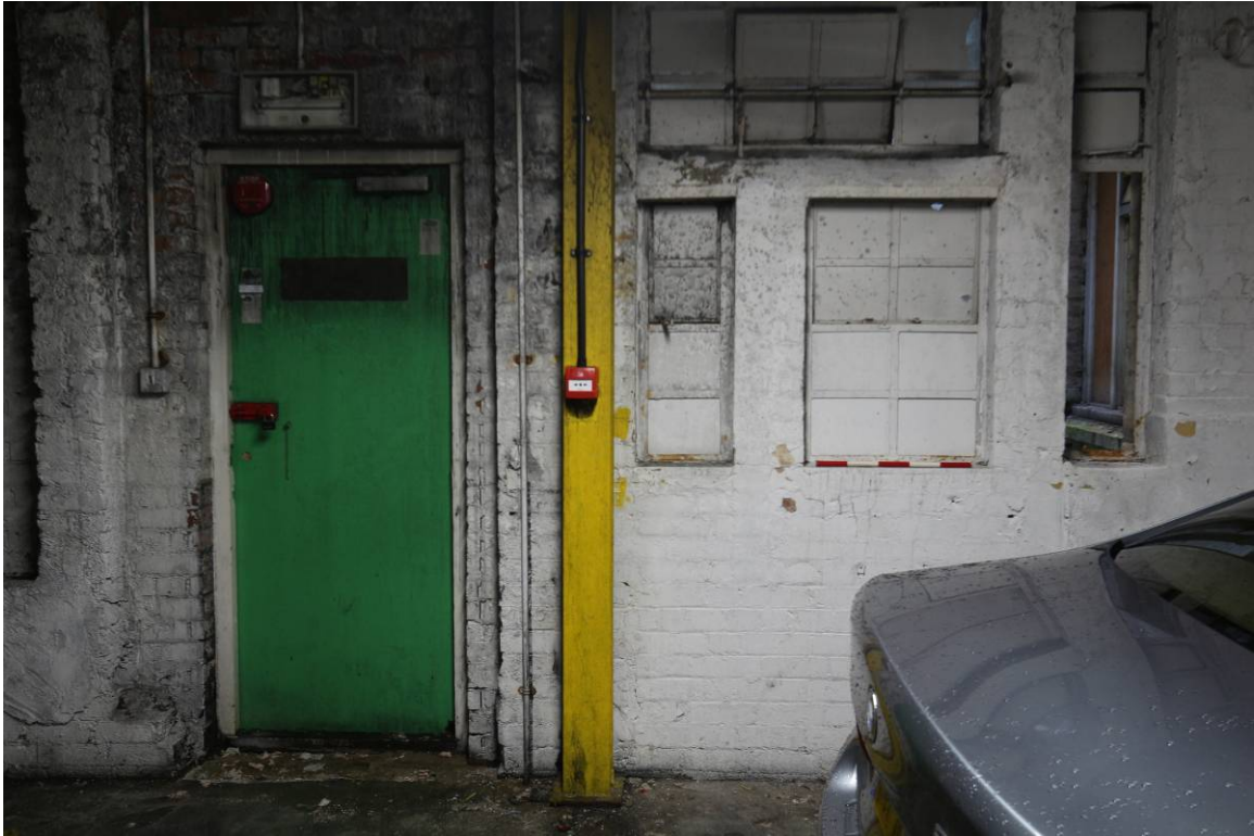
Plate 26b Upper ground floor level, western bays, looking north to north-west stairwell
