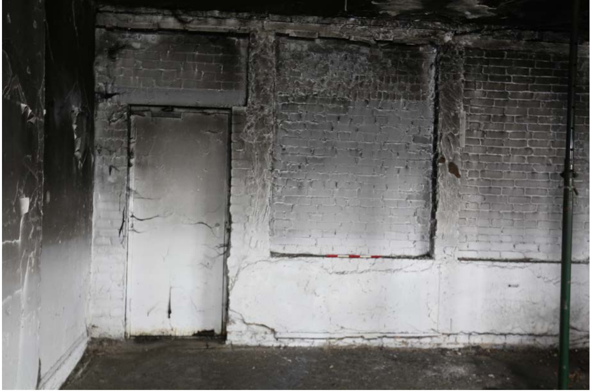
Plate 26a Upper ground floor level, western bays, looking west at the south end of the western elevation
