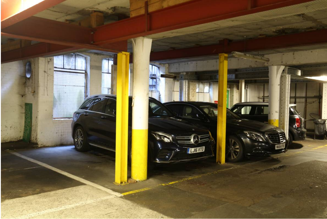
Plate 20 Upper ground floor level, eastern bays, windows into light well, looking south-east
