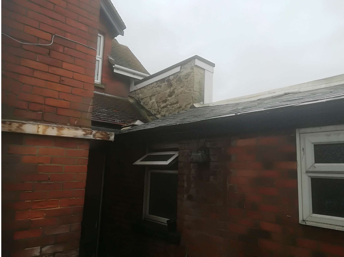
Plate 1. Recessed external northern end of the eastern elevation of the building. Part of a masonry wall is visible adjacent to the upper storey and a the men's toilets in the foreground. No scale.
