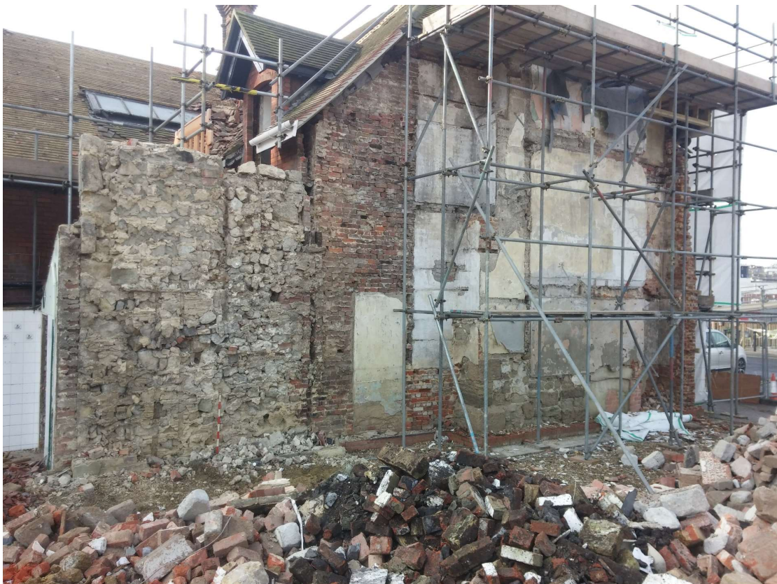
Plate 6. Exterior northern elevation of the White Hart Inn and limestone infill wall following removal of cladding sheet cladding. Scale 1m.
