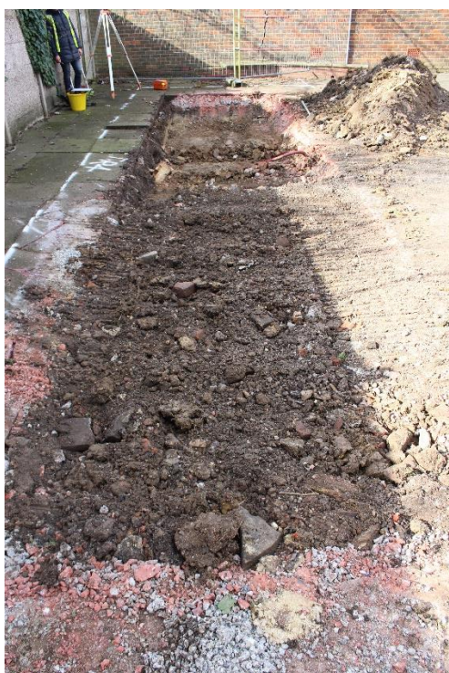
Plate 6: West view of Trench 4 shows eastern half of trench unexcavated due to unexpected buried live services seen in Plate 5.
