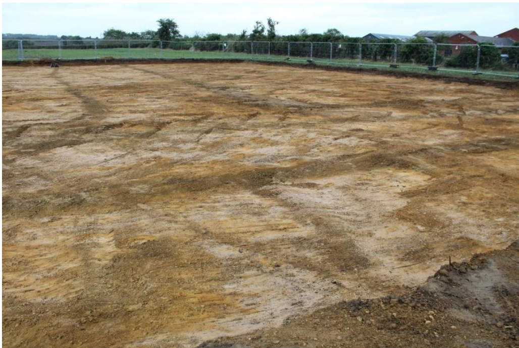
Plate 7. Overview shot showing the key romano-british features at the centre of Area B, looking northwest.
